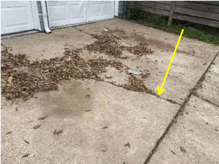
Uneven driveway -trip hazard
