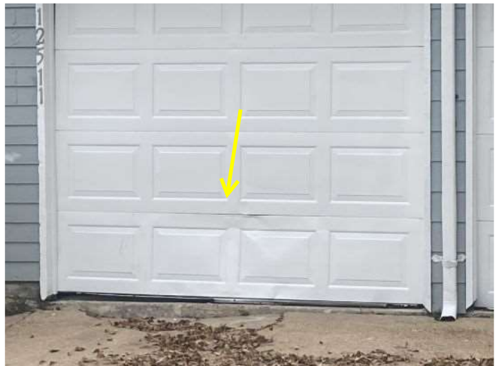
Dents on garage door
