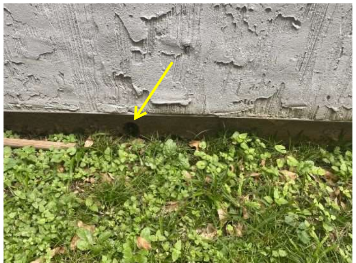
Post tension wire end exposed Rear left
