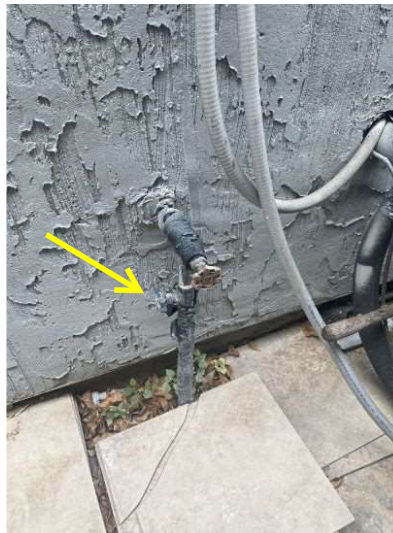
Water main shutoff for the house
