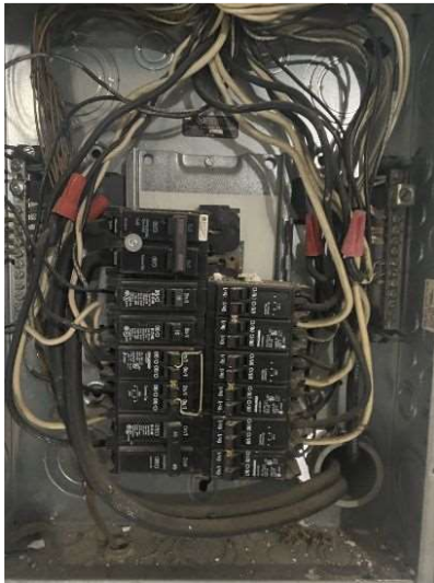
Branch circuit - Copper wiring observed
