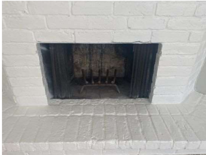
Fireplace installed as per standards
