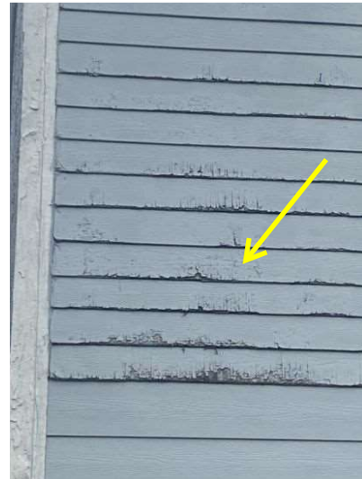
Wood siding deteriorating / weathered
