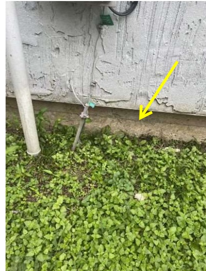
Crack on foundation slab - further evaluation recommended
