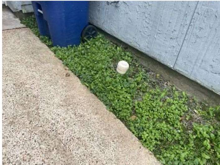
Plumbing main cleanout
