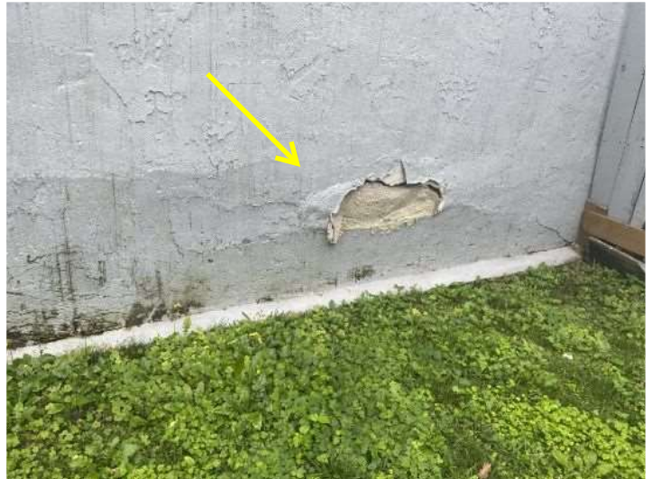
Cement parging off - rear wall
