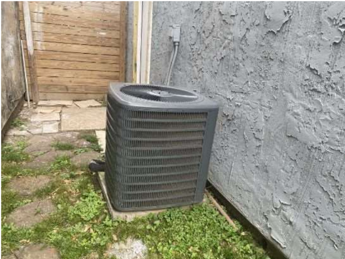
AC compressor installed as per standards
