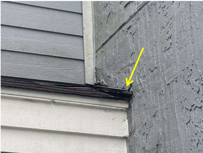
Corrosion weathered area - flashing corroded as well
