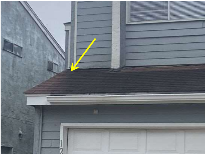
Flashing uplifted -corrosion observed
