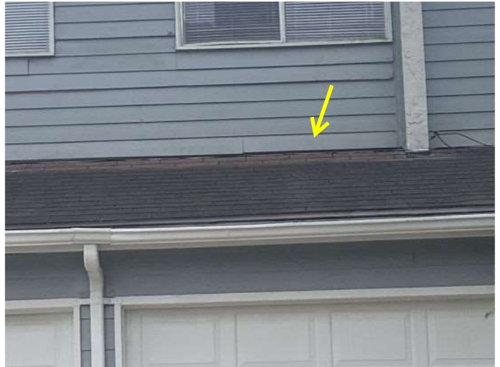
Flashing uplifted -corrosion observed
