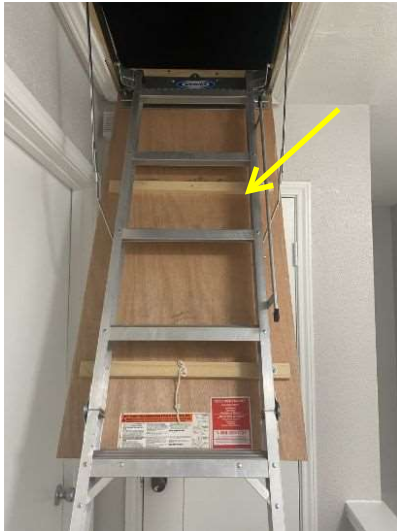
No fire resistant insulation installed
