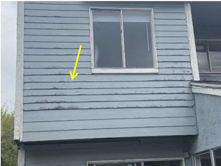
Siding weathered - rear
