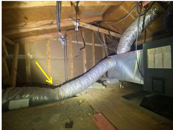
Ducts not hanging
