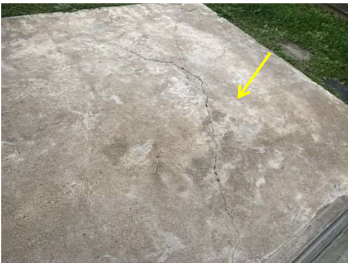
Cracks on patio slab
