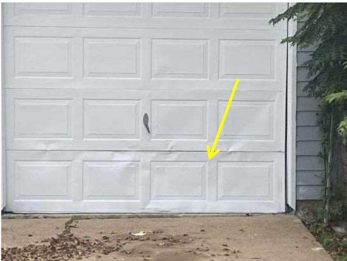
Dents on garage door
