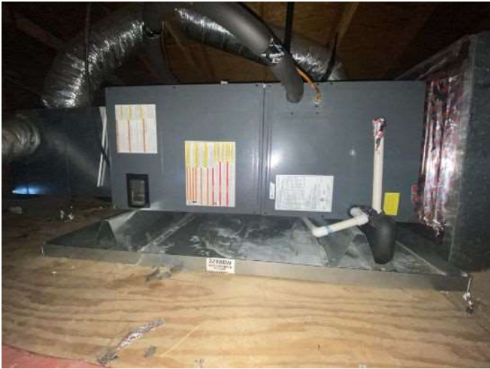
Furnace installed as per standards
