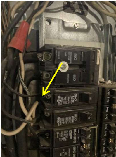
Anti Oxidant needs to be applied on service entrance Aluminum wires
