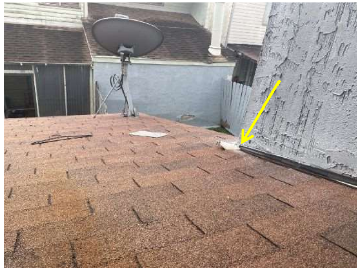
Flashing uplifted -corrosion observed
