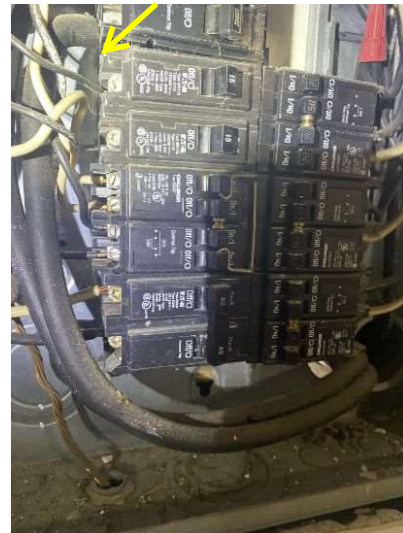
White wire used as hot wire not labeled
