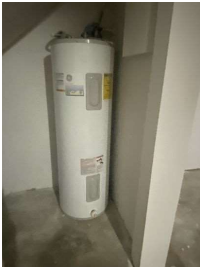
water heater located in Garage
