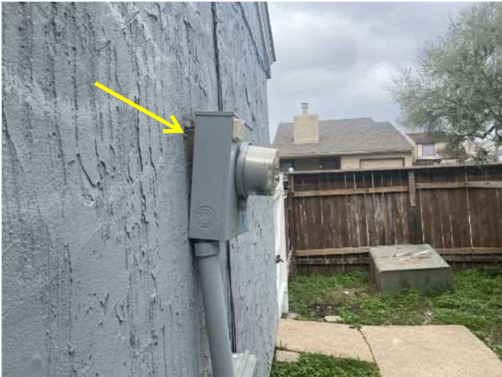
Electrical meter falling off the wall
