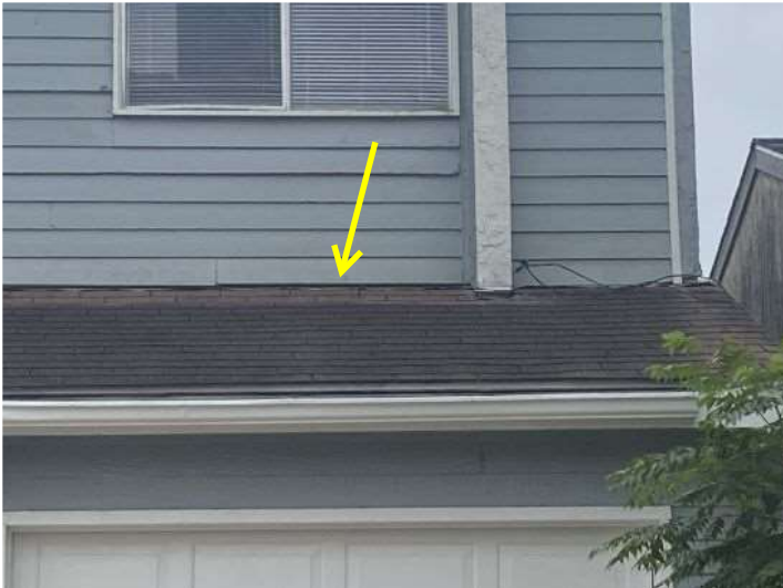
Flashing uplifted -corrosion observed
