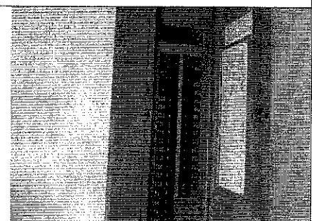
Missing ARC Breakers
