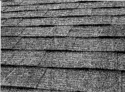
Signs of Aging/Granule Loss
