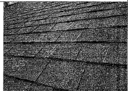
Signs of Aging/Granule Loss
