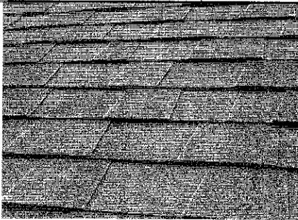
Signs of Aging/Granule Loss
