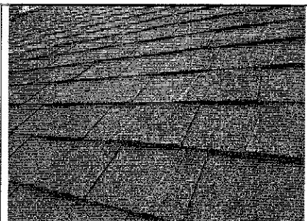
Signs of Aging/Granule Loss
