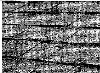
Signs of Aging/Granule Loss
