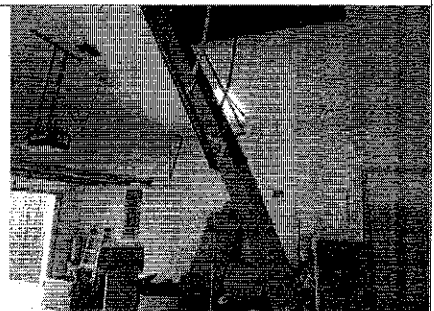
Access Ladder Not Fire Rated
