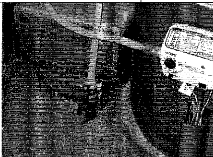
Missing Sediment Trap
