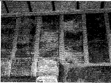
Cracks at Front
