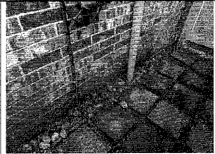
Ground Rod Not Visible
