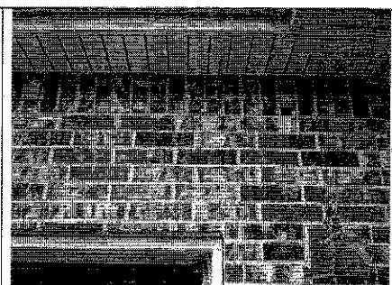
Cracks over Garage Door
