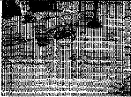
Stopper Not Functioning Proper
