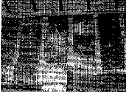
Cracks at Front
