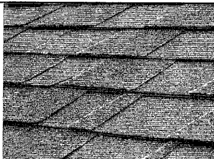
Signs of Aging/Granule Loss
