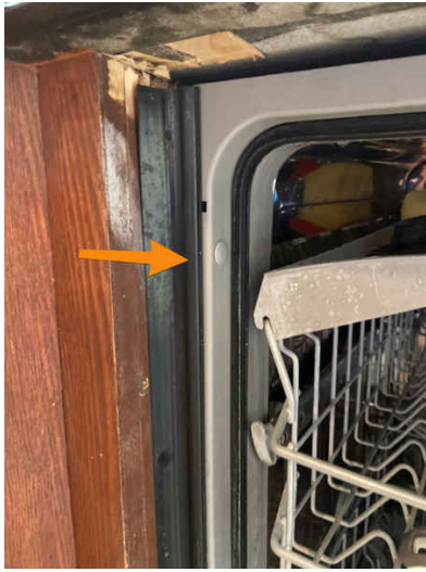
Fasteners are loose
