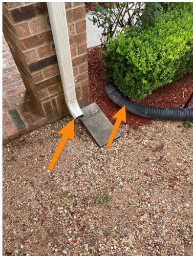
Extension needs to be reattached.
