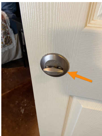
3rd Bedroom, knobs are replaced with dead bolts.
