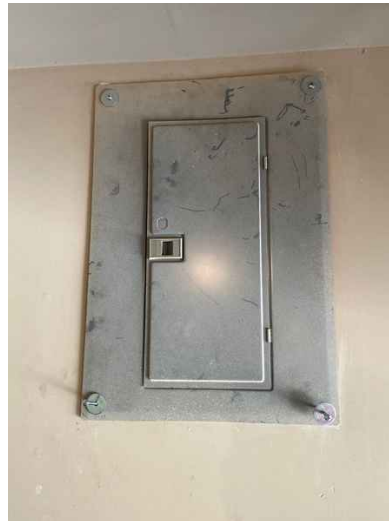
Panel is used as junction box.
