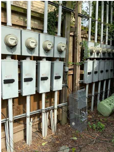
Main panels are not labeled.
