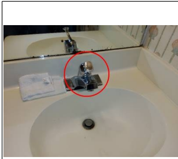
Bathroom sink faucet leaked
