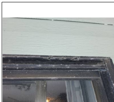
Aluminum sliding glass door is corroding
