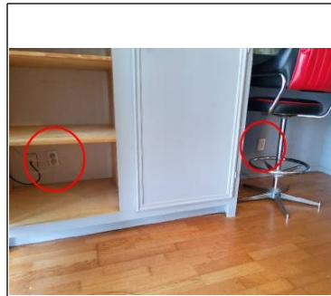
Outlets were not grounded
