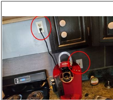
Outlet up top needs to be on GFCI and GFCI outlet needs to be replaced
