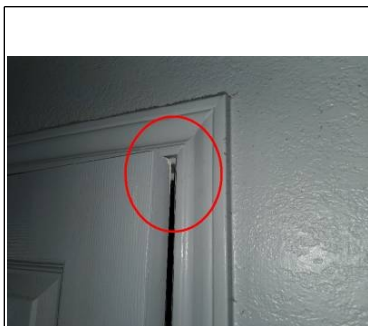
Door for water heater closet needs adjusted or trimmed
