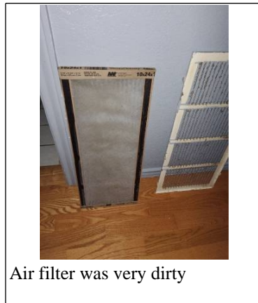
Fungal growth around hvac vents needs cleaned
