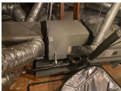
Interior - photo(s) of 2nd cooling system: Electric Central Air Conditioning
