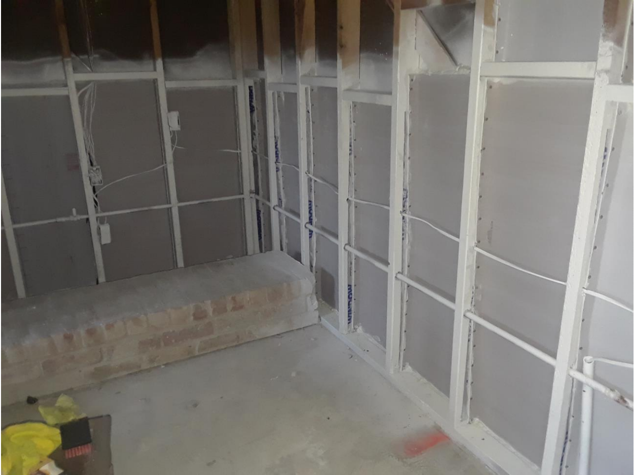
Image shows vapor barrier mitigation work in progress. Entire downstairs was repaired in this manner.
