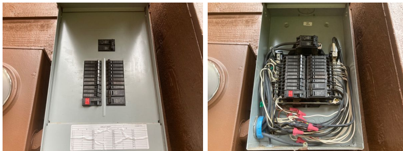
General Infrared Photos of Distribution Panel(s):
