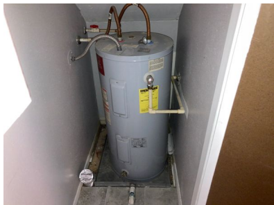
General Infrared Photos of Water Heating Equipment:
