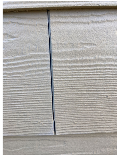
Multiple areas on siding need to be re caulked
