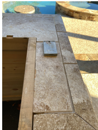
Loose outlet in outdoor kitchen
