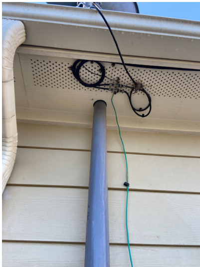
Exterior penetrations should be properly weather sealed
