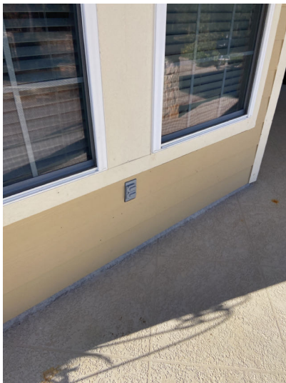
Loose outlet near pool
