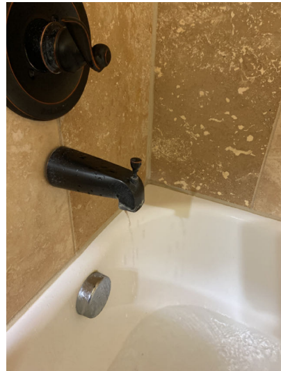
Valve doesn't fully stop when switched from bath to shower in guest bath
