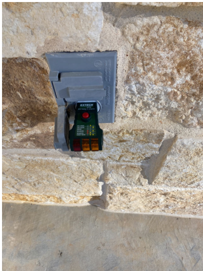
Exterior plug not working
