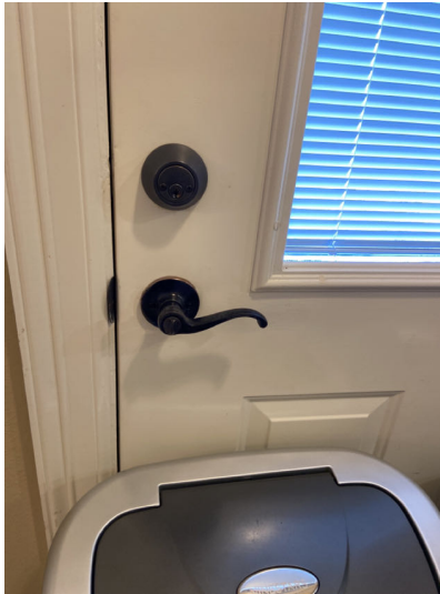
Doors cannot be keyed for exit, it's a fire hazard.
