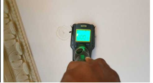
Stained area was dry
