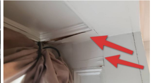
Water damaged finish details
