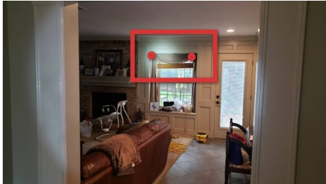
Water damage above living room window
