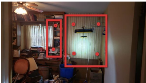
High moisture at and around southeast bedroom dormer window
