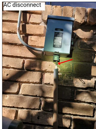
Exterior wiring should be protected by proper conduit.
