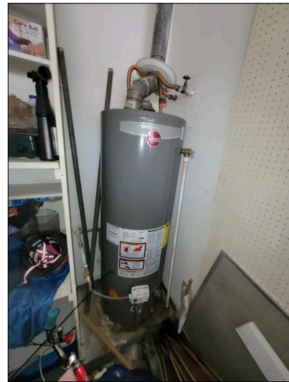
Base should be 18" above garage slab
