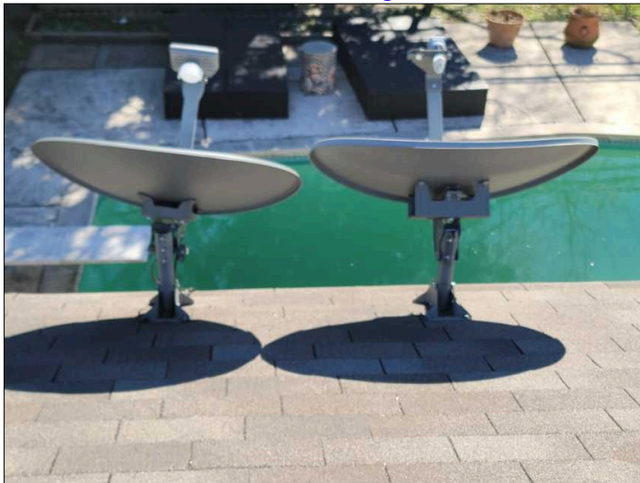
Antenna mounted directly to shingles. Sealant prevents water penetration through screws/nails. Monitor sealant to reduce the risk of water leaks.
