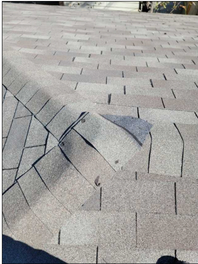
Lifted shingles noted. Ridge shingles installed improperly. These are subject to wind drive rain and water entering house.
