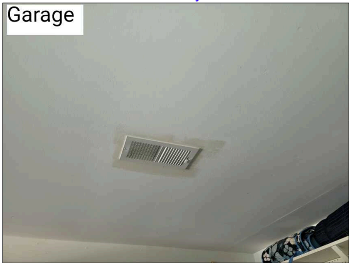
Supply register in garage. This added square footage may be more than the HVAC system was intended to climate control.
