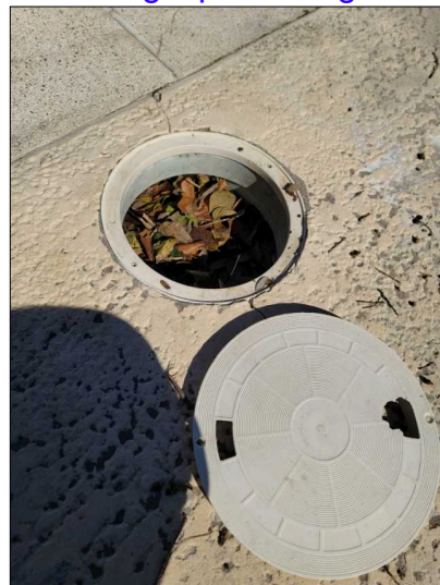
Leaf filters full of debris. Basket cover is cracked.
