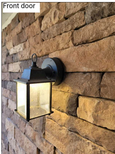
Exterior light fixtures should be weatherproofed.
