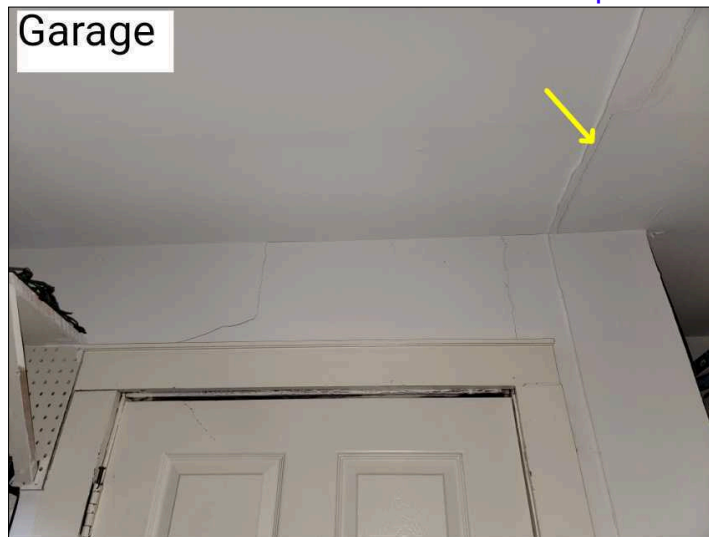
Cracks on ceiling noted.
