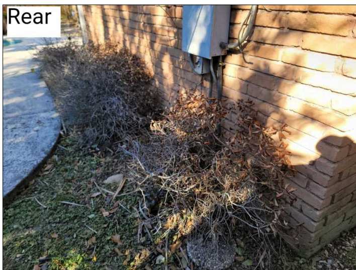
Bushes and shrubs should be clear of house walls by 12" or more. Some in contact with house.
