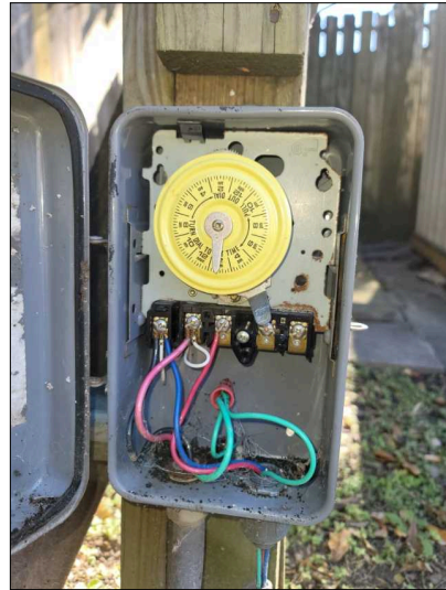
Mechanical pump timer
