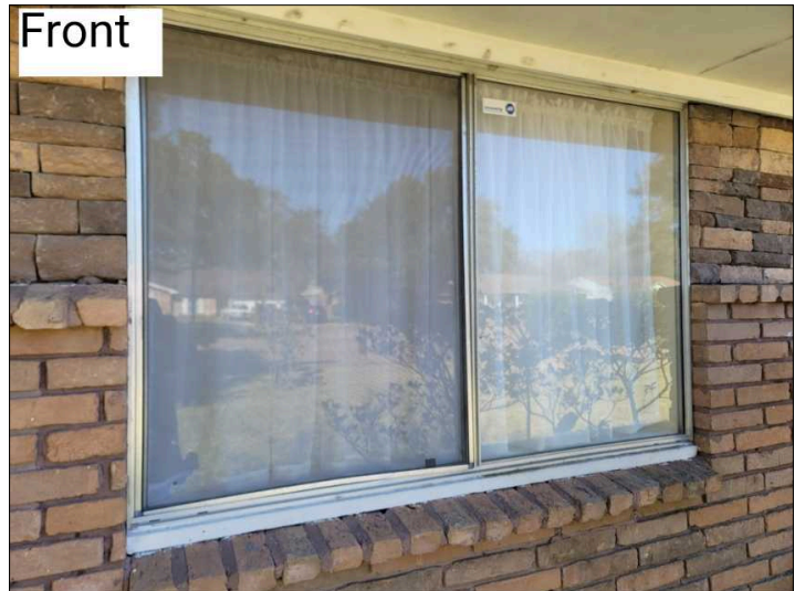
Missing and/or damaged screens noted.
