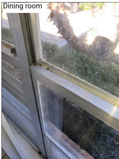
Broken hardware found.
