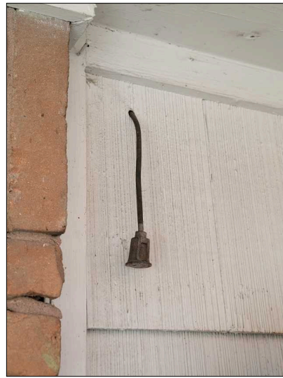
Extension cord used through wall as permanent wiring. Suggest full repair.
