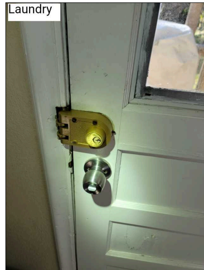
Exterior door has double deadbolt lock. This is a potential life hazard. In the event of a fire, if this is locked and no key is available. People may be trapped inside.
