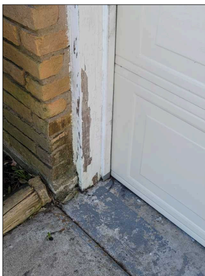
Wood to ground contact at garage door trim. Conducive to wood destroying insects.
