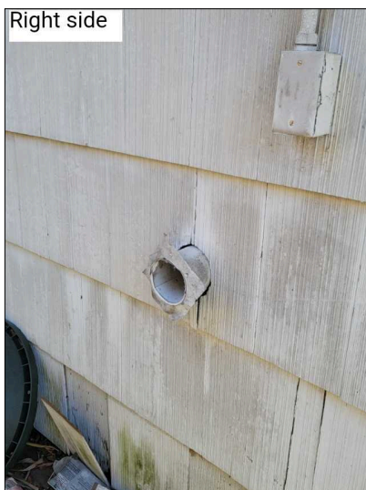
The dryer vent is missing the exterior cover.
