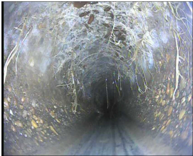
Tree roots were observed with a camera inspection. Tree roots are intrusive, may cause clogs and can grow very rapidly. Main Lateral Sewer -Yard to City Connections
