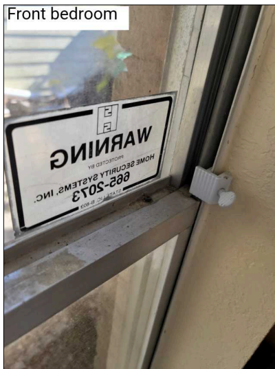
Broken hardware found.
