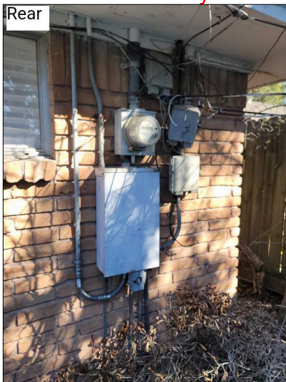
Electric meter and service panel
