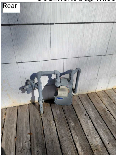
Gas meter and shutoff
