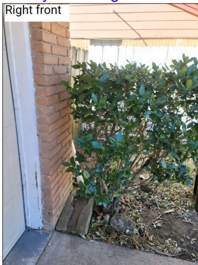
Bushes and shrubs should be clear of house walls by 12" or more. Some in contact with house.
