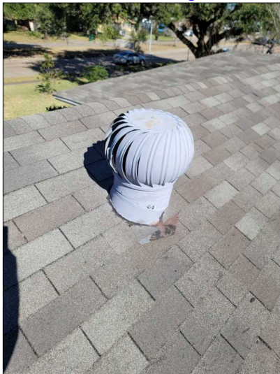
Rusted vents and flashing on roof.
