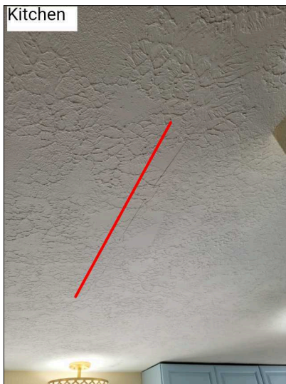
Cracks on ceiling noted.
