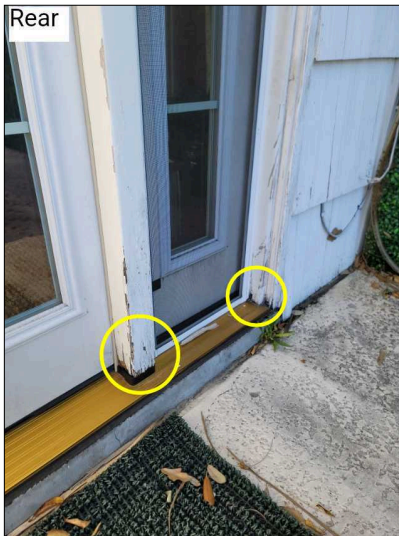
Wood rot / damage noted at door and door trim.
