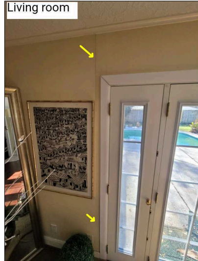
Cracks and/or holes in drywall noted.
