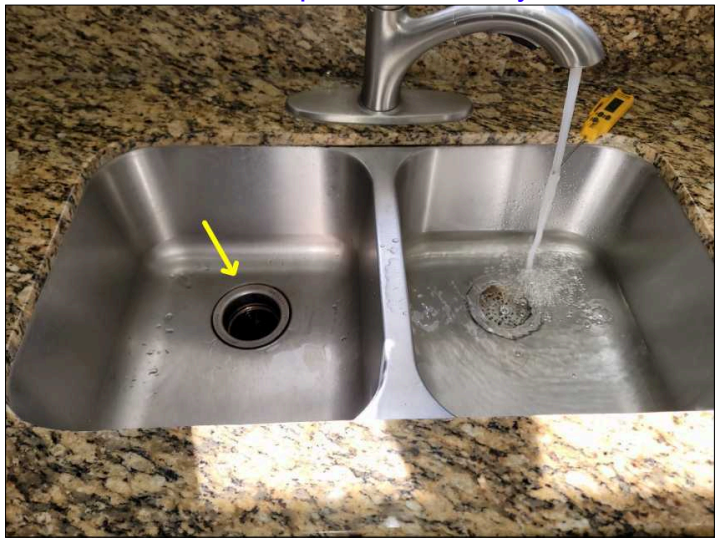
Missing stopper in sink / tub.
