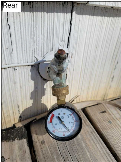
Static Water Pressure Reading: 60 psi. Backflow preventer not present on exterior hose bib. This will prevent contaminants from flowing back into the potable water system.
