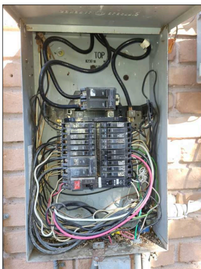
There are white wires in the panel that should be labeled as hot wires
