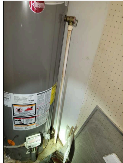
Temperature and pressure valve does not have proper discharge line. This min. 3/4" cpvc line should exit attic space and discharge within 6" of the ground outside.
