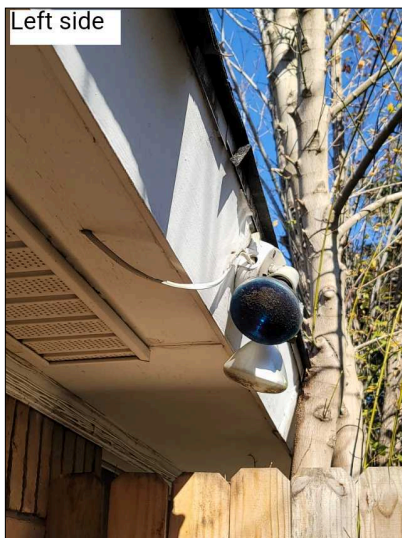
Exterior light fixtures should be weatherproofed. Exterior wiring should be protected by proper conduit.
