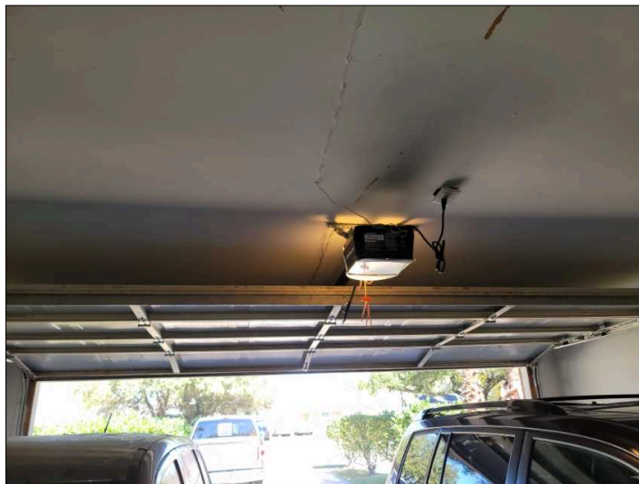
Garage door did not want to close. Suggest adjustment to operator.
