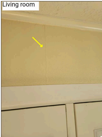
Cracks and/or holes in drywall noted.
