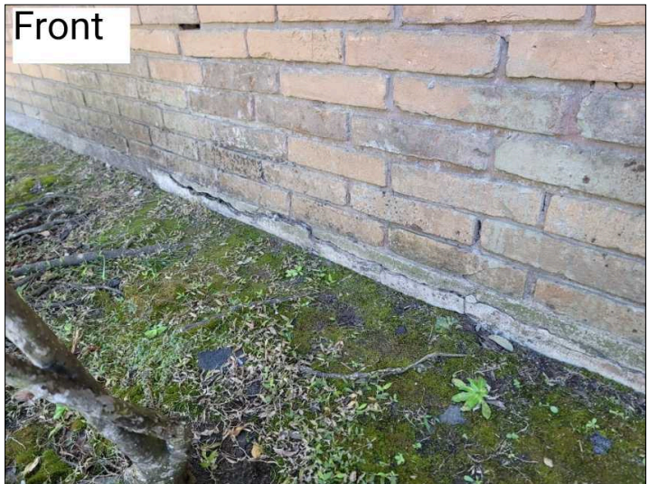
Spalling observed. Spalling is a result of water entering brick, concrete or natural stone and forcing the surface to peel, pop out or flake off
