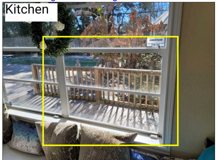
Window did not open in several locations.
