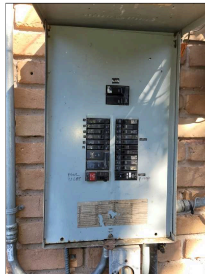
The electrical panel is not properly labeled.
