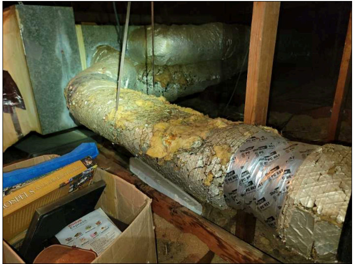
Damaged and missing insulation on metal ducting. Insulation factors may not reach R6.
