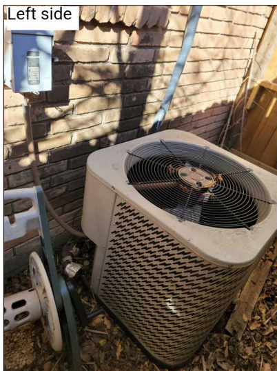
AC compressor, 3.5 ton, R22 refrigerant, manufactured 2010
