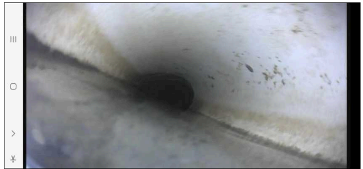
A sewer camera inspection found a significant belly or dip in the pipe. This will hold water and debris and does not fully drain the system. These bellies can cause clogs and excessive pipe deterioration. Main Lateral Sewer -Yard to City Connections
