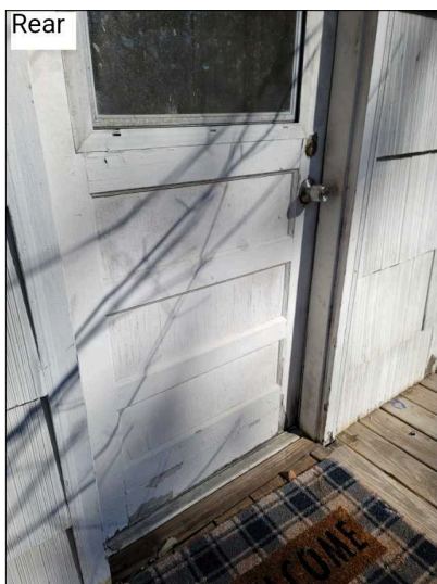
Exterior door is fully exposed to the weather and elements. Paint delamination and damaged. A storm door may help protect the door and door frame from accelerated deterioration.
