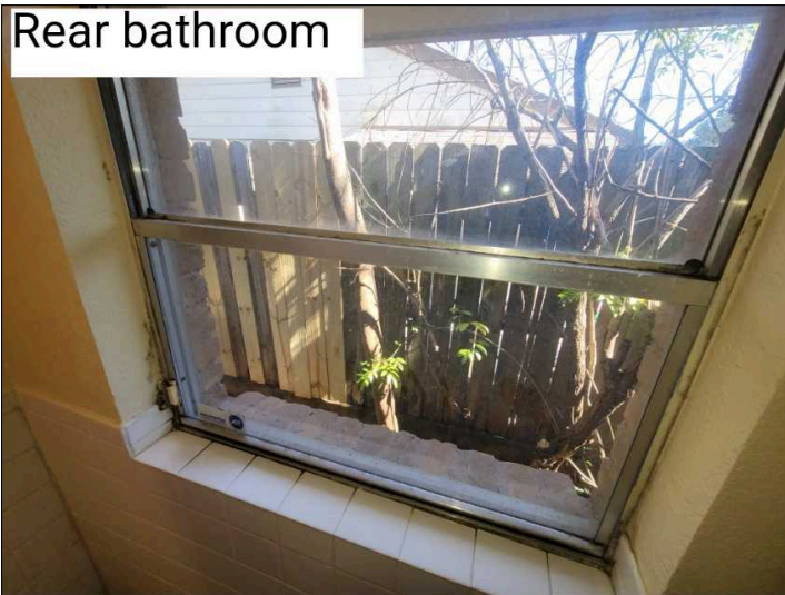
Broken hardware found.
