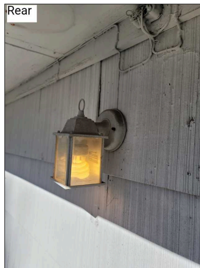
Exterior light fixtures should be weatherproofed.
