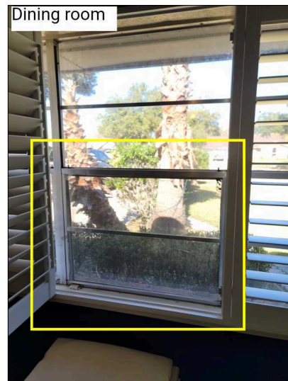
Window did not open in several locations.
