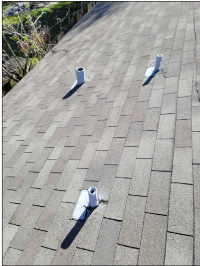
Could not fully inspect vents on roof.
