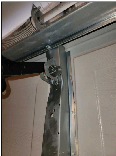
Damaged garage door.
