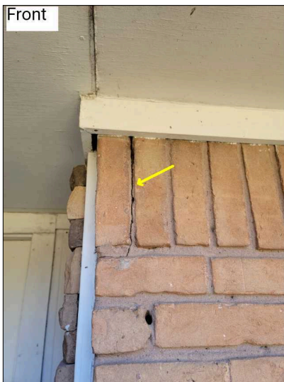
Exterior cracks in brick and/or mortar noted.
