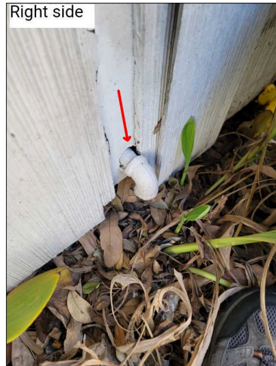
Appears to be abandoned water heater drain line
