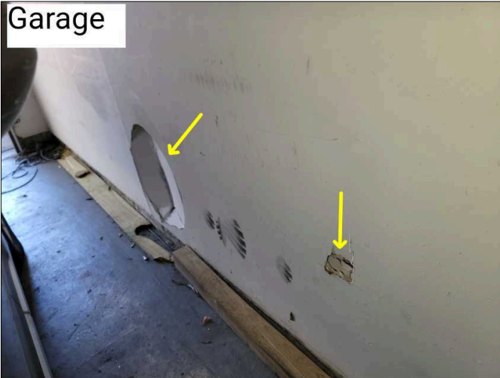
Holes in drywall in garage. These are breaks in the "firewall" and should be repaired to ensure fire rating.
