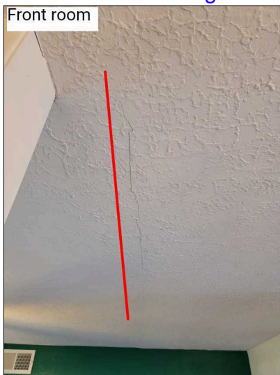
Cracks on ceiling noted.
