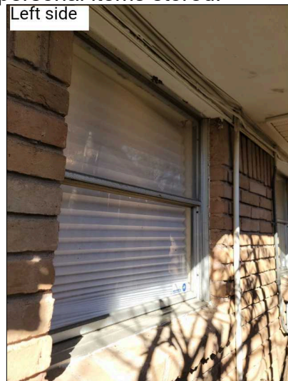
Missing and/or damaged screens noted.
