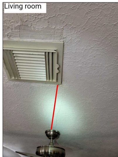
Cracks on ceiling noted. Patched areas on the ceiling.
