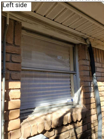
Missing and/or damaged screens noted.
