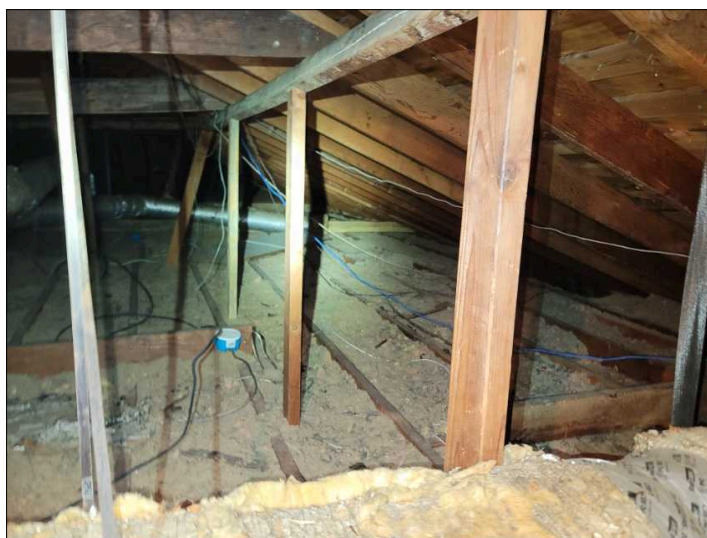
Insulation thickness varies. Suggest additional insulation to meet R30 requirements for our area.
