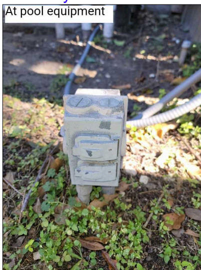
Outdoor receptacles should be GFCI protected and have an "in-use" weatherproof cover. Additionally "WR" (weather resistant) receptacles should be used. All these items are to help prevent electrocution.
