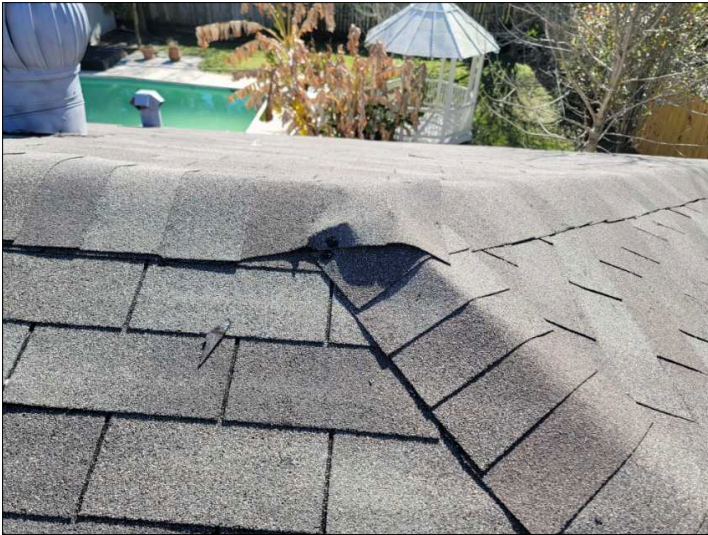
Lifted shingles noted. Ridge shingles installed improperly. These are subject to wind drive rain and water entering house.
