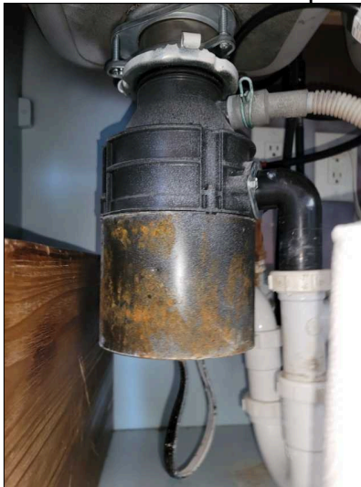
There is rust present on or inside the disposal unit.
