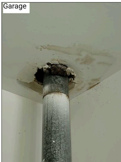
Water stain noted on ceiling. Inaccessible for moisture readings.
