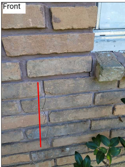
Exterior cracks in brick and/or mortar noted.
