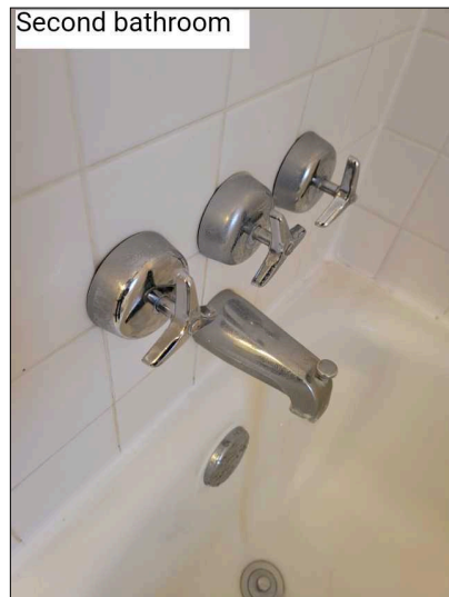
Suggest sealing around faucets in shower to prevent water from entering wall.
