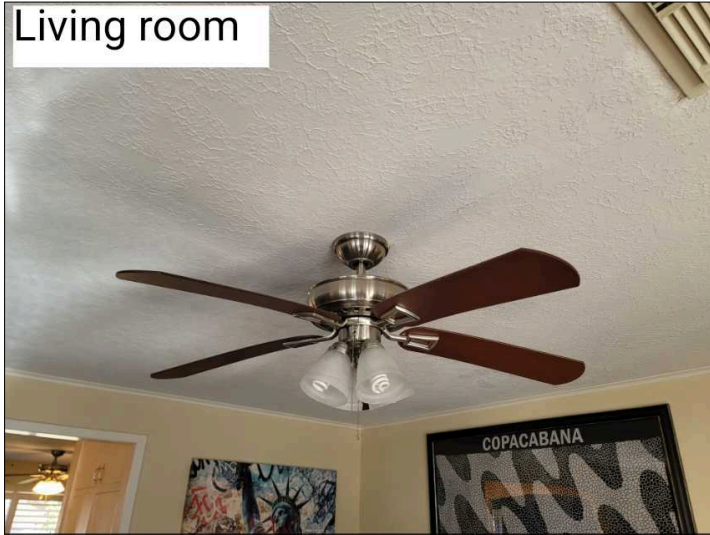
Inoperable ceiling fixture, no switch located.
