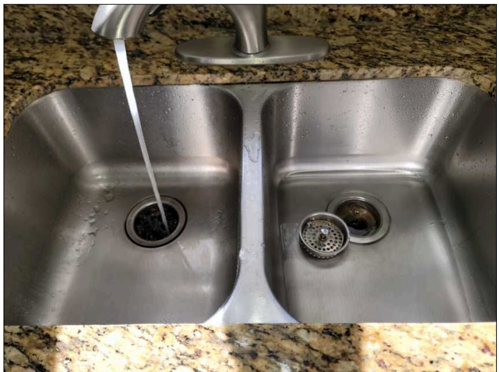
Drains slow. Suggest having plumber to snake drains.
