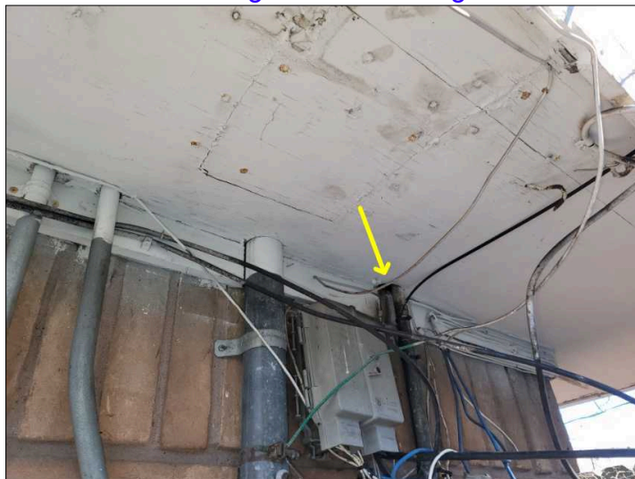
Open holes noted at edge of attic space. These could be a location for rodents to enter.
