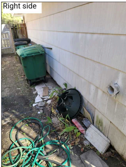
Heavy debris against walls.
