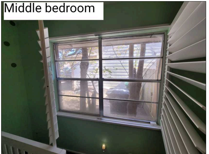
Window did not open in several locations.
