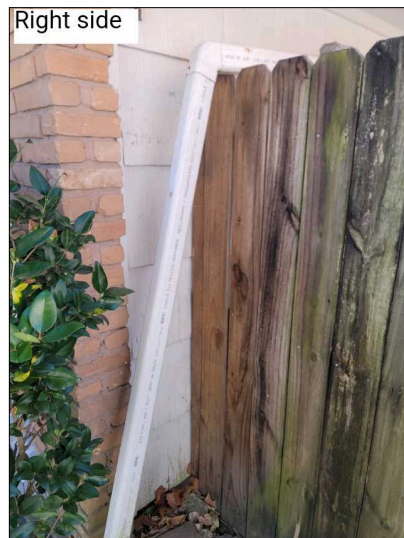
Wood in contact with house.
