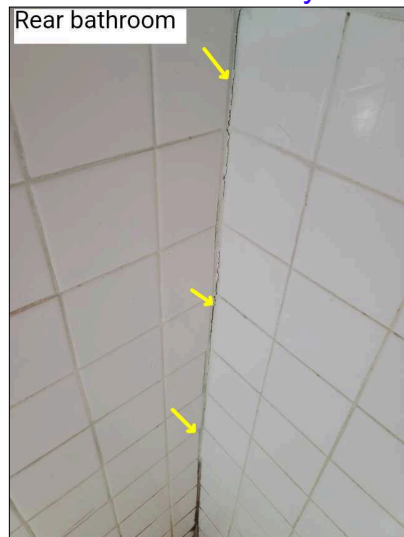
Cracks in grout in shower/tub. Recommend sealing to prevent water intrusion.
