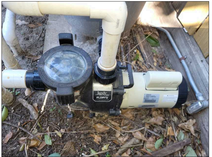
Missing bonding wire from pump
