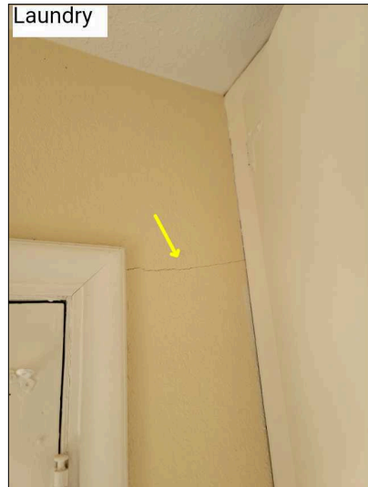
Cracks and/or holes in drywall noted.
