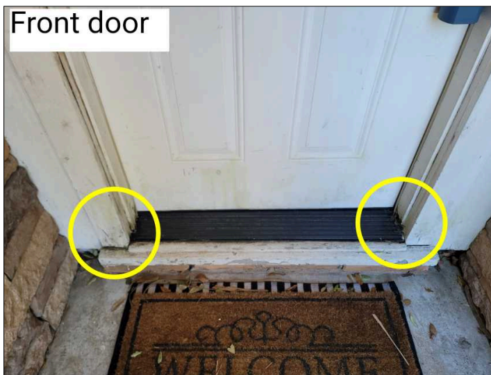
Wood rot / damage noted at door and door trim.
