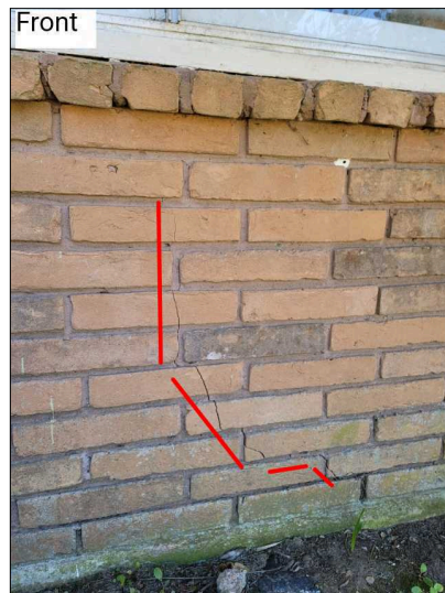
Exterior cracks in brick and/or mortar noted.
