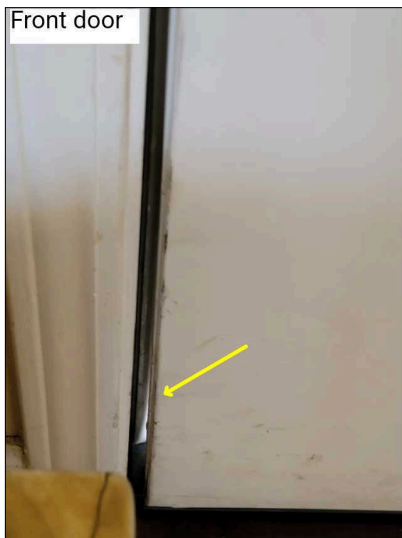
Missing / damaged weatherstripping at door.
