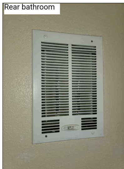
Loose switch at wall heater, not tested
