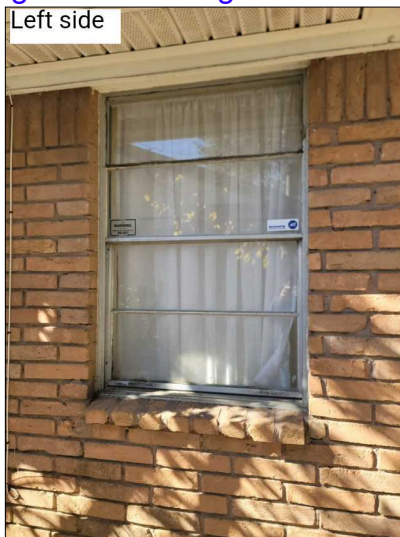
Missing and/or damaged screens noted.
