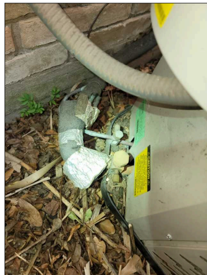
Missing locking refrigerant caps. These caps prevent tampering and possible chemical abuse.
