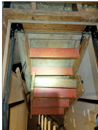
Attic ladder has loose or damaged hardware. Suggest repairs prior to using access ladder.
