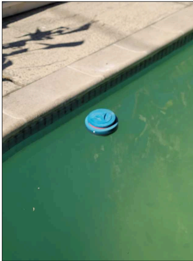
Floating basket chlorinator noted. No automated disinfectant installed.
