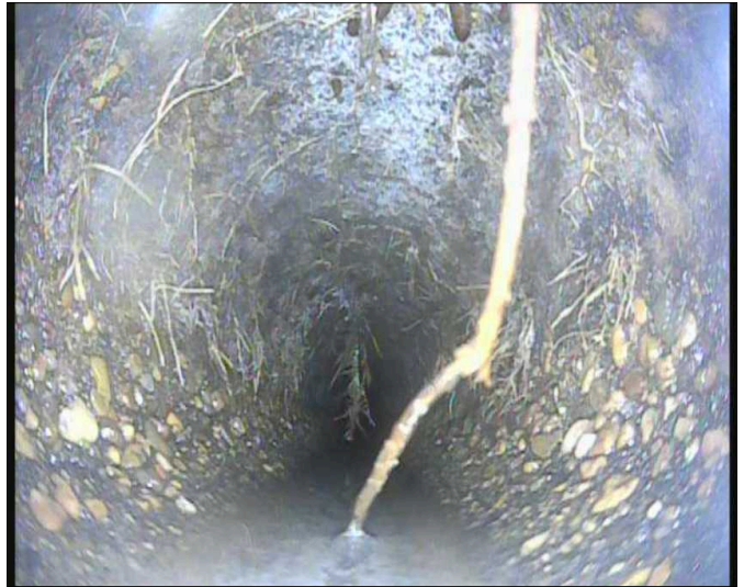
Tree roots were observed with a camera inspection. Tree roots are intrusive, may cause clogs and can grow very rapidly. Main Lateral Sewer -Yard to City Connections
