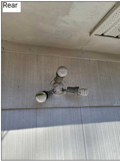
Some lights / switches did not function at time of inspection.
