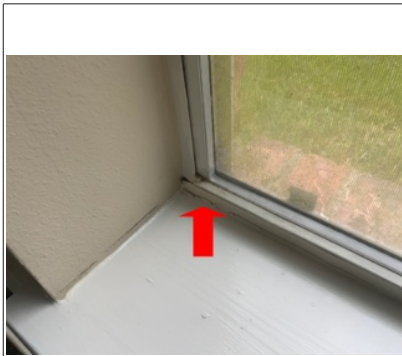
Interior caulking improvements needed throughout home.
