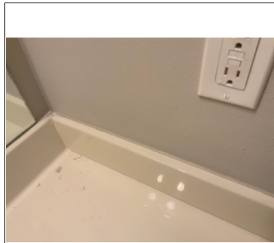
Vanity seal improvements needed at upstairs J&J bathroom.
