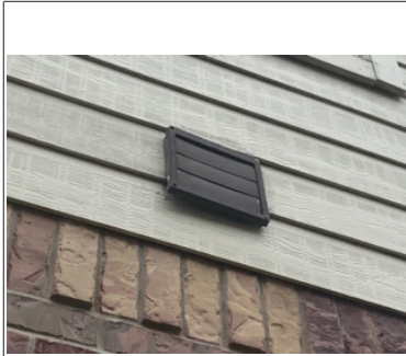
Vent cover damaged at left of home.
