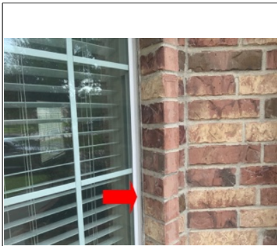
Exterior caulking improvements needed at front of home
