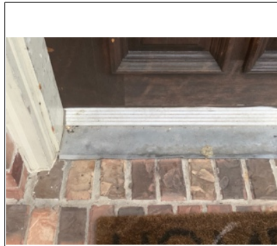
Damaged threshold at entryway door.
