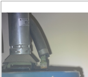
Corrosion at supply line.
