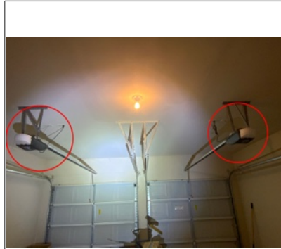
Garage door openers do not operate.
