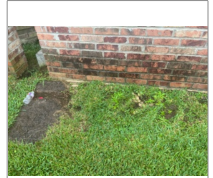
Grading improvements needed at Back of home.
