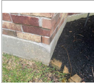
Broken front left corner.
