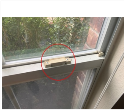
Damaged hardware at office.
