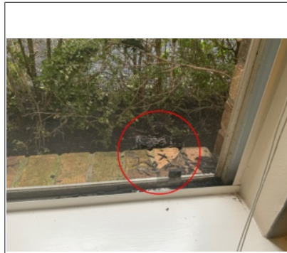
Damaged screen in office.
