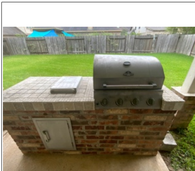
Inoperative at the time of the inspection.
