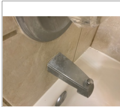
Faucet seal improvements needed at upstairs bathroom bathtub.
