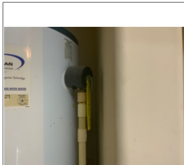
Inoperative TPR valve.
