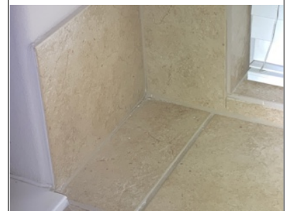
Enclosure grout improvements needed at primary bathroom bathtub.
