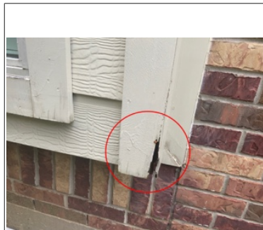
Decaying siding at right of home.
