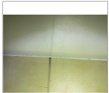
Bathtub base seal improvements needed at upstairs J&J bathroom.
