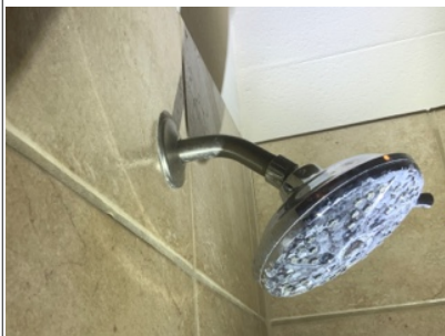
Faucet seal improvements needed at primary bathroom shower.
