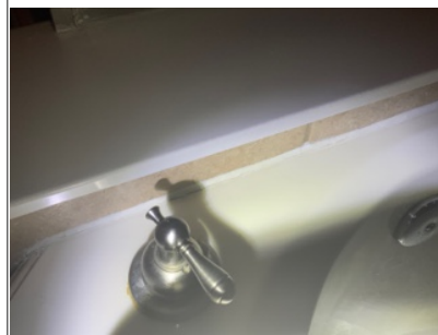
Bathtub enclosure caulking improvements needed at primary bathroom bathtub.
