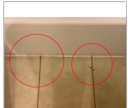
Cracked tiles at upstairs J&J bathroom.
