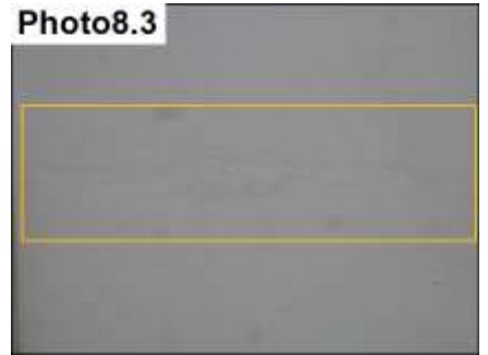
Hairline Cracks And Efflorescence Noted/ Clean/ Paint
