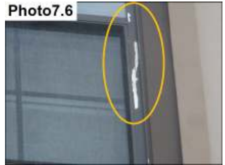
Deteriorating Paint/ Clean And Paint
