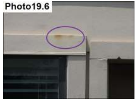
Rust Stains/ Clean And Paint
