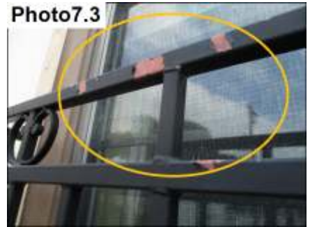
Deteriorating Paint/ Clean And Paint
