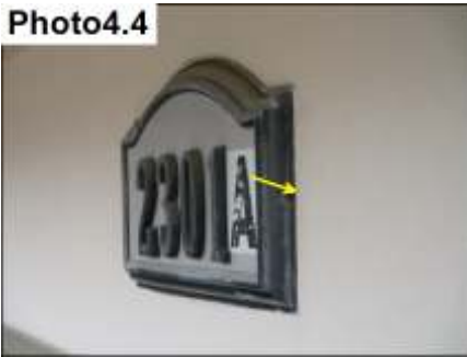
Penetration Sealants/ Seal
