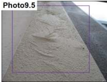
Delaminating Paint/ Clean, Prime And Re-Paint
