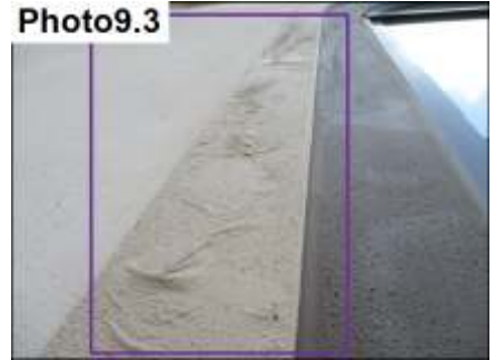
Delaminating Paint/ Clean, Prime And Re-Paint
