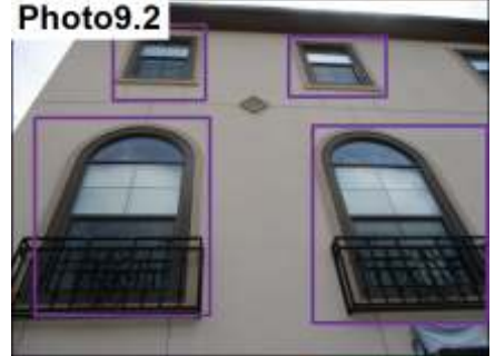
Delaminating Paint/ Clean, Prime And Re-Paint
