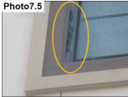
Deteriorating Paint/ Clean And Paint
