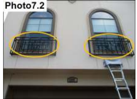
Deteriorating Paint/ Clean And Paint
