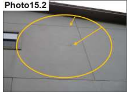
Delaminating Paint And Moisture Intrusion/ Repair And Resurface
