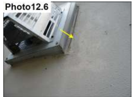
Penetration Sealants/ Seal
