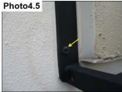
Penetration Sealants/ Seal
