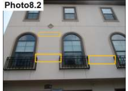
Hairline Cracks And Efflorescence Noted/ Clean/ Paint
