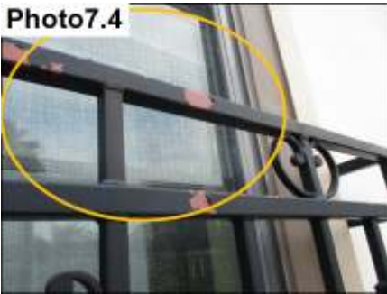
Deteriorating Paint/ Clean And Paint
