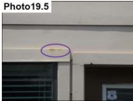
Rust Stains/ Clean And Paint
