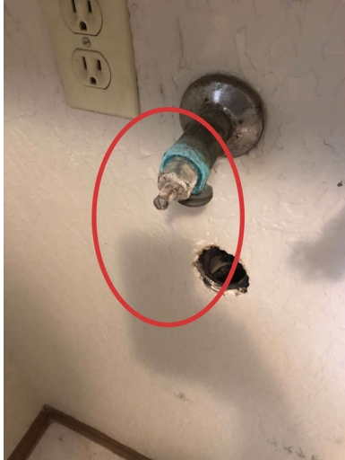
Missing handle at washer connection
