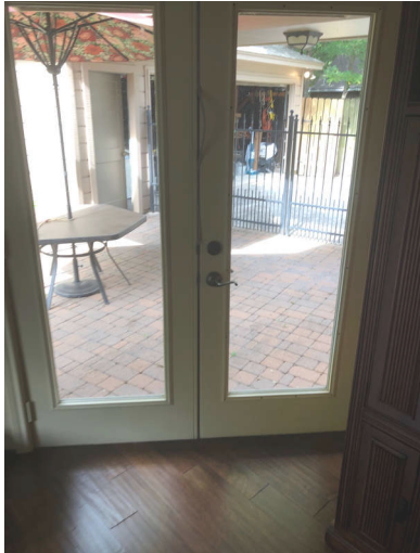
Inoperable-could not open
