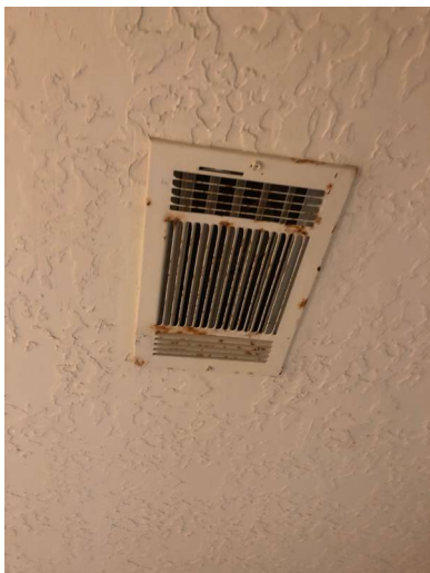
Master Bathroom: most likely from lack of venting
