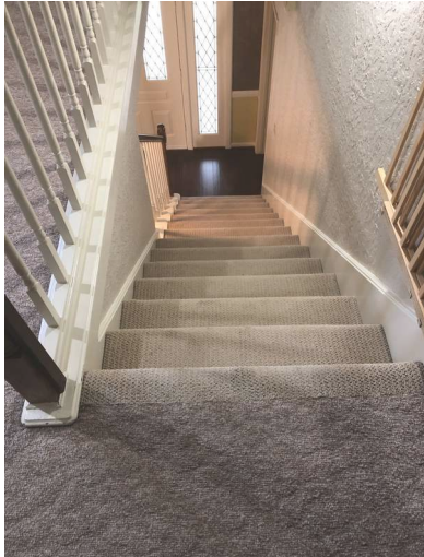
No hand rail at top section
