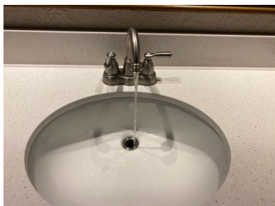
2nd Floor Bathroom #1 , Hot Water Side
