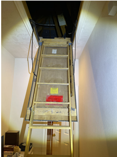
Attic ladder not insulated
