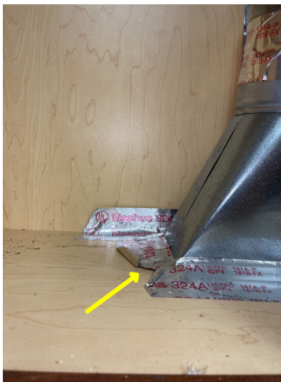
Minor air loss
