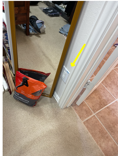
GFCI reset location in master closet
