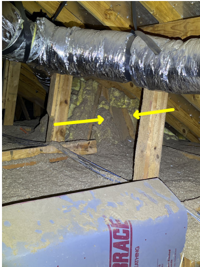
Missing insulation at left skylight wall
