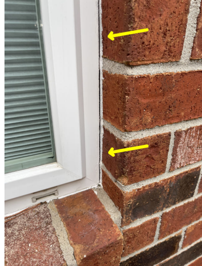
Additional sealant needed at all windows
