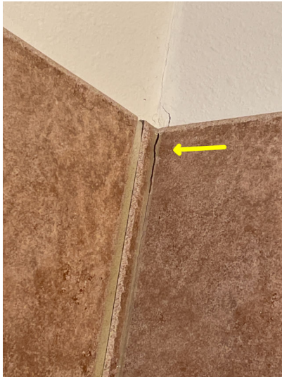
Grout/sealant needed at top corner of master shower
