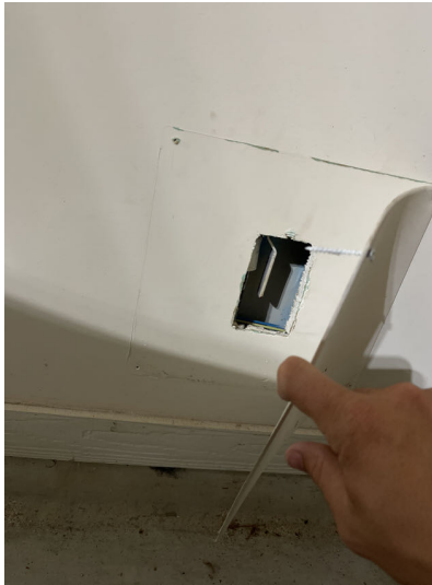
Main water shut off inside garage
