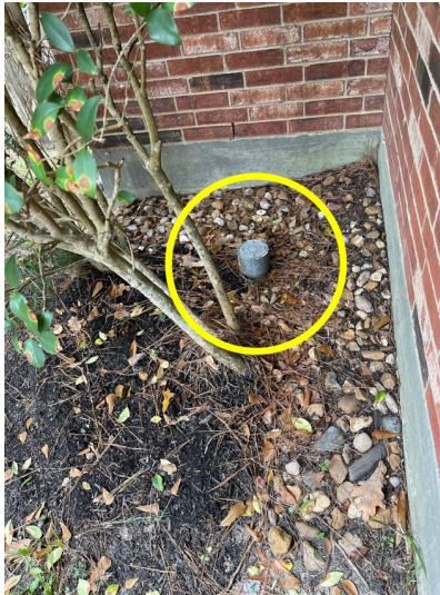
Main sewer clean out at left side
