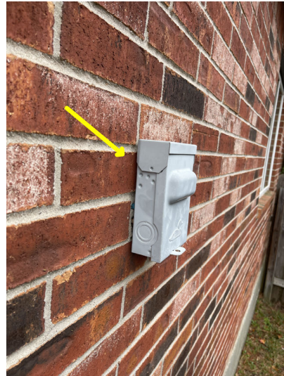
Sealant needed at left side disconnect box
