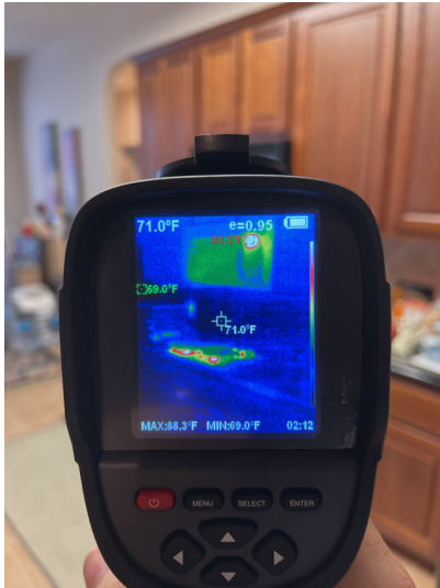
Thermal scan performed - no anomalies
