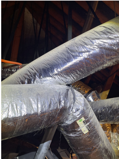
Ducts in contact
