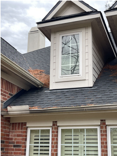
Debris and valleys needs to be cleaned
