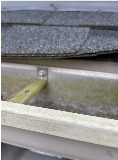
Gutters not behind drip edge flashing
