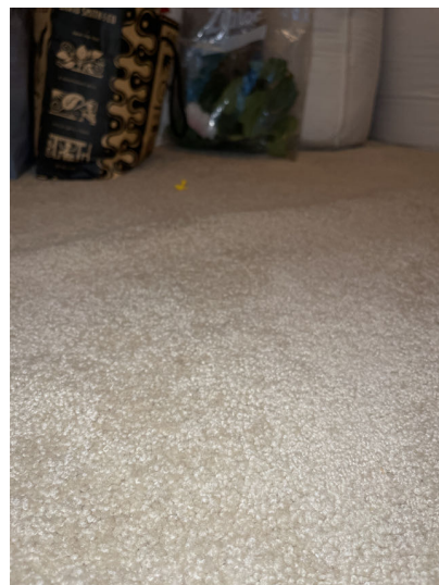
Loose carpet at rear right bedroom closet
