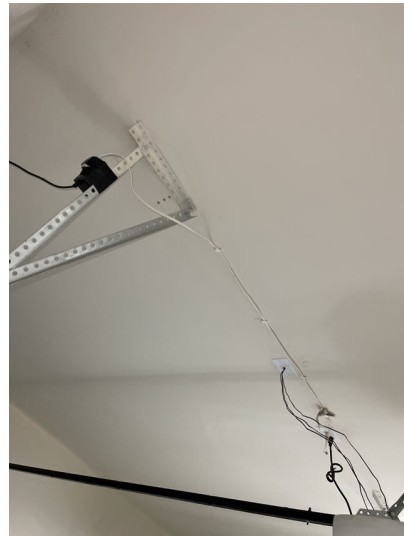
Extension cord permanently in use in garage for irrigation system
