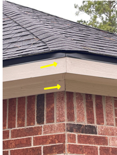
Sealant needed at siding joints - multiple locations
