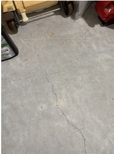
Normal shrinkage cracks in garage
