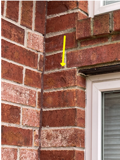
Minor mortar crack at rear window
