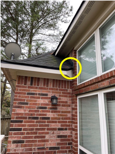
Kick out flashing needed at rear
