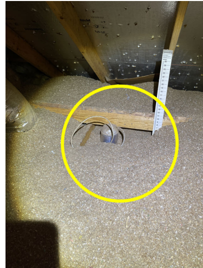
Low insulation around right side sunroom ceiling
