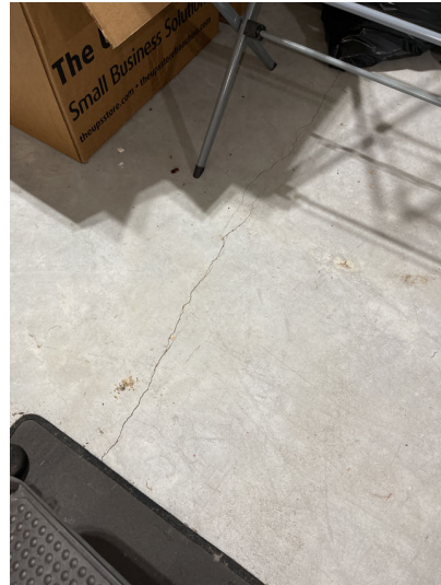
Normal shrinkage cracks in garage
