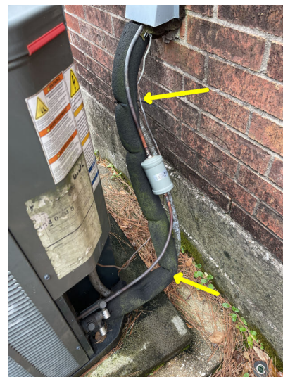
Insulation not sleeved
