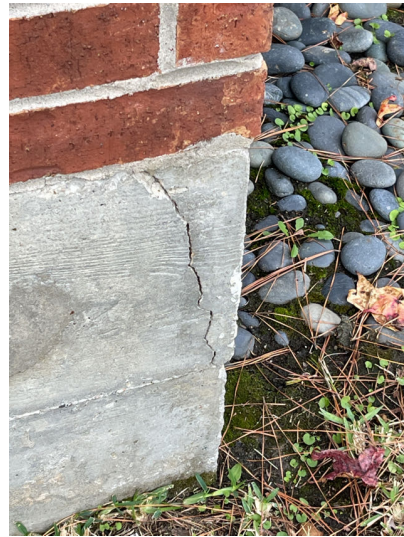
Cosmetic corner crack at rear
