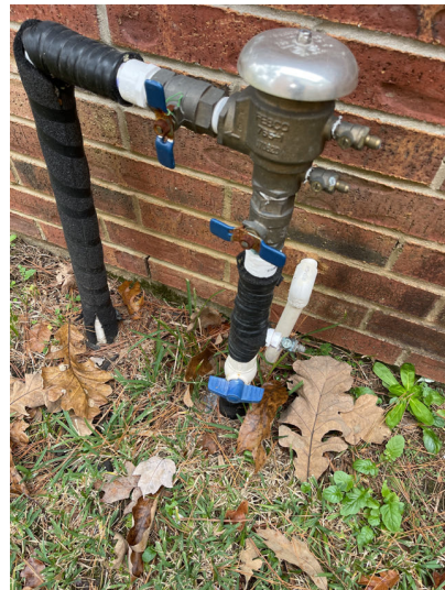
All valves turned off
