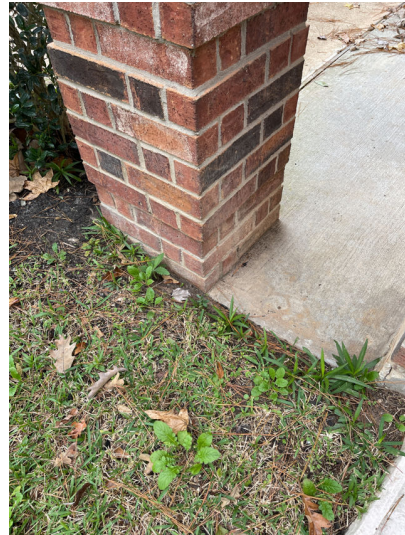
No weep holes at column
