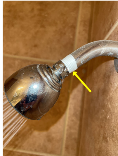
Slow leak at right hall bath shower head
