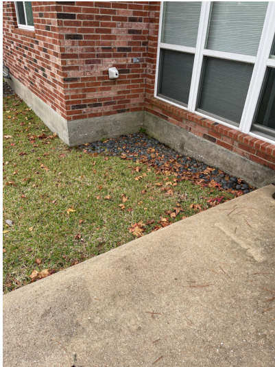
Improper slope at rear - both sides of patio
