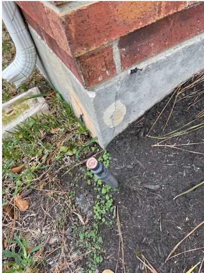
Cosmetic crack at front left corner
