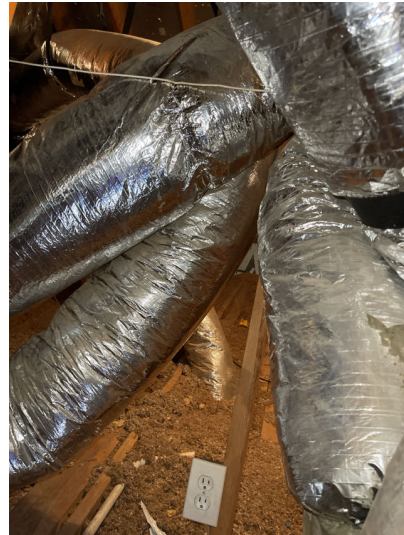
Ducts in contact
