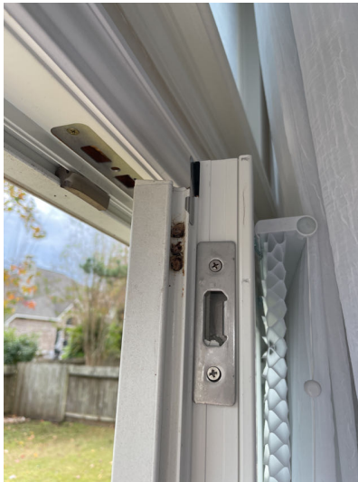
Flush bolts not installed
