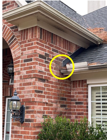
Kick out flashing needed at front
