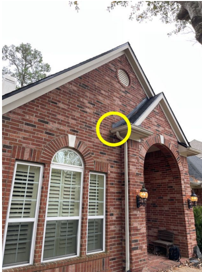
Kick out flashing needed at front
