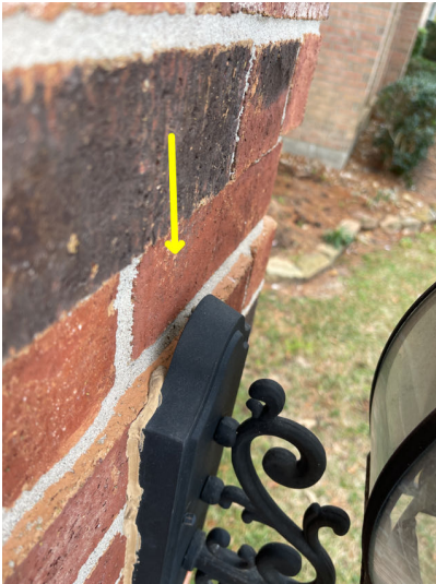
Sealant needed at exterior lights
