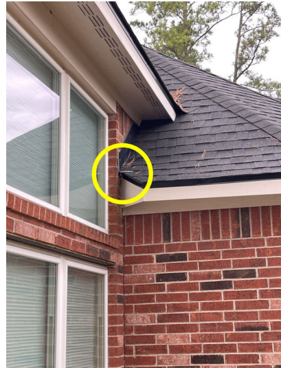
Kick out flashing needed at rear
