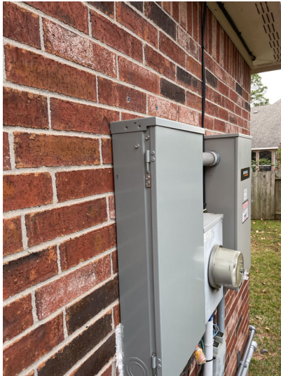
Sealant needed around right side electrical boxes
