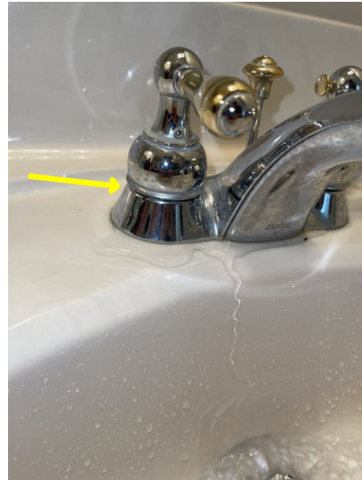
Hot water valve leaked - right master vanity
