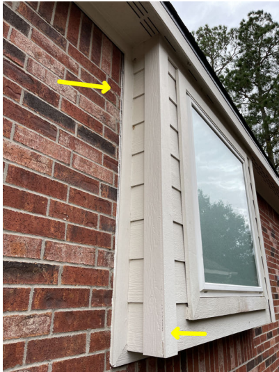
Sealant needed at left side window trim
