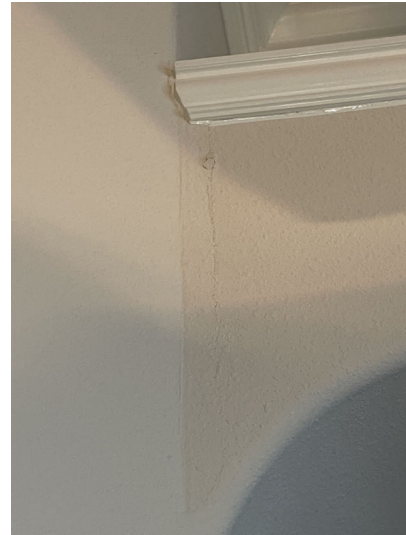
Cosmetic drywall tape joint at living room
