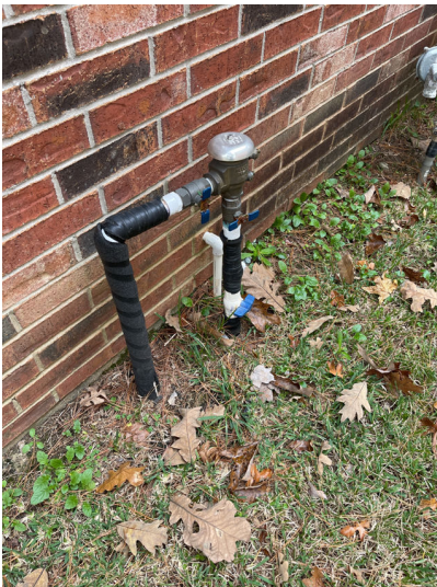
Not anchored in place, not fully insulated
