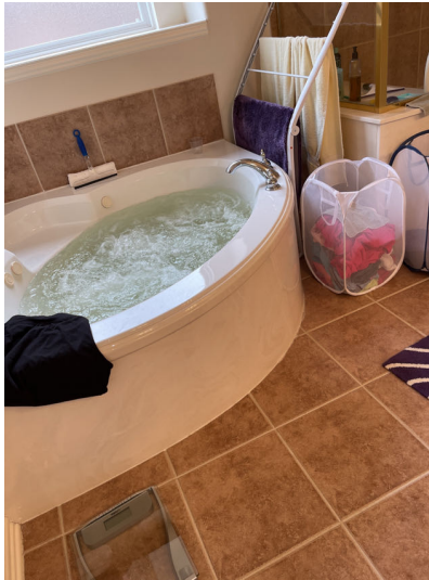
No access panel to view motor
