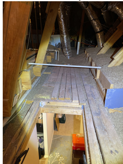
Pipe in walkway not protected
