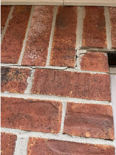
Loose mortar at right side window
