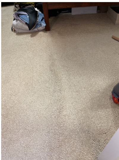
Loose carpet at master closet
