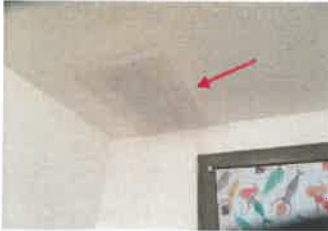
Indications of sheetrock repair in downstairs apt.
