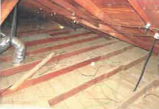
Reference picture shows the lack of insulation in the attic.
