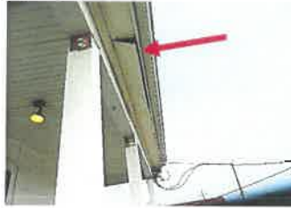
A section of the enclosed soffit along the front eave has come loose.
