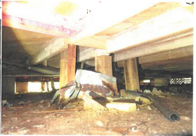
Spotted piers propped under individual joist not beams
