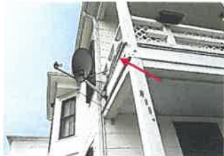
Damage to upper porch area along the left side.
