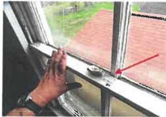
As shown the upper section of the window has dropped lower than the lower section and the window lacks a latch.
