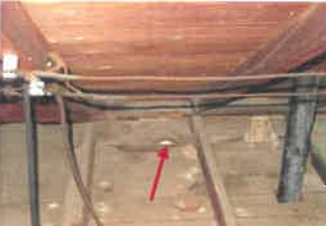
Damage to soffit area along the left side ( Forward of waste stack)
