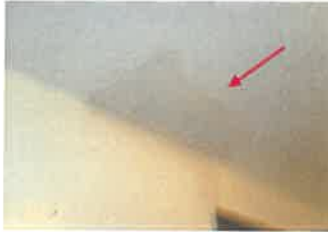
Indication of sheetrock painting or repair.
