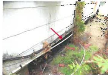
Water supply line ran along the exterior of the building drooping
