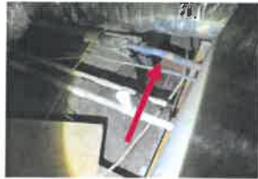
Low pressure line at evaporator not insulated.
