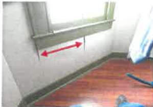
Plywood wall covering separating in upstairs Apt front bedroom.
