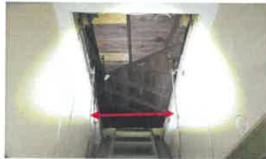
Both of the attic drop staircase springs or loose or damaged and get hung up on the pulleys.
