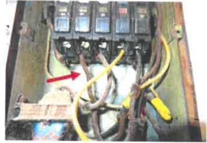
Older cloth wiring exist in the sub panel located in the upstairs apt.
