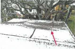
It appears a lot of the granules on the flat area of the roof are gone leaving the mat exposed to the sun
