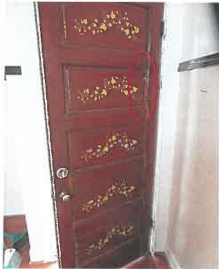
Damaged panel of exterior back door of upstairs apt.
