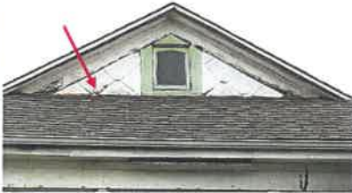
The vertical wall flashing along the front is rusted and should be checked.
