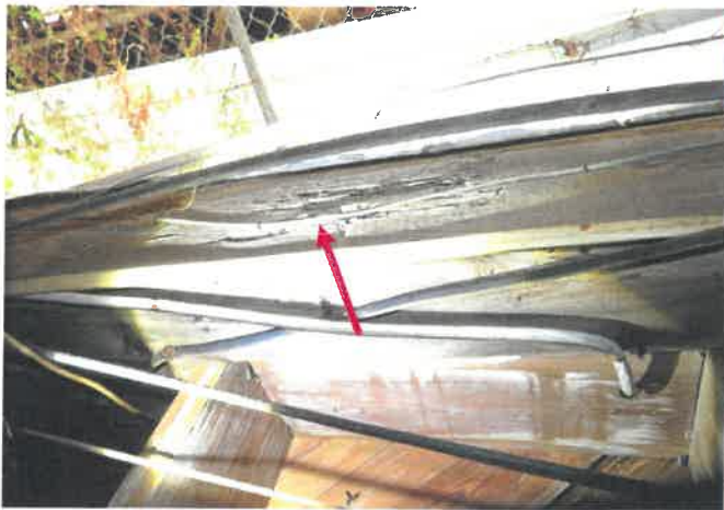
Minor deterioration to beams in spotted areas
