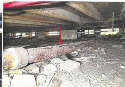
Entire main drain is cracked and in need of repair
