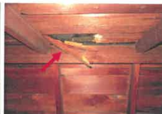
Damaged section of roof decking along right gable where the roof covering has nothing to nail to.
