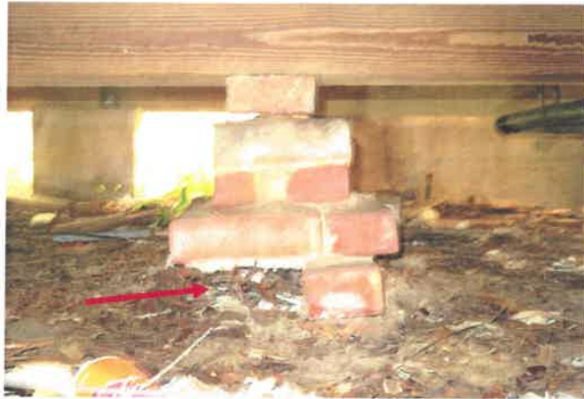
Make shift masonry piling along front beam is damaged, and does not make a good support due to a missing brick,
