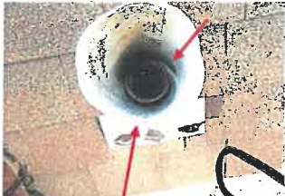
The arrow points to the plumbing vent which is not properly sealed
