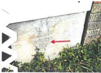
Front left corner concrete pier has a vertical crack which should be checked.
