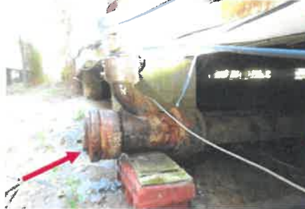
Drain line leaks >>>>>
