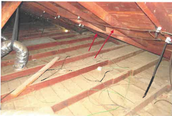
Knob and tube wiring observed in attic
