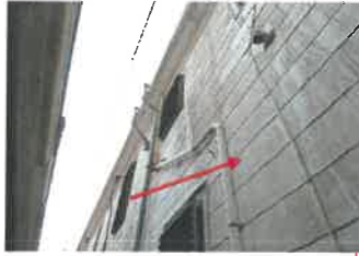
Exterior tiles discolored or stained
