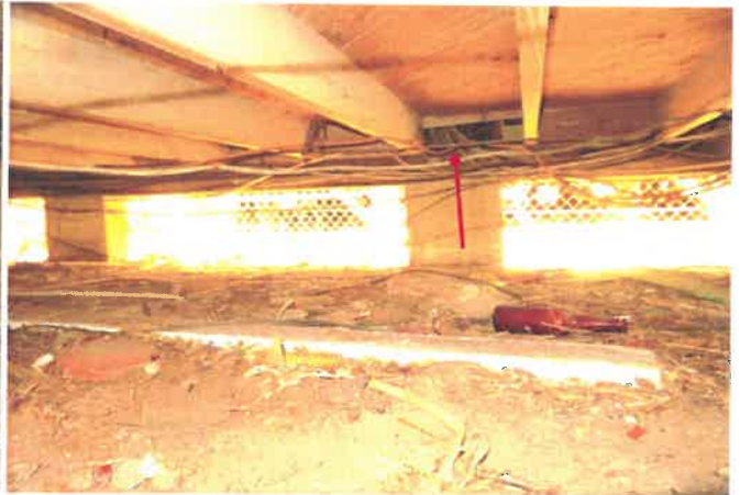
One of the areas above the beam is not block where wires pass which may allow pest to enter.
