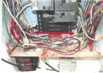
The above reference pictures shows several of the electrical wires passing thru a couple of panel knockouts w/o use of non metallic bushing.
