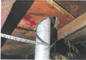
Insufficient space between gas furnace vent and combustible material.
