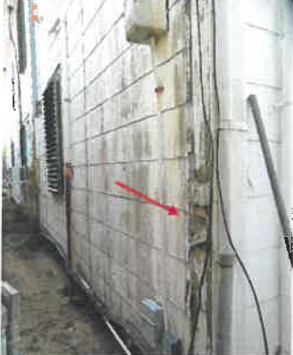
The corner trim on the house is damaged in spotted areas and the paint is gone leaving the wood unprotected.
