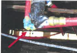
Water leak present on supply line along right side of house (in crawl space)
