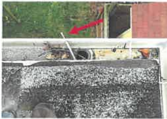
One of several popped gutter nails
