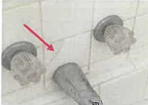
Tile crack on plumbing wall of downstairs apt bathroom.
