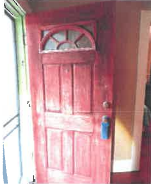
The original covering on the front door is wearing thin and needs to be reapplied to provide the door with adequate protection.
