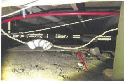
Crawl space pictures shows one of several electrical wires drooping and some wiring in direct contact with soil.
