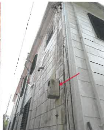
The meter which provides power to the sub panel is not weather sealed
