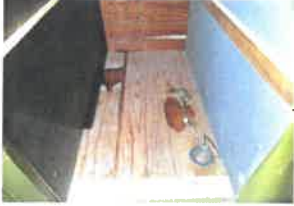
Water stains on linen closet floor.
