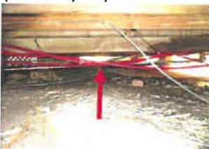
Sections of the pex water supply plumbing is not properly strapped and droops
