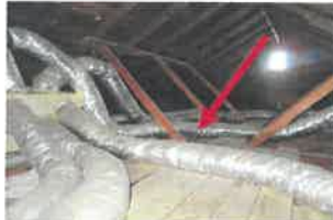
Ventilation ducts not suspended
