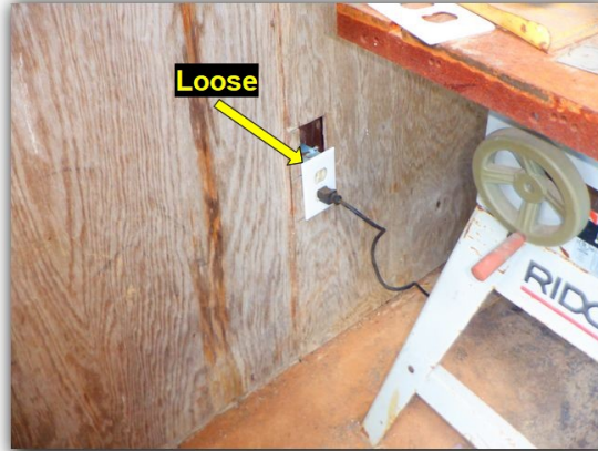
Observed multiple loose outlets.
