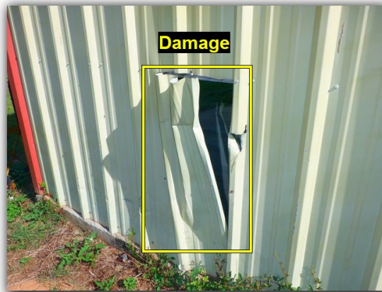
Observed damage to the exterior siding in one or more areas.
