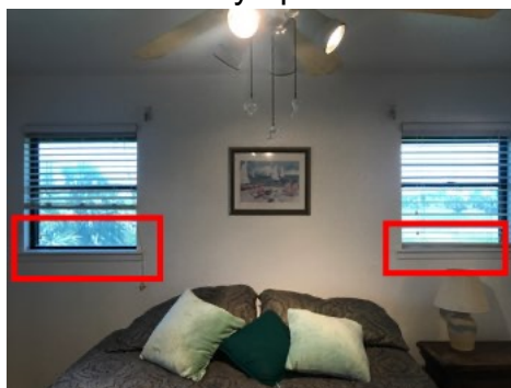
Bedroom 2: elevated moisture levels at window sills
