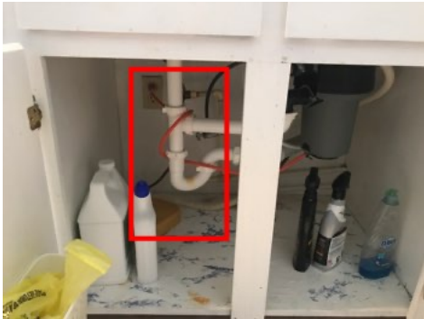
Kitchen: leak at drain
