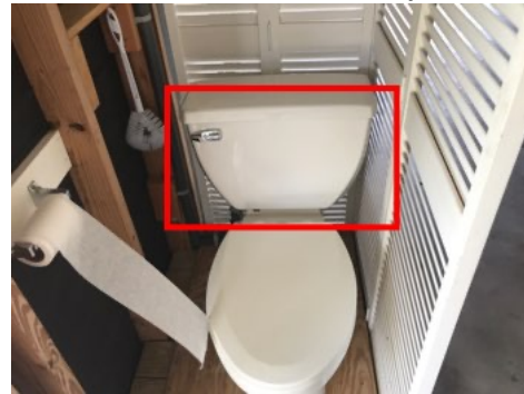
Garage: loose toilet tank
