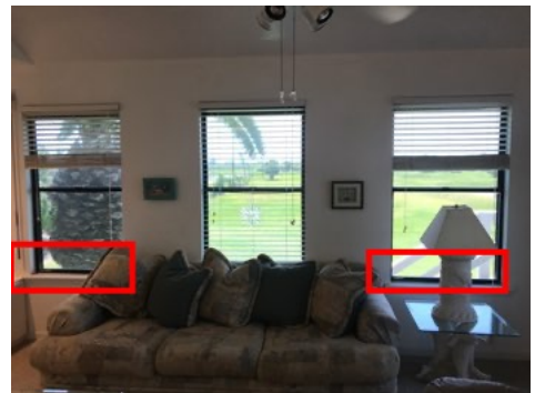
Living Room: elevated moisture levels at window sills
