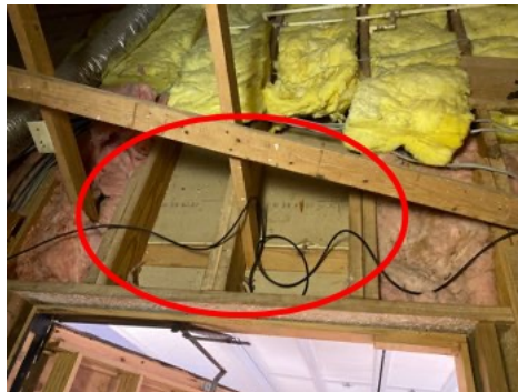
Insulation needs improvement
