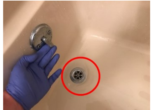
Bathroom 1: inoperable stopper
