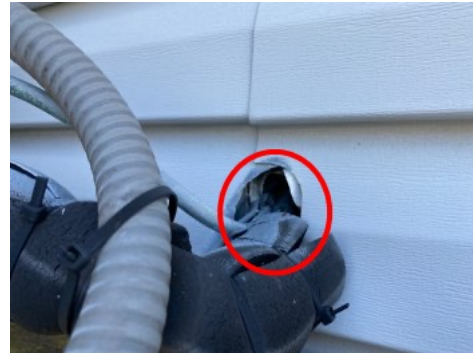
Left: hole in wall at ac lines
