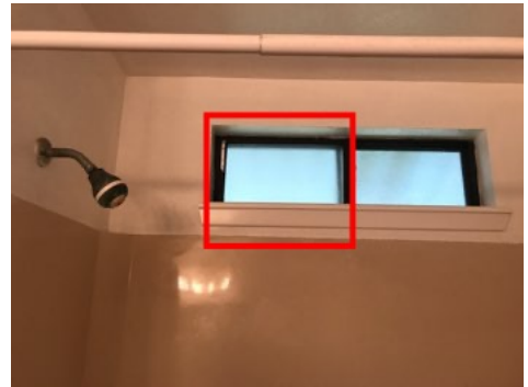
Bathroom 2: inoperable window
