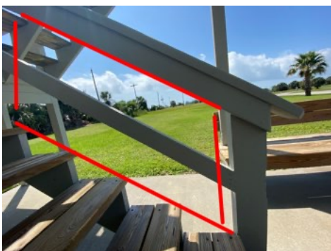
Handrail: Spindles more than 4 and 3/8" apart(climbable)
