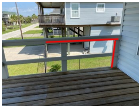
Balcony: guard rail loose
