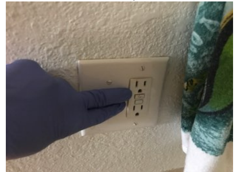
Bathroom 1: deteriorated GFCI, would not reset
