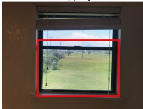
Bedroom 2: window would not stay open
