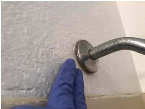
Caulk needed at bathroom wall protrusions
