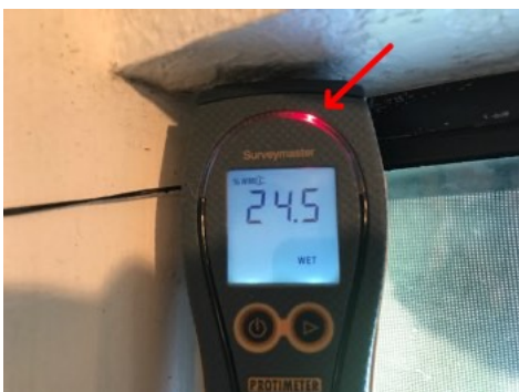
Living Room: elevated moisture levels at window sills confirmed
