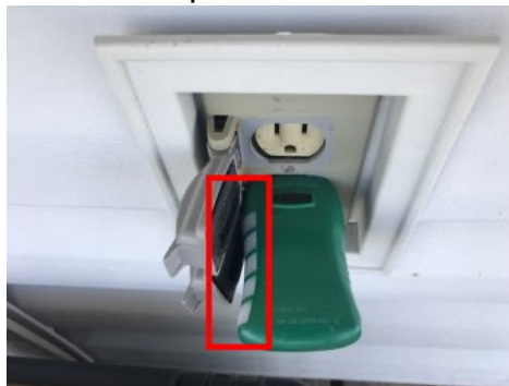
Front Porch: no power at outlet
