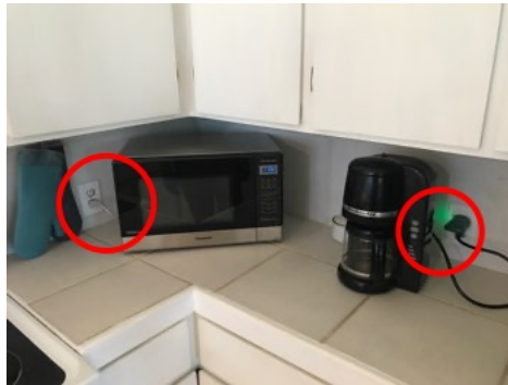
Kitchen: outlets not GFCI protected
