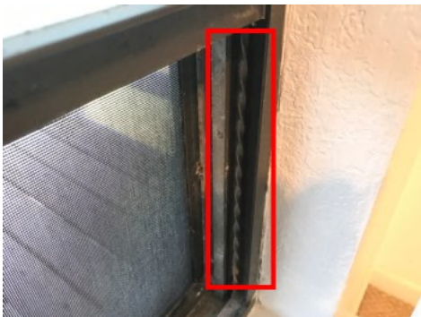
Dining Room: damaged hardware
