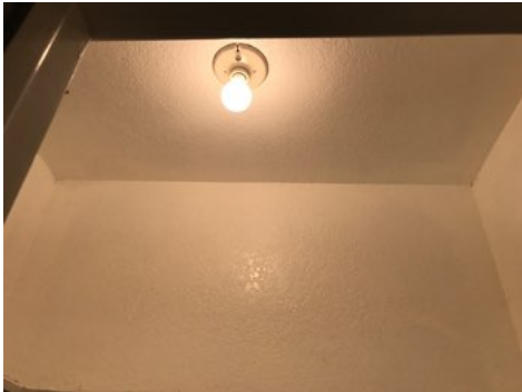
Closets: Globe missing
