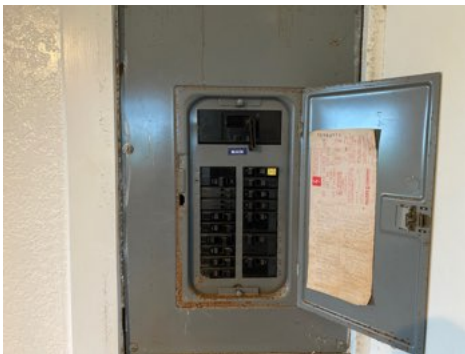
Bedroom 2: service panel
