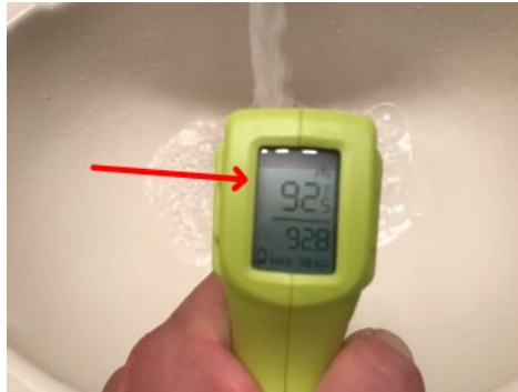
Hot water temperature
