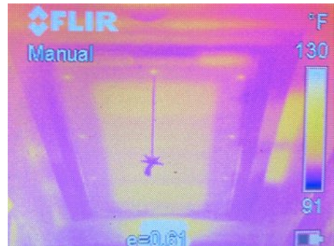
Thermal image of pull-down stairs lacking insulation
