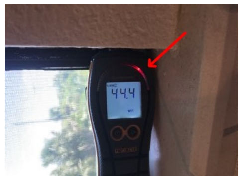
Bedroom 2: elevated moisture levels at window sills confirmed
