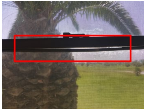
Living Room: loose weather stripping
