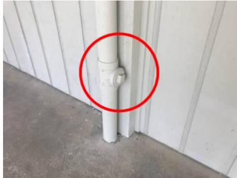
FYI: Main Cleanout located on the right
