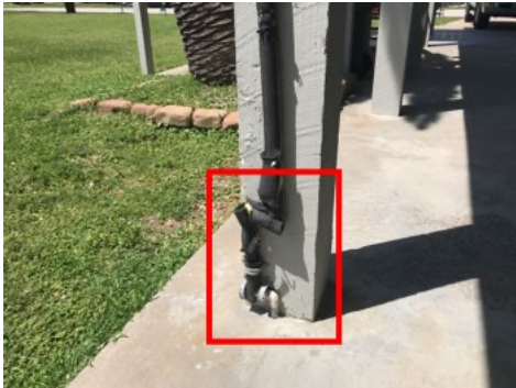
Right: Main Water Shutoff valve
