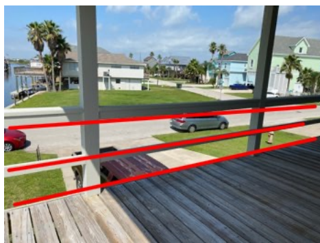
Guardrail: Spindles more than 4" apart(climbable)
