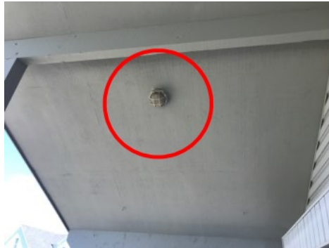
Front: inoperative fixture
