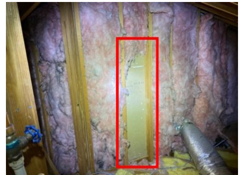
Front: fallen vertical insulation
