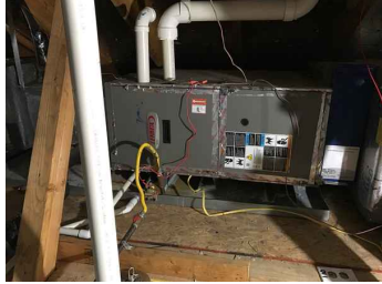
General Photos of HVAC Equipment:
