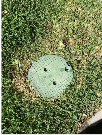
Vacuum Breaker/Backflow Preventer: Installed
