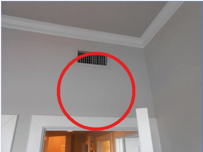
E. Item 1(Picture) Condensation stains here
