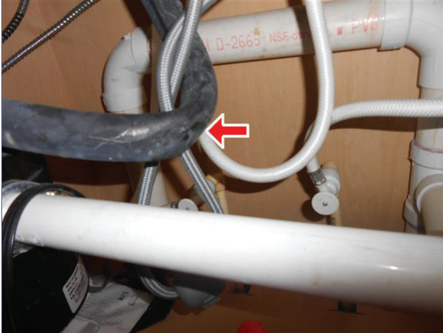
B. Item 1(Picture) Kinked drain line
