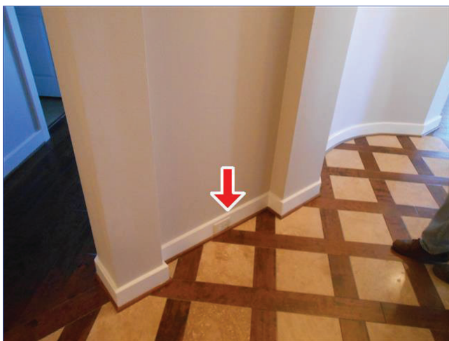
B. Item 4(Picture) Damaged power outlet cover
