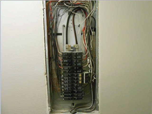
A. Item 1(Picture) View of the breaker panel open for inspection
