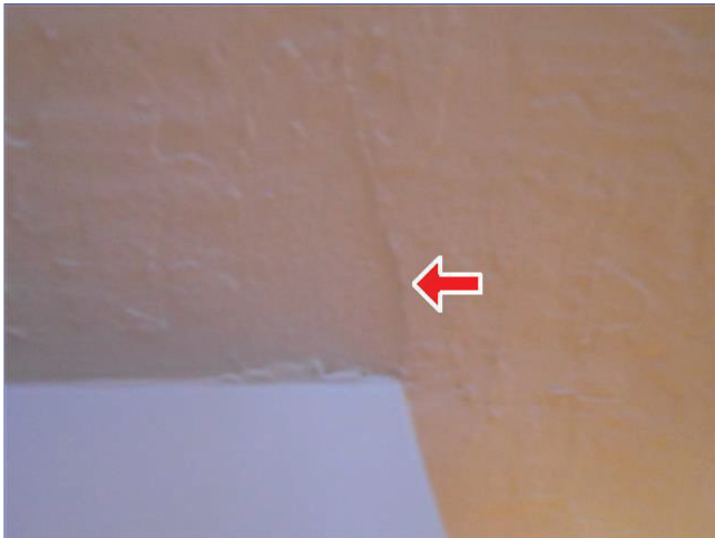
F. Item 1(Picture) Settling crack in hallway ceiling
