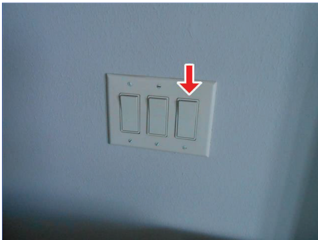
B. Item 6(Picture) Unidentified switch
