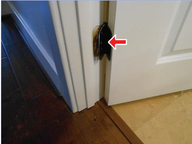
G. Item 3(Picture) loose lower door hinge
