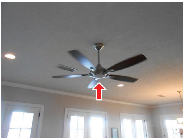
B. Item 2(Picture) This light failed to light with activation of the light switch.
