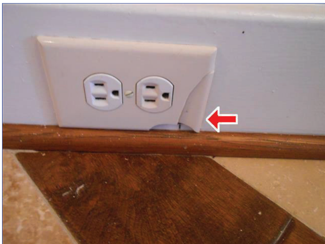
B. Item 3(Picture) Damaged power outlet cover
