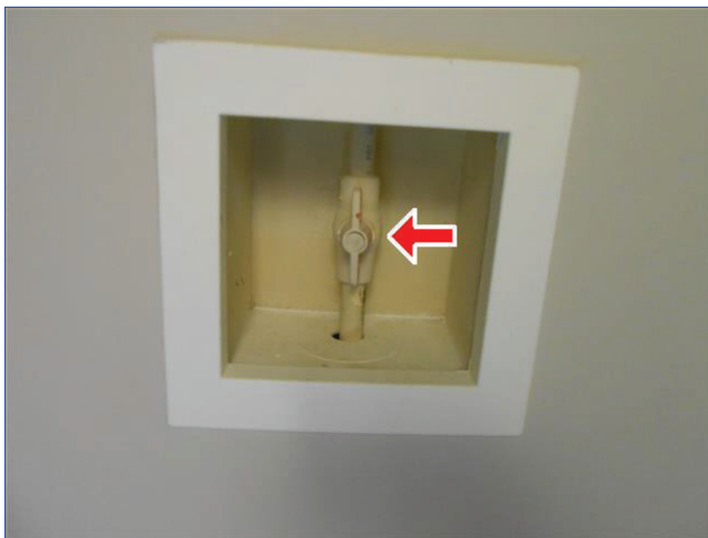
A. Item 1(Picture) Main water shut off in laundry room
