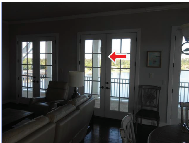
G. Item 2(Picture) Damaged door latch here
