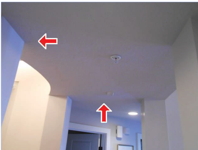
F. Item 3(Picture) Settling cracks here
