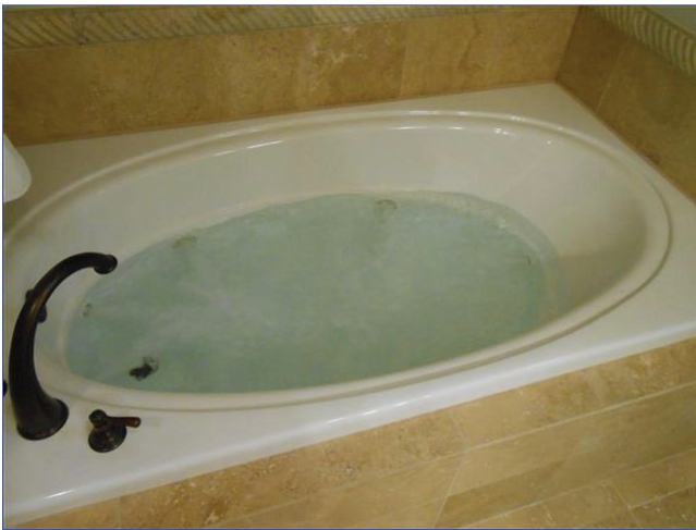
D. Item 2(Picture) View of the jetted tub functioning.
