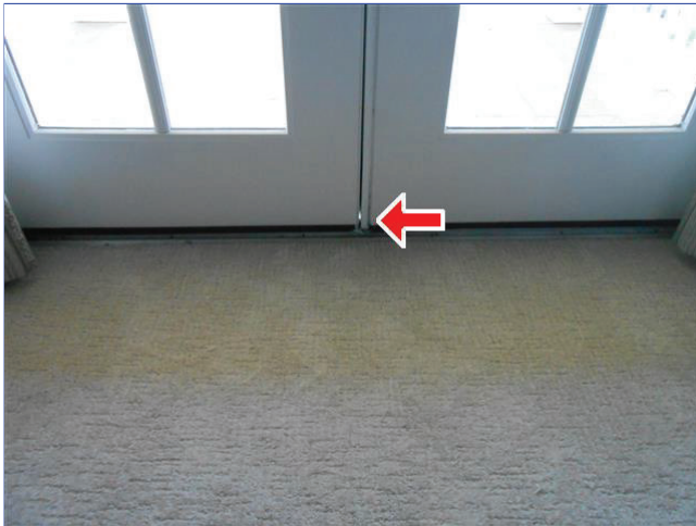
G. Item 4(Picture) The weather stripping needs attention here
