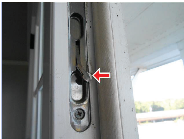
G. Item 1(Picture) Damaged door latch
