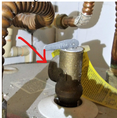
Missing safety valve piping.
