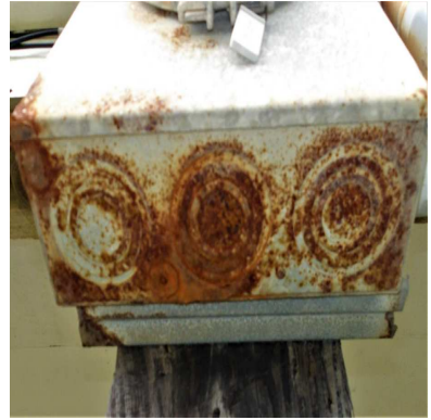
Heavy rust a meter panel.
