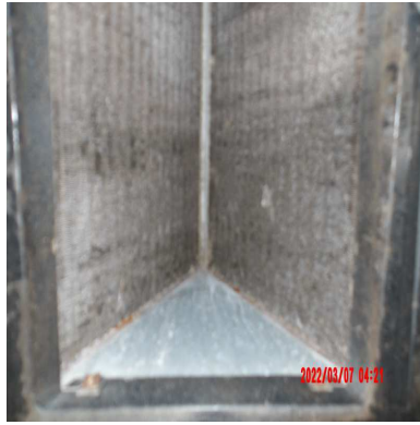
Evaporator coils dirty.
