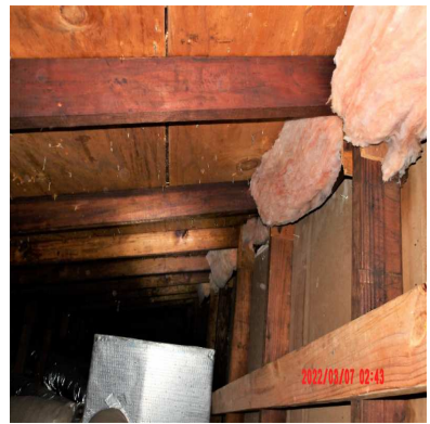
No insulated attic vertical walls.
