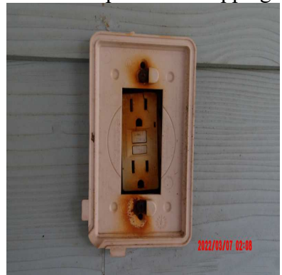
Loose GFCI receptacle in the wall.
