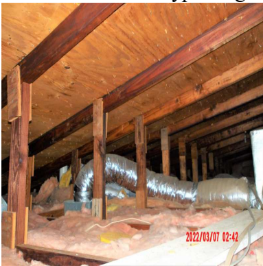
Ductwork not tied to the structure.
