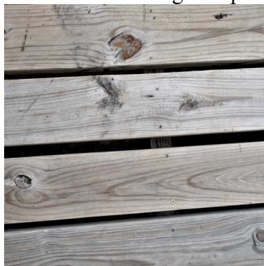
Wide gaps between of deck boards.
