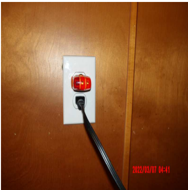
No GFCI protection.
