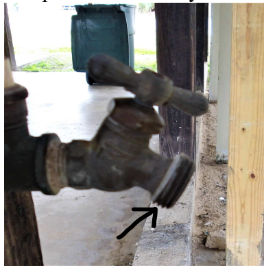
Missing back flow devices.
