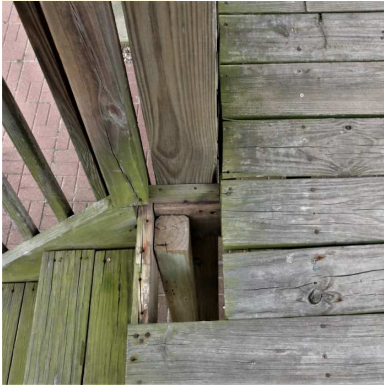
Missing deck step board.
