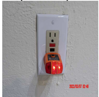
GFCI receptacle not tripping.
