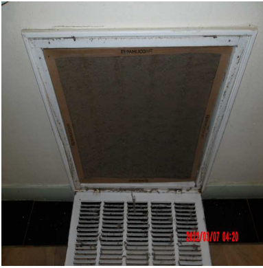
Both of the filters bypassing.
