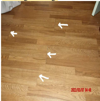
Flooring gaps sample.
