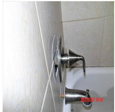
Fixture piping loose in the wall.
