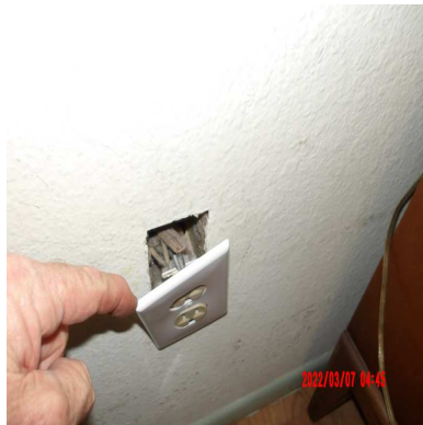
Loose receptacle in the wall.
