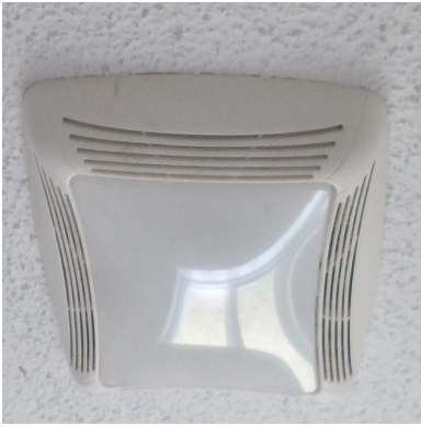
Bath vents not functioning.
