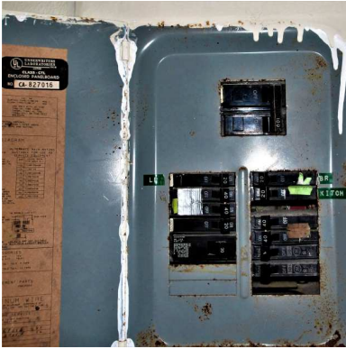
Sub panel stuck to the wall.
