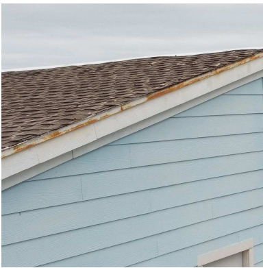
Rusted edge flashing.
