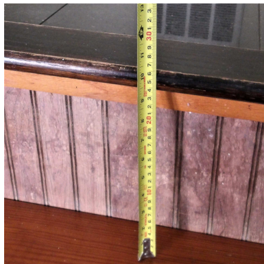
Hazardous riser height steps.
