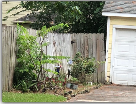
Observed damage section of the fence at one or more locations
