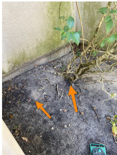
Front of home, slopes towards the foundation in the landscaping
