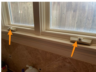
Kitchen, missing handles to crank window open
