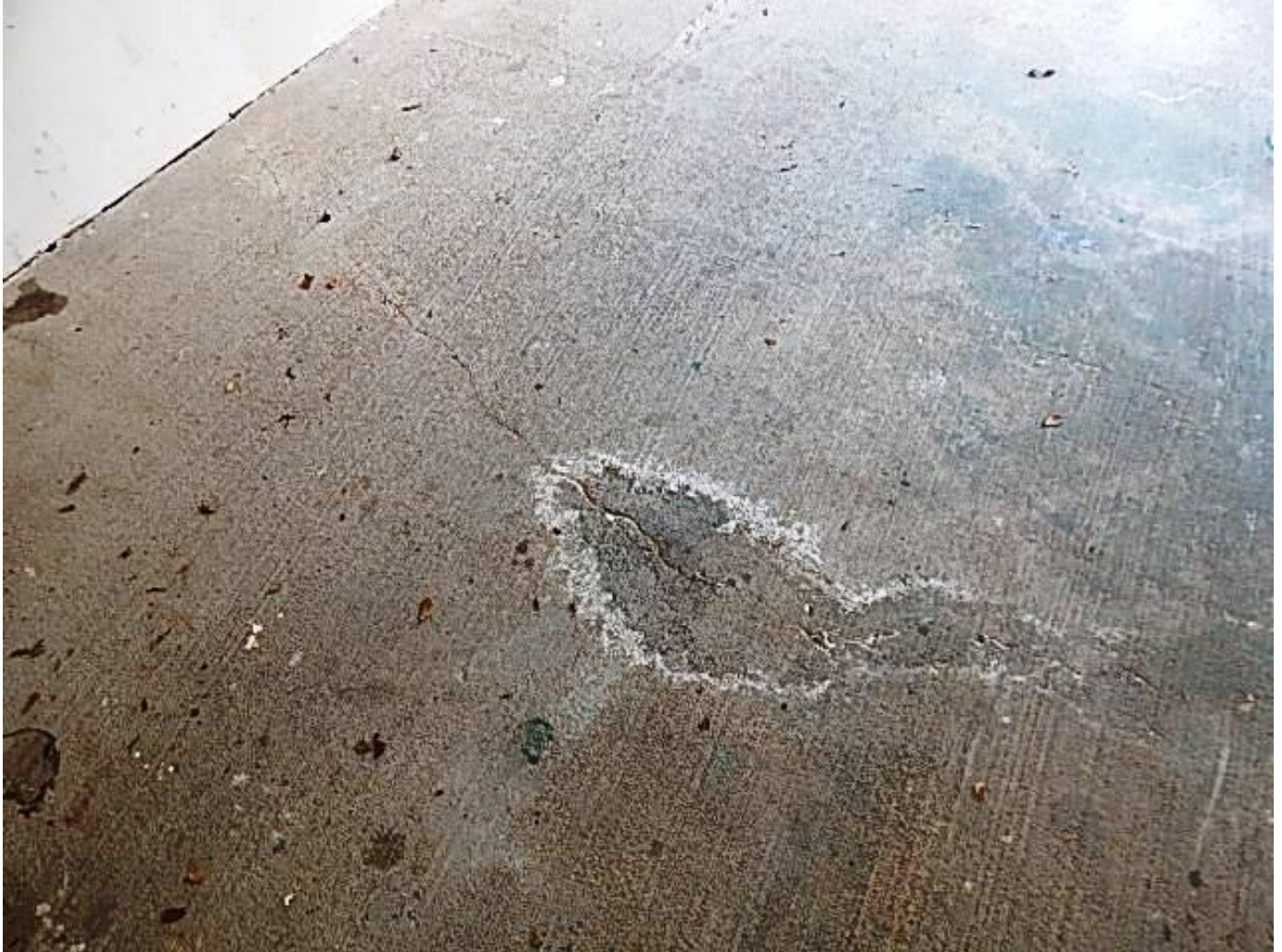
Cracks in the garage concrete.
