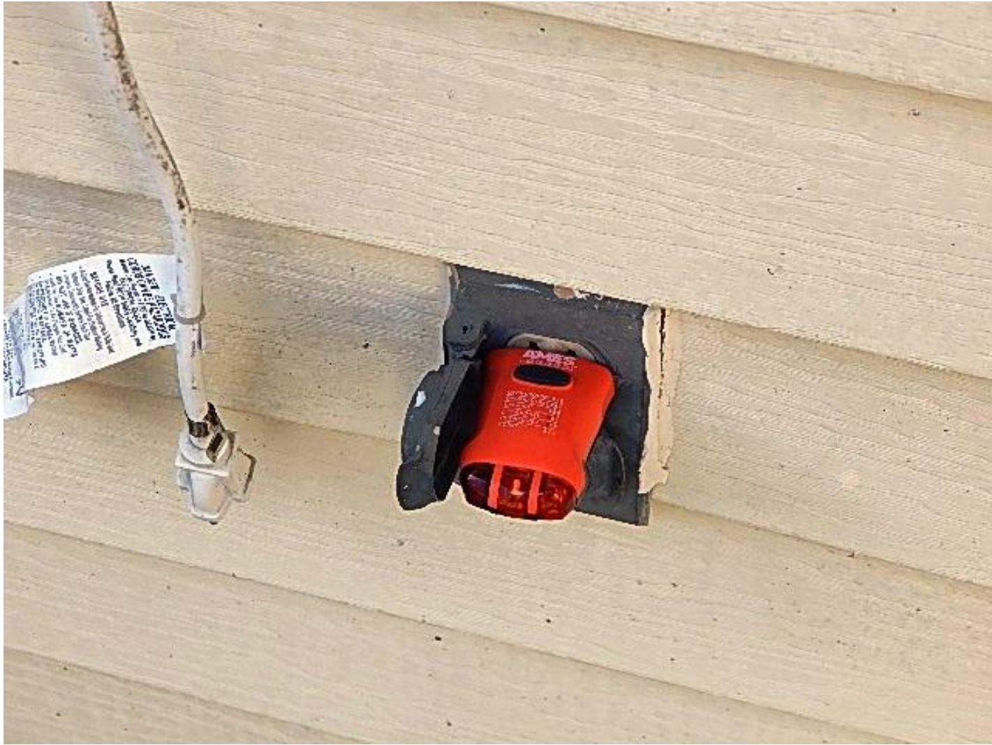
Not GFCI protected.
