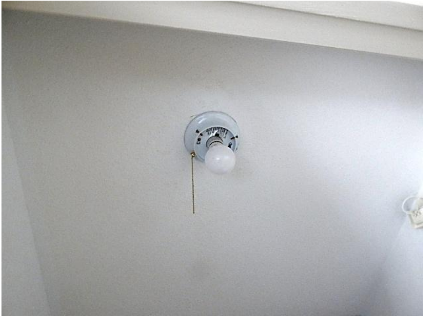
Missing globe cover.
