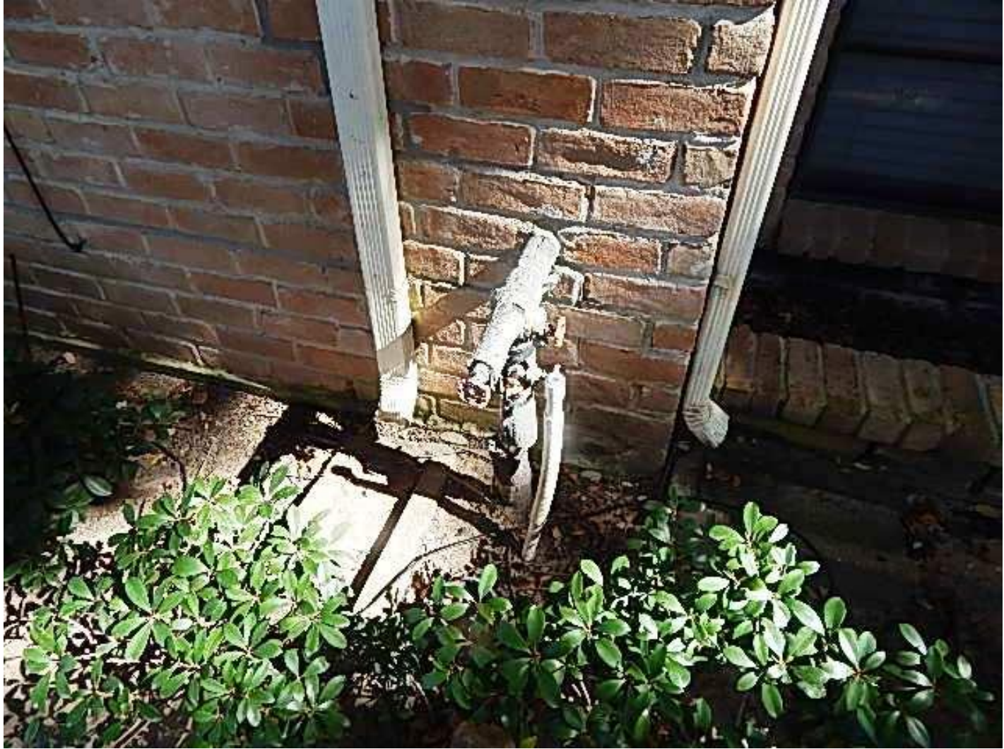
Main shut off.
