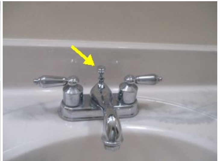
Non functioning drain stop pull lever at right sink in addition bathroom.
