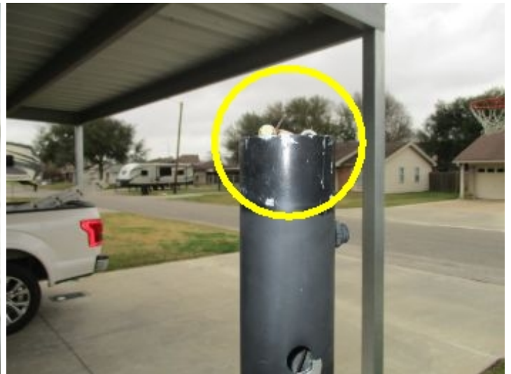
Missing fixture atop pole light in front yard.
