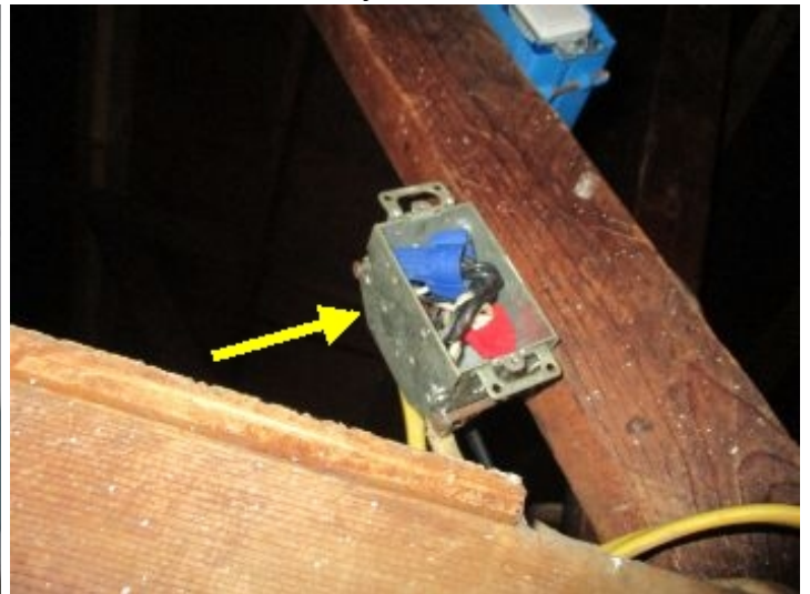
Replace missing cover plates at receptacles and or junction boxes.
