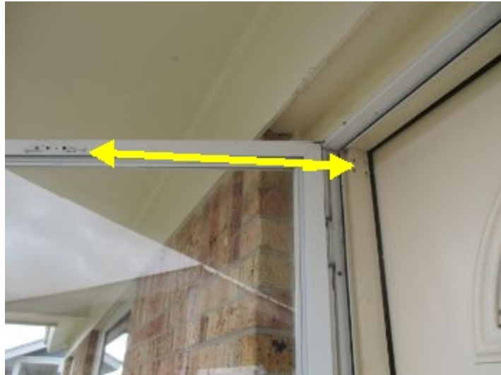
Missing hydraulic door closure at front storm door.
