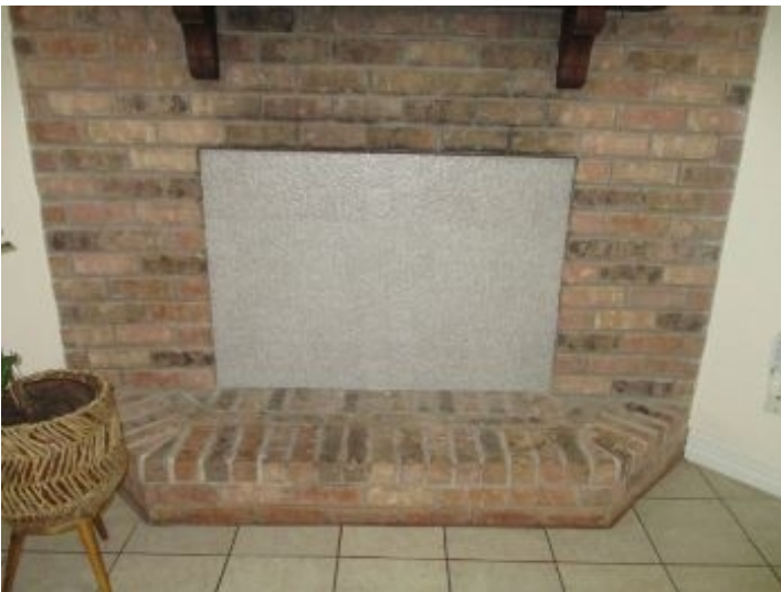
Unable to remove large tiles covering at ft of firebox to view firebox.
