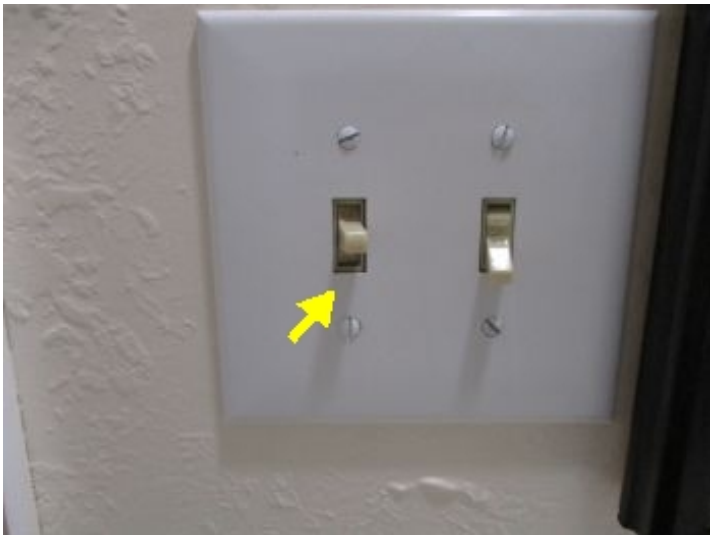
Worn and loose wall switch in rear addition bathroom.
