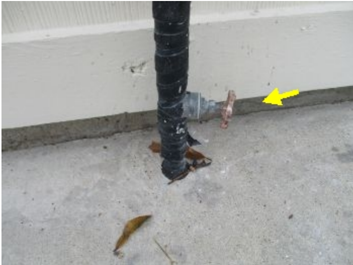
Main shut off valve
