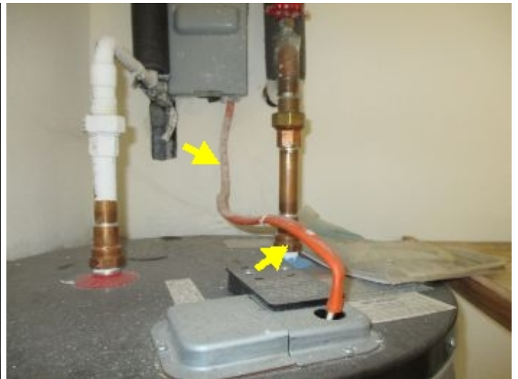
The exposed romex (electrical wire) atop water heater is required to be in protective conduit for safety reasons.
