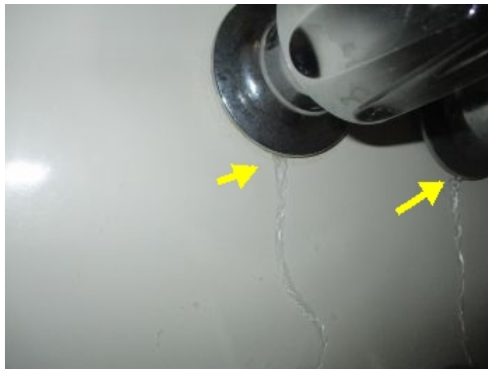
Leak at tub / shower fixtures in addition bathroom.
