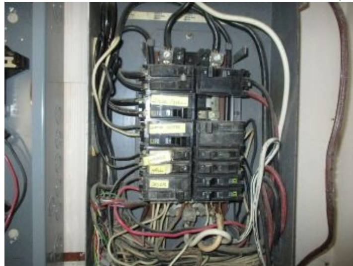
View of wiring to breakers in right panel
