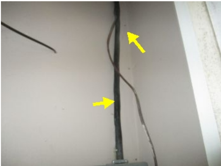
The exposed romex (electrical wire) in the closet of rear addition above panel is required to be in protective conduit for safety reasons.
