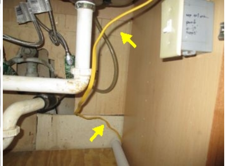
The exposed romex (electrical wire) under kitchen sink is required to be in protective conduit for safety reasons.
