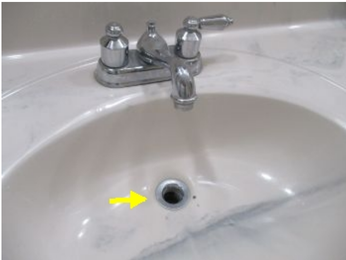
Missing drain stop at at left sink in addition bathroom.
