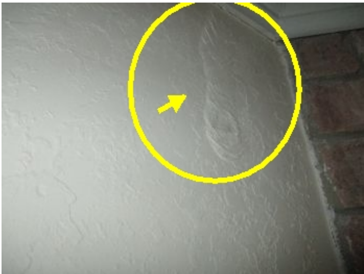
Observed what appears to be water damage to interior wall in the addition den on wall to the left of fireplace.
