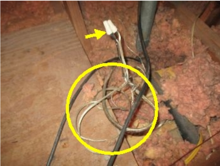
Exposed wire splice in attic at kitchen sink pendant light is required be in protected junction box for safety reasons. Note use of extension cord for permanent wiring to this light.
