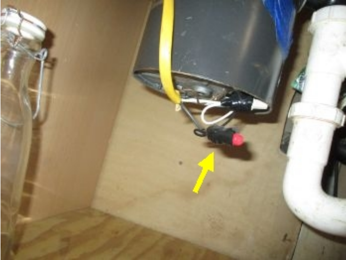
Exposed wire splice at disposal is required be in protected junction box for safety reasons.
