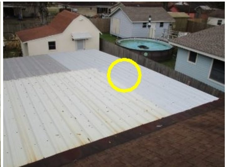
No through roof or to exterior flue.
