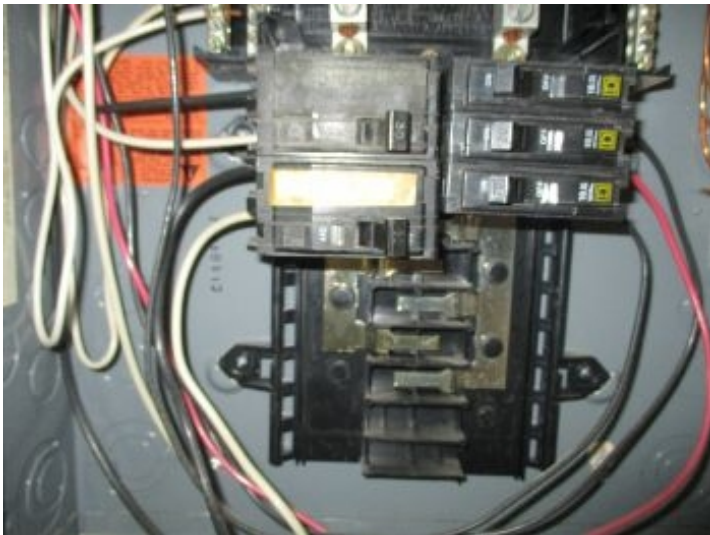
View of wiring to breakers in left panel
