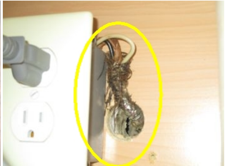
worn insulation on romex to receptacle in cabinet above microwave.
