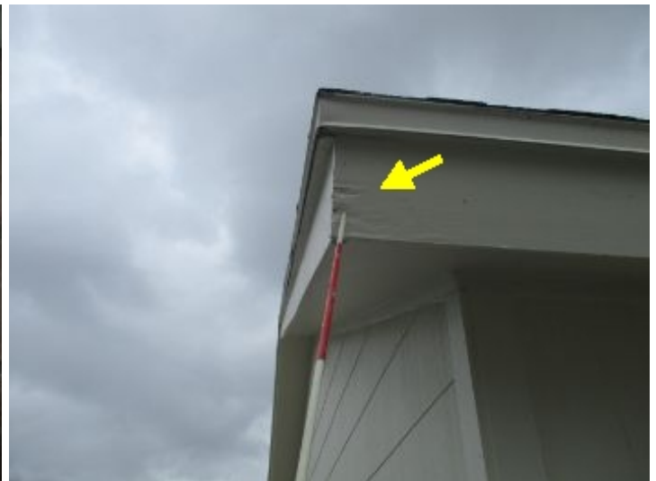
Rot to rear right corner eave fascia trim board.
