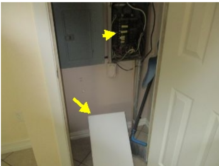
Incorrect cover plate used at right panel in addition closet. Original cover plate is removed and hinges are damaged.
