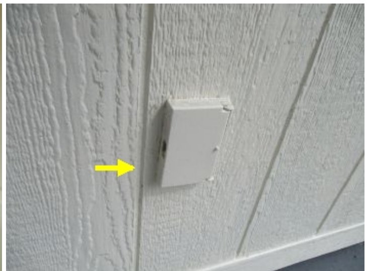
Rear porch receptacle cover is painted shut, unable to open.
