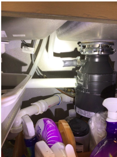
General Photos of Range Hood/Exhaust Systems:
