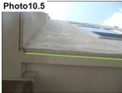
Reglet Vent Installed / No Modification
