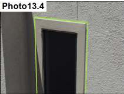
Window Accent/Stucco Termination / Seal
