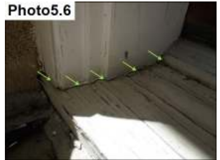
Door Sealant Separation / Seal
