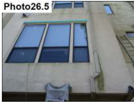
Relief Missing / Install
