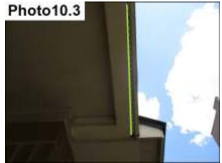
Reglet Vent Installed / No Modification
