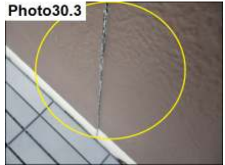
Cement Fiber Panels Separated / Re-Fasten and Seal
