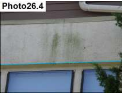
Relief Missing / Install
