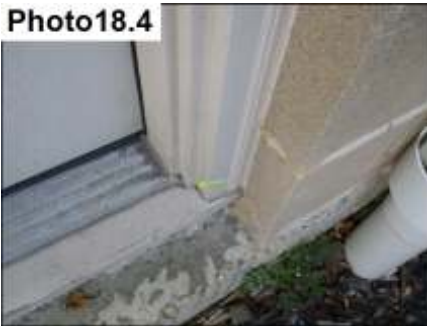
Door Sealant Separation / Seal
