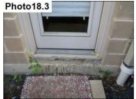
Door Sealant Separation / Seal
