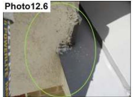
Roof Diverter Flashing / Seal
