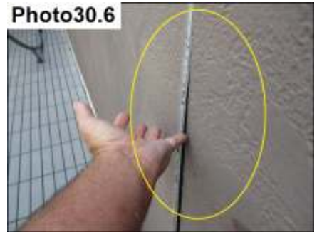
Cement Fiber Panels Separated / Re-Fasten and Seal
