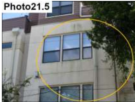
Mildew Noted & Runoff Stains / Clean Aesthetic Concern
