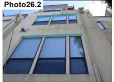
Relief Missing / Install
