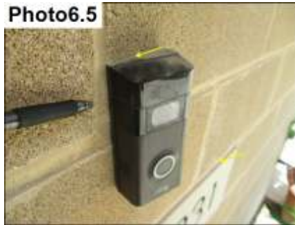
Penetration Sealants / Seal
