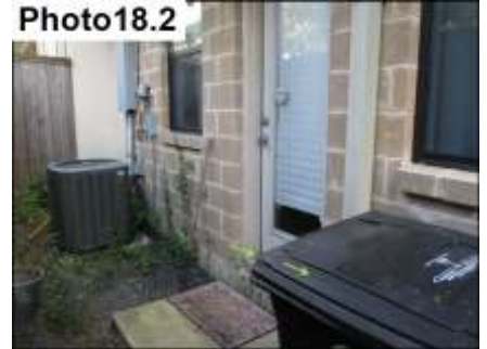
Door Sealant Separation / Seal
