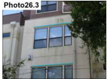
Relief Missing / Install
