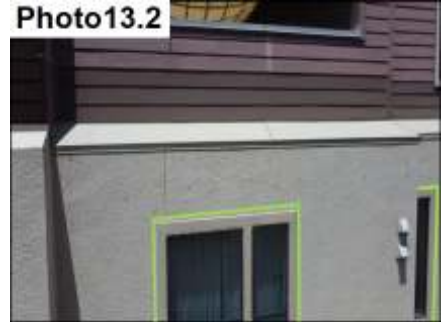
Window Accent/Stucco Termination / Seal
