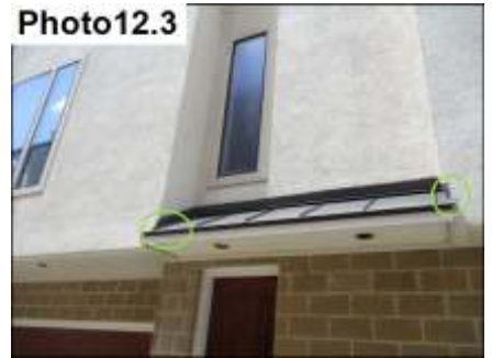
Roof Diverter Flashing / Seal
