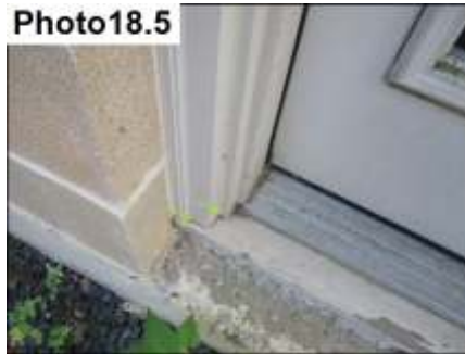
Door Sealant Separation / Seal
