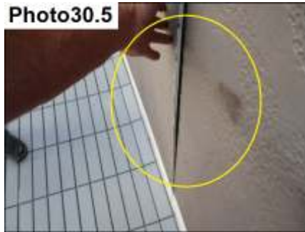
Cement Fiber Panels Separated / Re-Fasten and Seal
