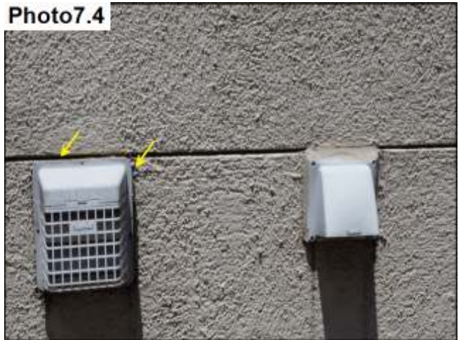
Penetration Sealants / Seal
