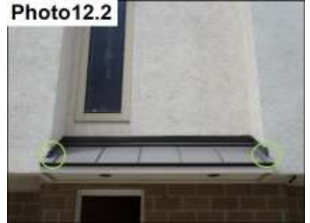
Roof Diverter Flashing / Seal
