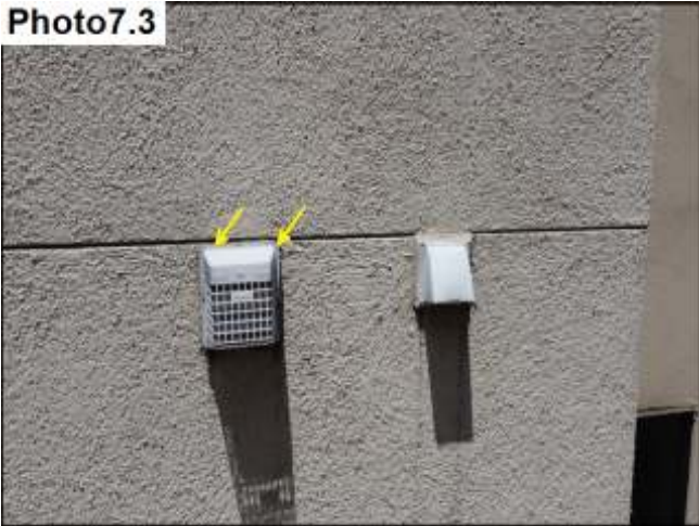
Penetration Sealants / Seal
