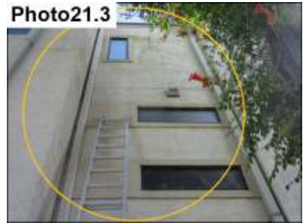
Mildew Noted & Runoff Stains / Clean Aesthetic Concern
