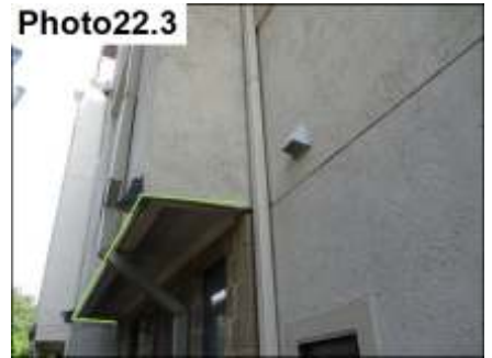
Reglet Vent Installed / No Modification
