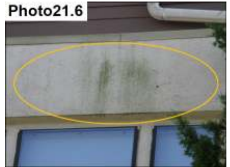
Mildew Noted & Runoff Stains / Clean Aesthetic Concern
