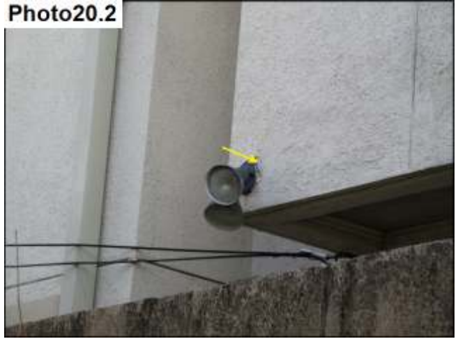
Penetration Sealants / Seal
