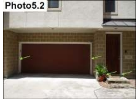
Door Sealant Separation / Seal
