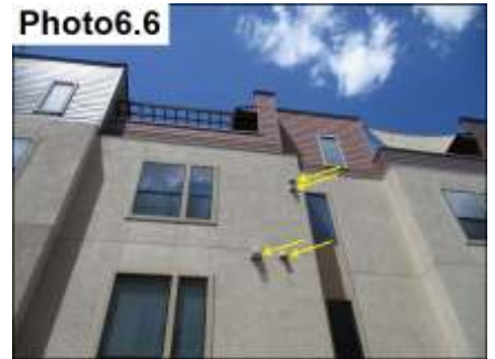
Penetration Sealants / Seal
