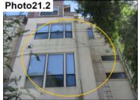
Mildew Noted & Runoff Stains / Clean Aesthetic Concern
