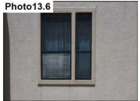
Window Accent/Stucco Termination / Seal
