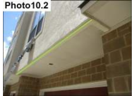
Reglet Vent Installed / No Modification
