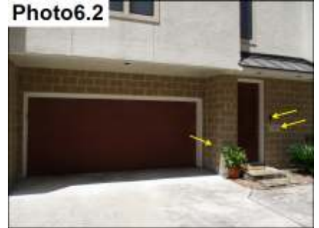
Penetration Sealants / Seal
