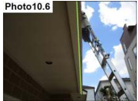
Reglet Vent Installed / No Modification
