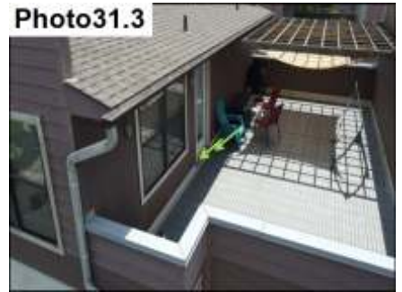
Door Sealant Separation / Seal
