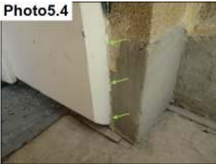
Door Sealant Separation / Seal
