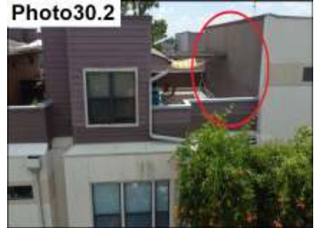
Cement Fiber Panels Separated / Re-Fasten and Seal
