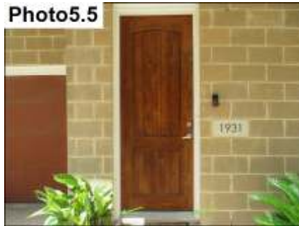
Door Sealant Separation / Seal
