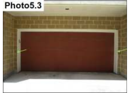
Door Sealant Separation / Seal
