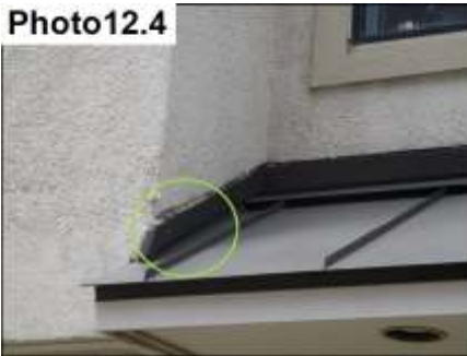
Roof Diverter Flashing / Seal
