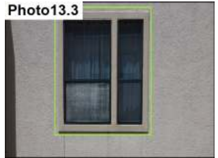
Window Accent/Stucco Termination / Seal
