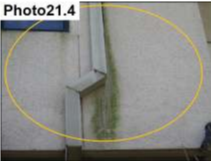
Mildew Noted & Runoff Stains / Clean Aesthetic Concern
