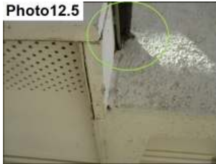
Roof Diverter Flashing / Seal
