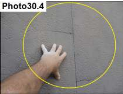
Cement Fiber Panels Separated / Re-Fasten and Seal
