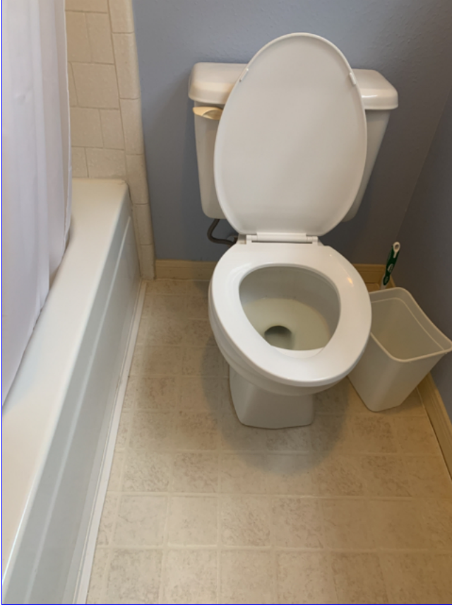
A. Photo 1(Picture) The toilet is loose at floor at the bath. Repairs may involve re-setting the toilet on a new wax seal. I recommend a qualified licensed plumber repair or correct as needed.
