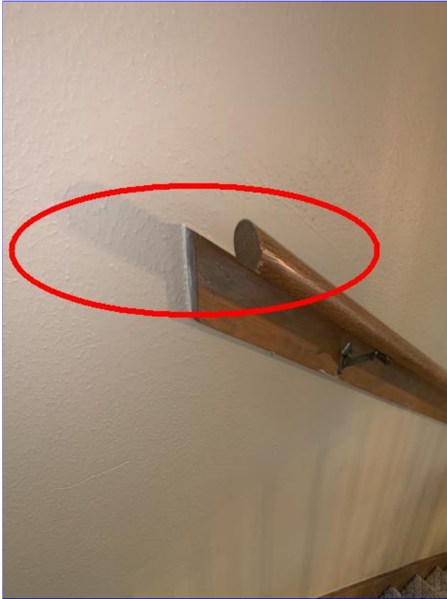
I. Photo 1(Picture) The handrail ends do not return to the walls. Open handrail ends can catch on clothes causing safety concerns on stairs.
