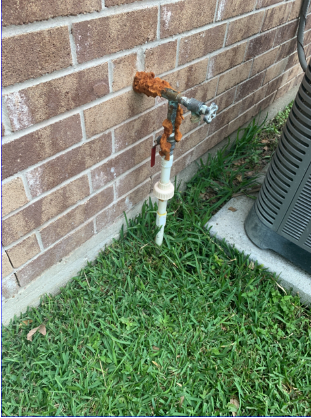
A. Photo 4(Picture) The main water supply line at the exterior, is not properly protected from freezing.
