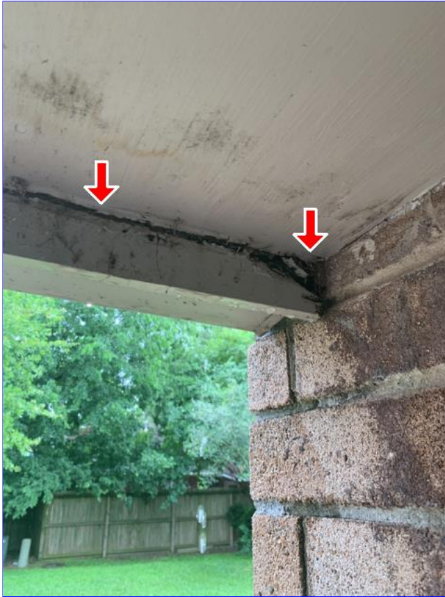
E. Photo 4(Picture) Areas of wood rot were observed on the soffit fascia boards.
