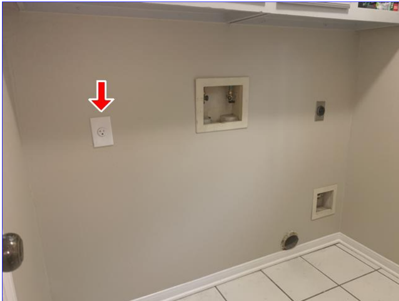
B. Photo 1(Picture) In the laundry room, there's only one receptacle for both the washer and gas dryer.
