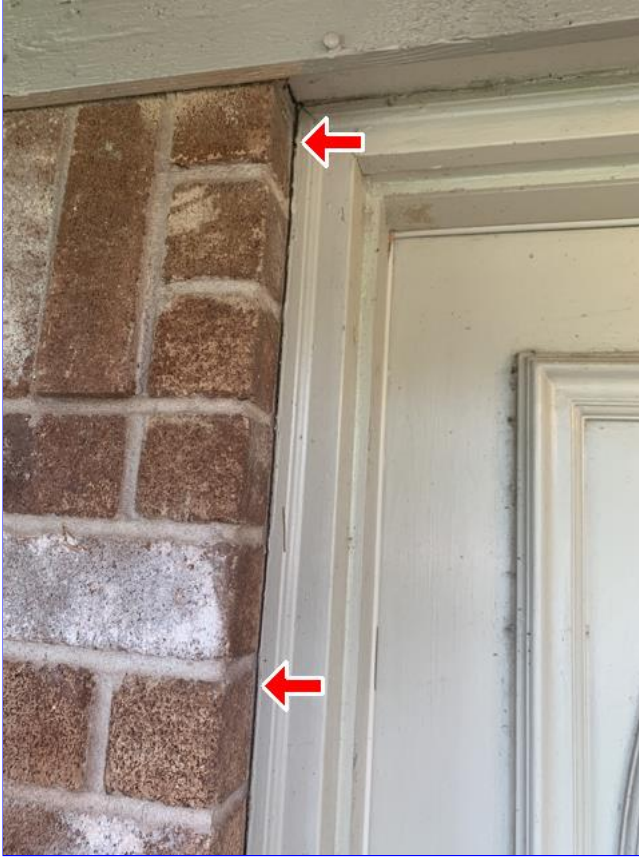
E. Photo 3(Picture) Areas were observed, where the brick, siding and/or trim needs to be resealed.
