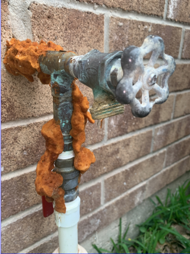
A. Photo 3(Picture) On the right side of the home, the hose bib has a constant leak.
