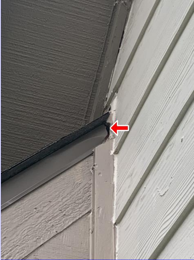
E. Photo 1(Picture) Areas were observed, where the brick, siding and/or trim needs to be resealed.
