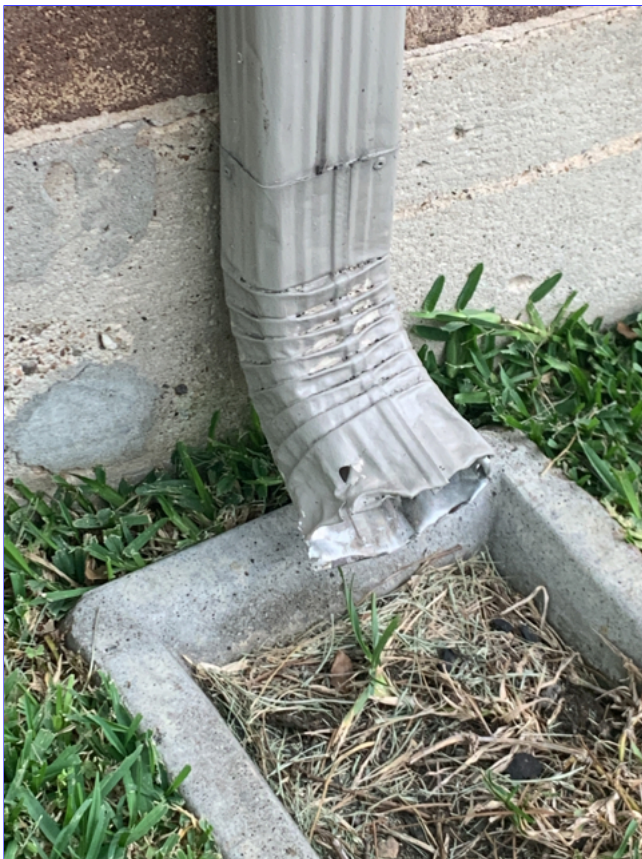
B. Photo 1(Picture) Several damaged downspout turn outs were observed.
