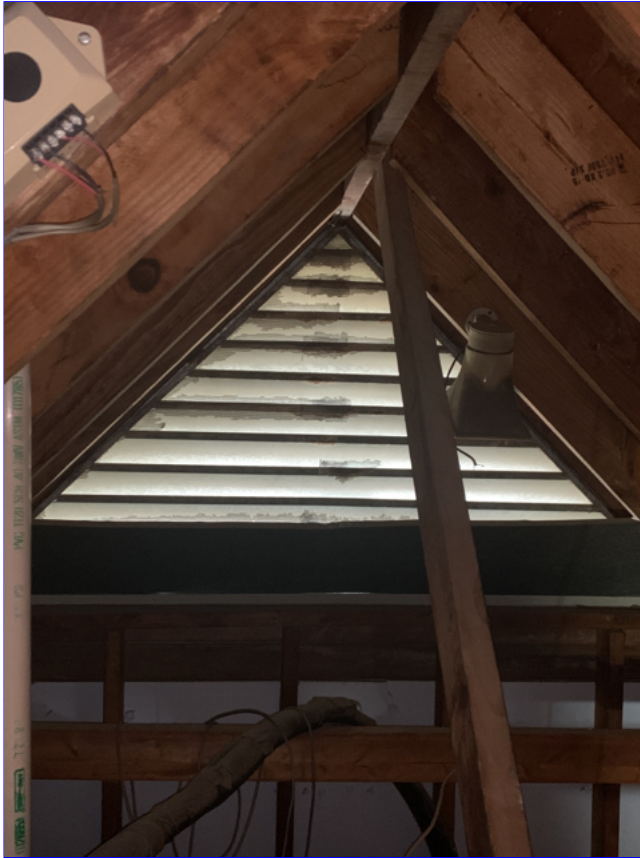
D. Photo 1(Picture) The gable vent screens have deteriorated. Recommend replacement.
