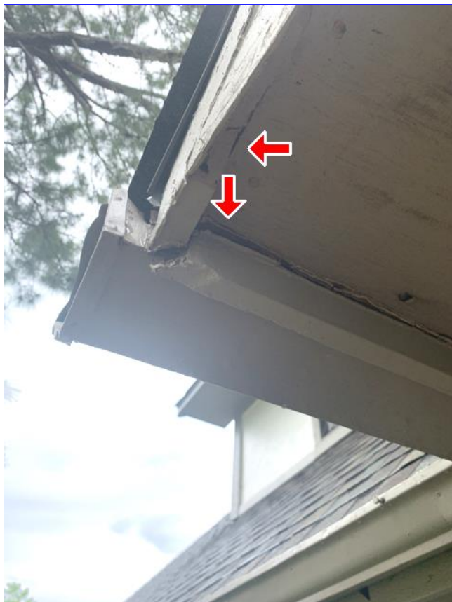
E. Photo 5(Picture) Areas of wood rot were observed on the soffit fascia boards.
