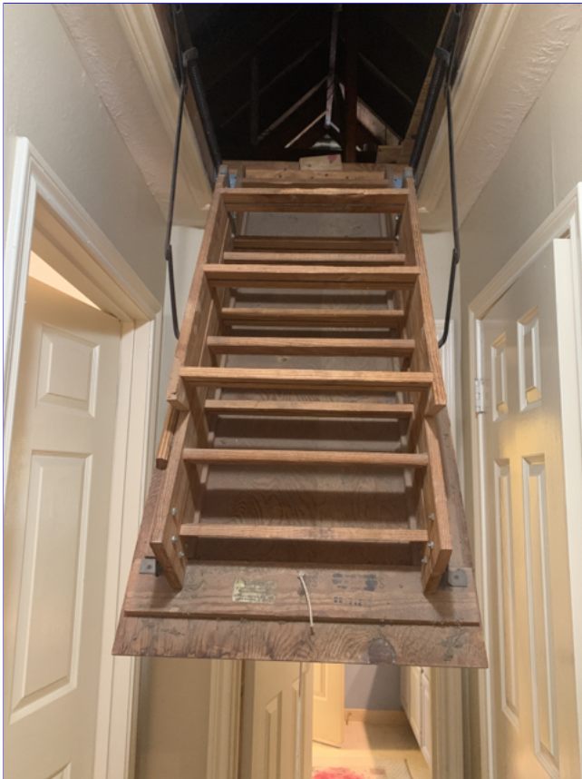
G. Photo 1(Picture) Note: The attic access door (pull down stairs), is not insulated or weather stripped. This door separates a non-conditioned space (attic) from the interior conditioned space and should be insulated and weather stripped for energy efficiency reasons.
