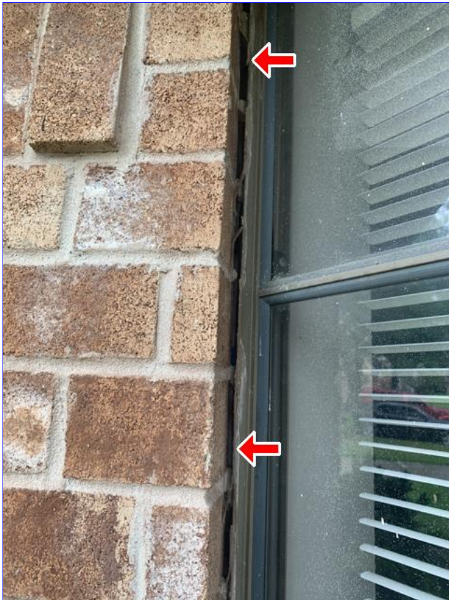
H. Photo 2(Picture) The perimeter sealant, has failed on some windows.
