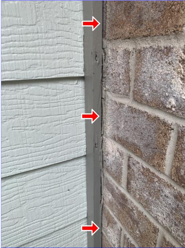
E. Photo 2(Picture) Areas were observed, where the brick, siding and/or trim needs to be resealed.
