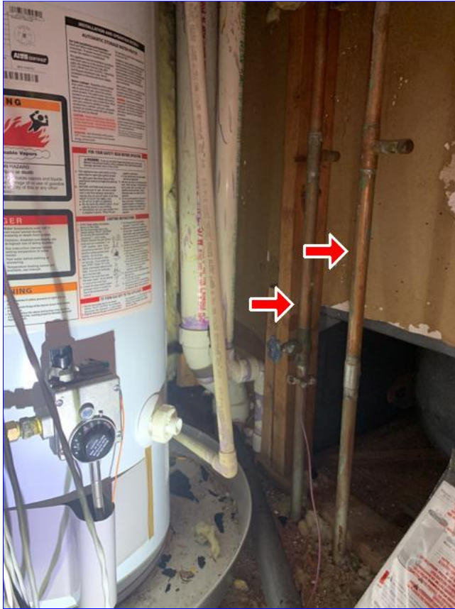
A. Photo 5(Picture) Exposed water pipes observed in the attic space are not properly protected from freezing. Water pipes should be buried under the insulation or properly wrapped to prevent breakage from freezing.
