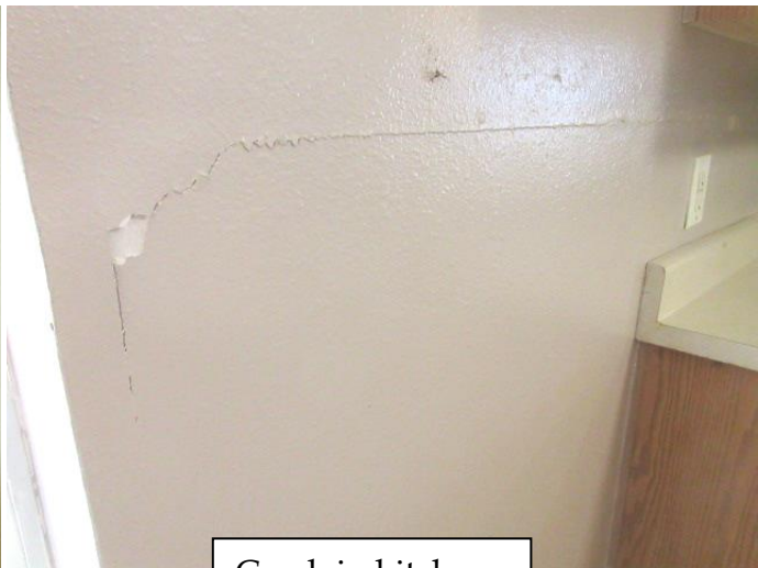
Crack in kitchen
