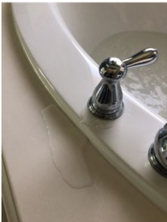
The master tub fixture is leaking. Suggest a licensed professional repair.
