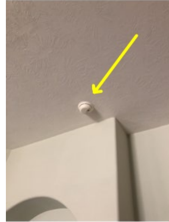
The smoke detector in front of the master bedroom does not operate when tested.
