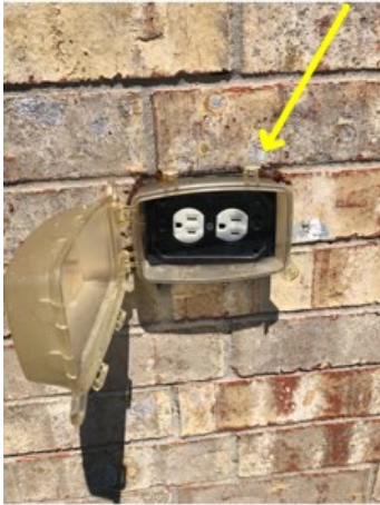
Receptacle by the AC unit is loose and needs to be repaired.
