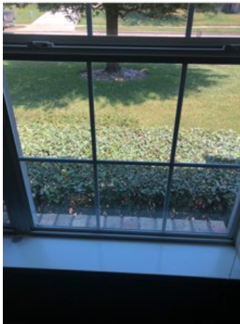
Some window screens are missing.
