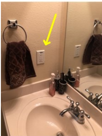
The GFCI receptacle for all bathrooms is in the guest bath.
