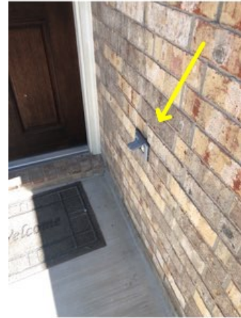
The receptacle outside the front door is not GFCI protected.
