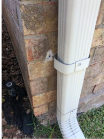
The downspout on the right side of the house is loose.
