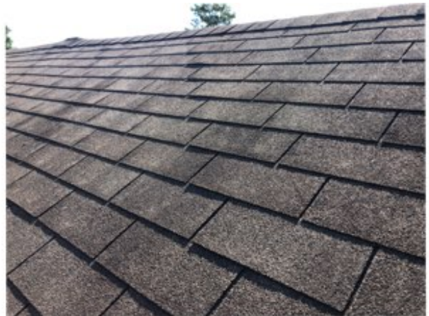
The shingles are starting to lift and come loose. The shingles are nearing the end of their life cycle.
