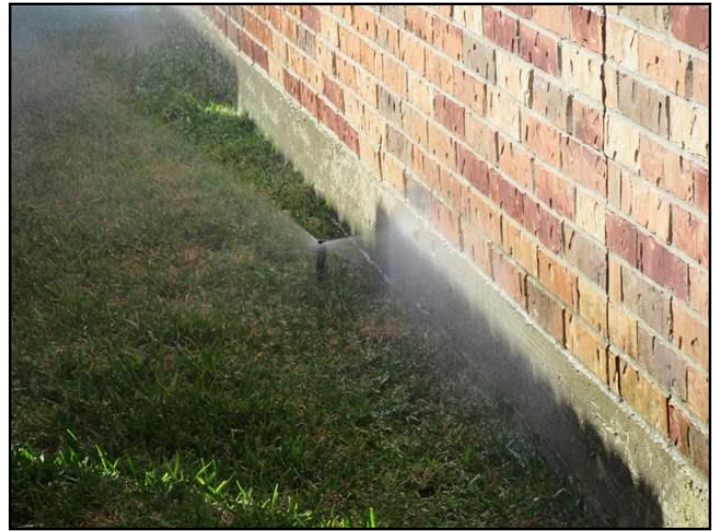
31. Sprinkler heads should be adjusted to spray...
