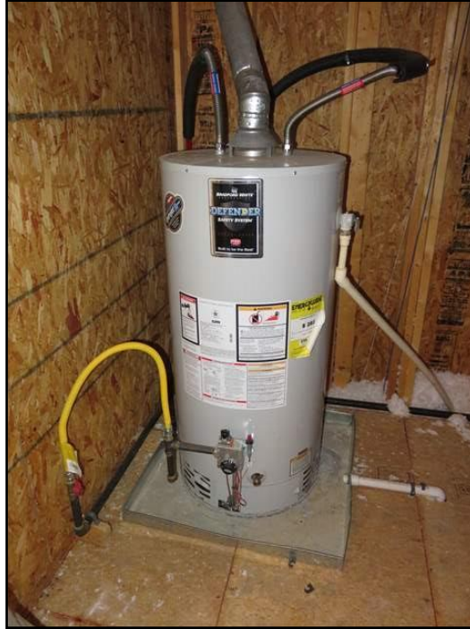
15. General view of water heater.
