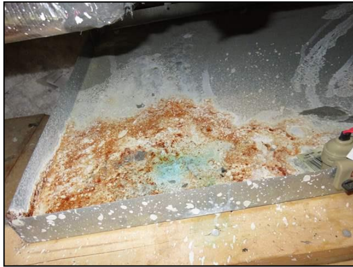
12. Rusting in the evaporator condensate...
