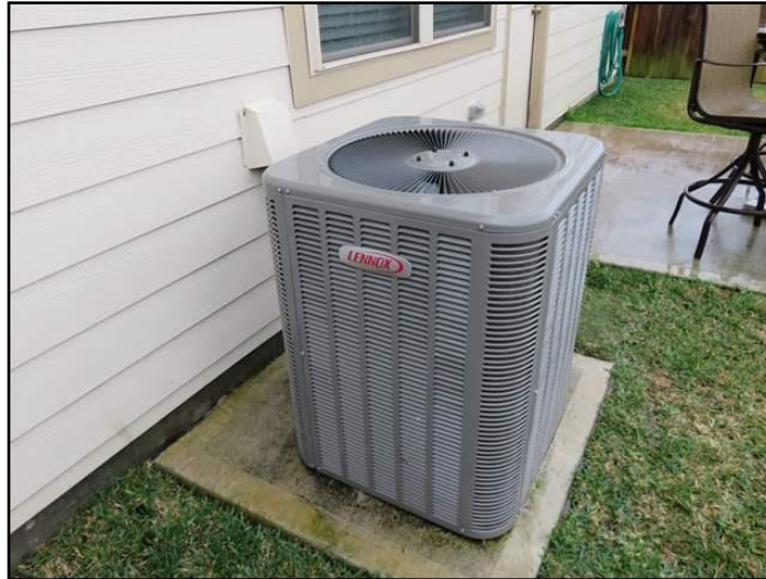
11. General view of air conditioner...
