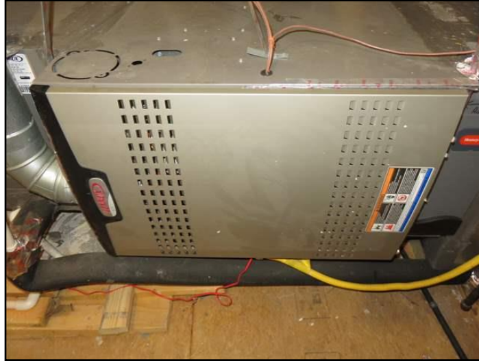
10. General view of heating system.
