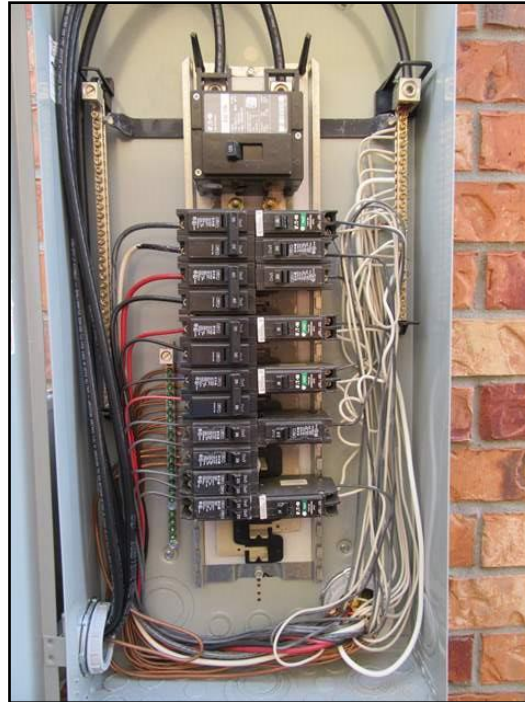
9. General view of electrical panel(s).
