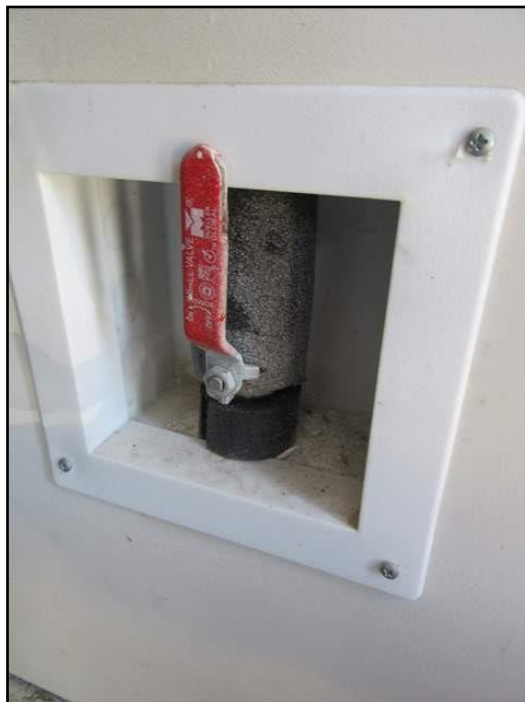
16. View of interior water shut off location.
