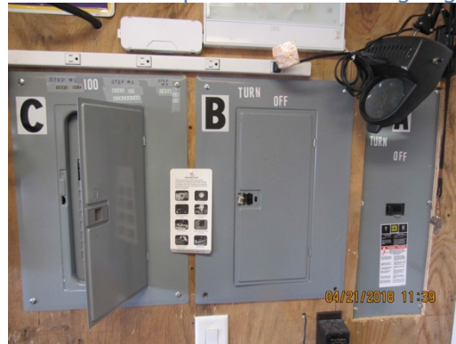
3-Interior Sub panels boxes at the garage.
