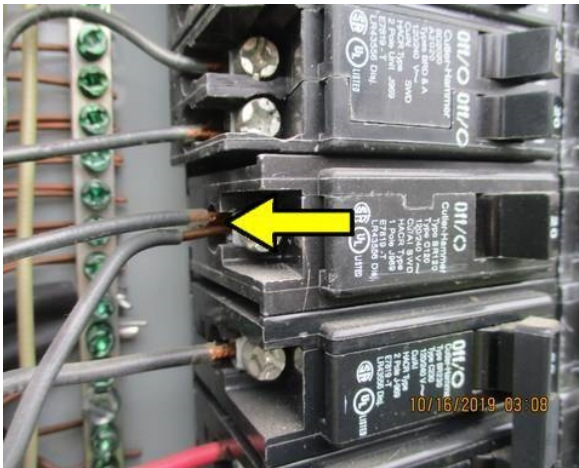
Double tapped breaker
