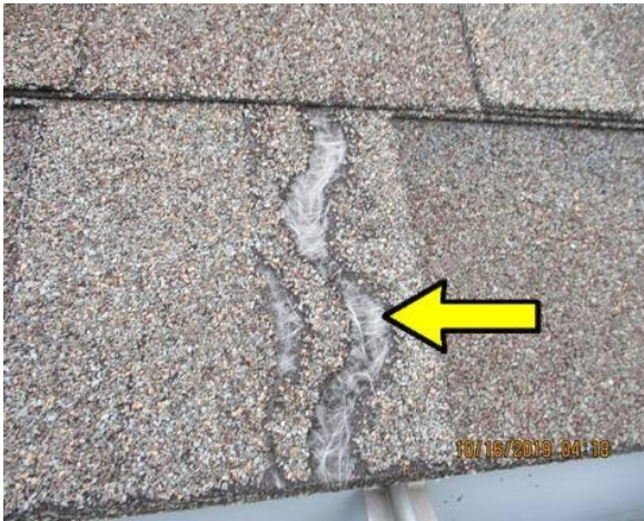
Damaged shingle above front porch
