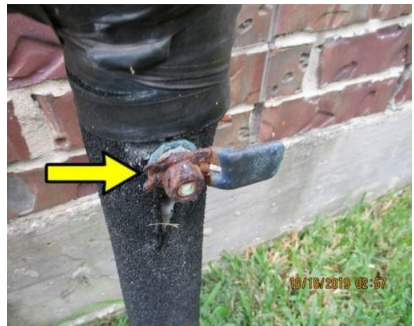
Handle is broke on backflow preventer valve
