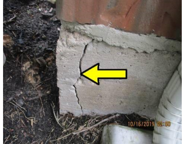
Spalled at front right
