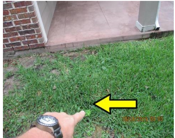
Fill hole at right of back porch
