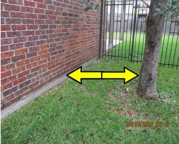
Tree in close proximity
