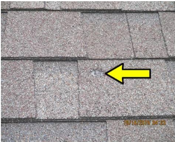
Possible hail damage at back slope
