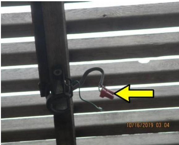
Secure exposed wire at back patio cover
