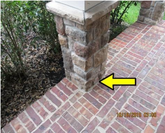
Missing weep holes at front porch column
