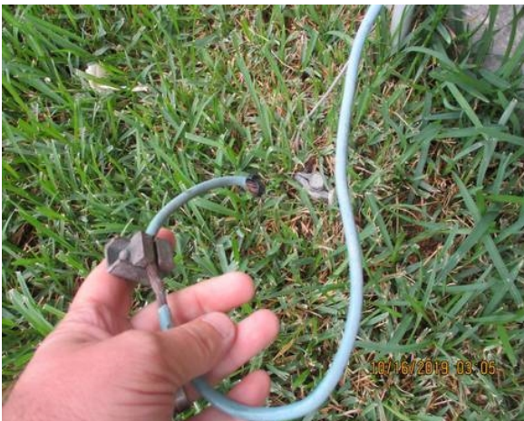
Ground wire is not attached
