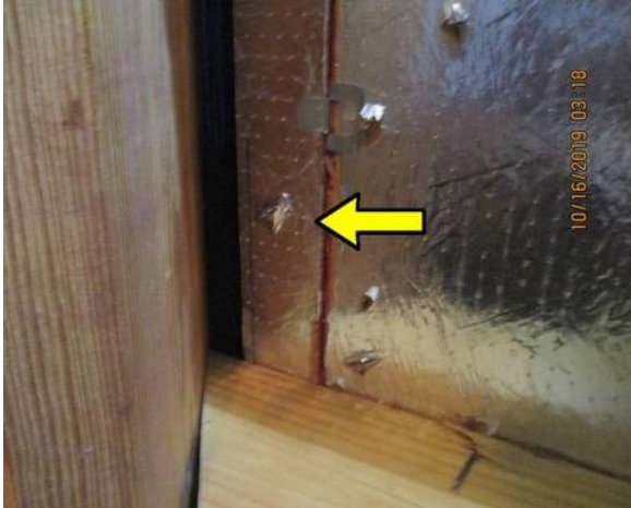
Deck board is too small at the ridge
