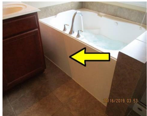
No access to the motor
