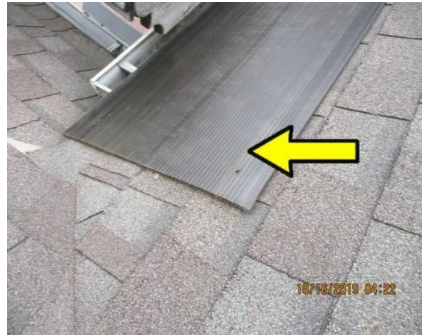
Improper flashing at back slope above patio cover
