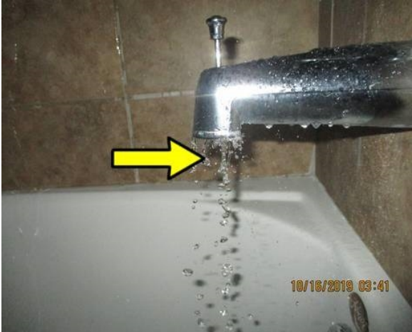
Diverter leaks at upstairs bath
