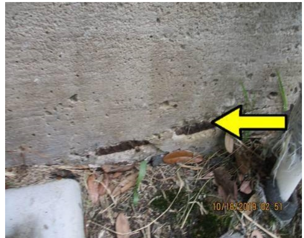
Exposed reinforcing at right side
