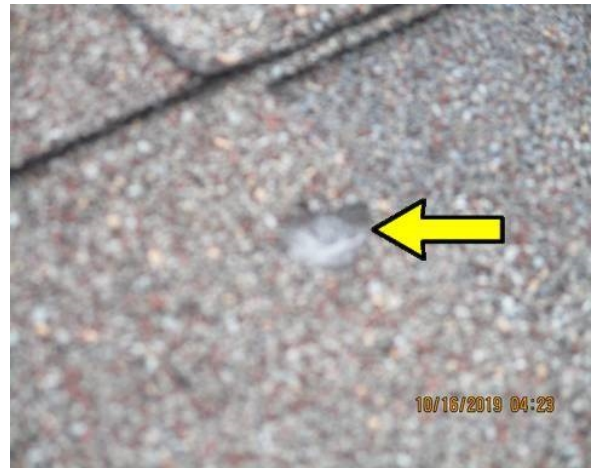
Possible hail damage in back
