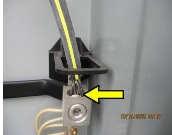
No antioxidant on service wires
