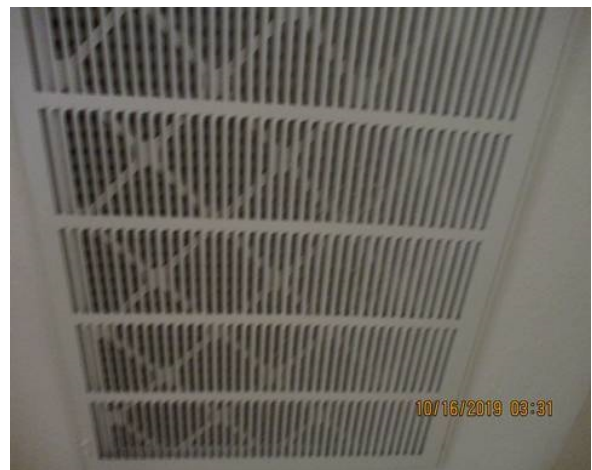
Remove filters out of return air grilles
