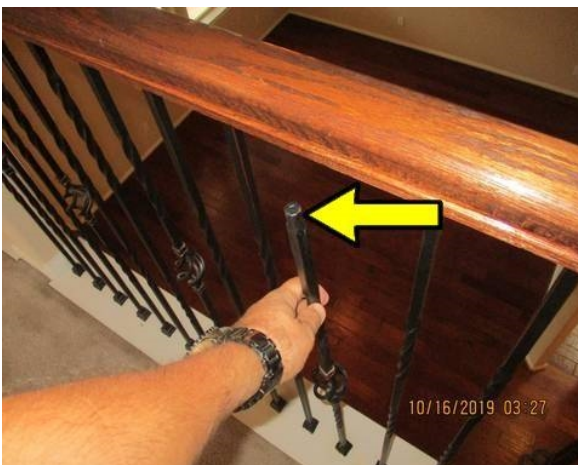
Baluster not attached
