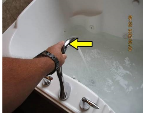
Faucet is loose at master tub
