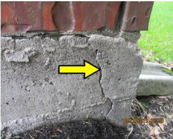
Spalled at back left
