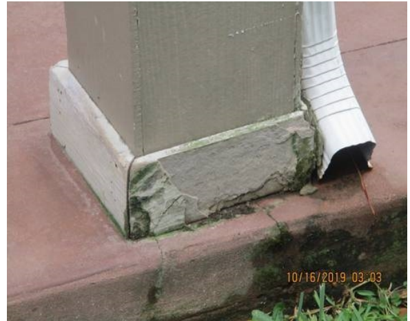
Deteriorated trim around back porch post
