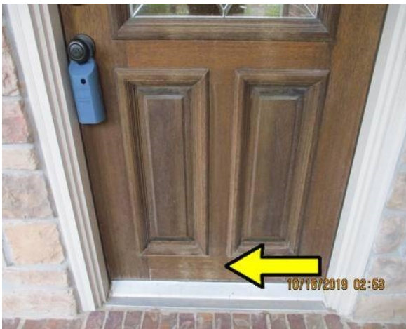
Finish on front door is deteriorating
