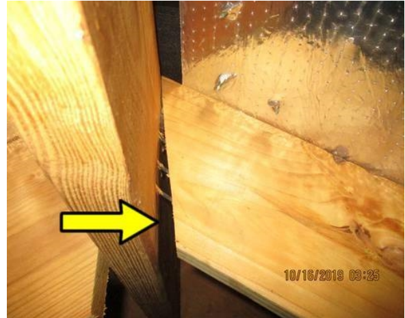
Rafter has pulled away from ridge board
