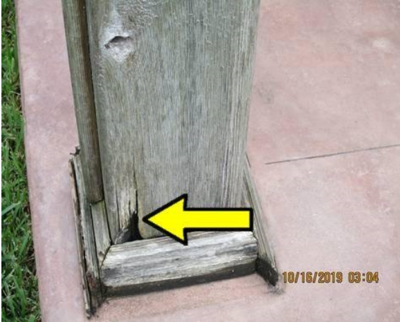
Deteriorated wood at back patio cover post
