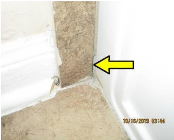
Seal grout around tub at upstairs bath
