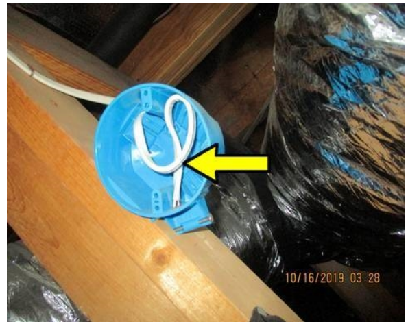
Add cover plate to junction box in attic access at top of stairs
