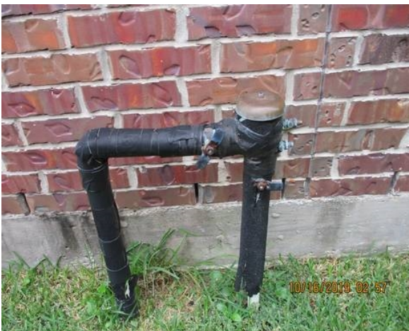
Backflow preventer installed
