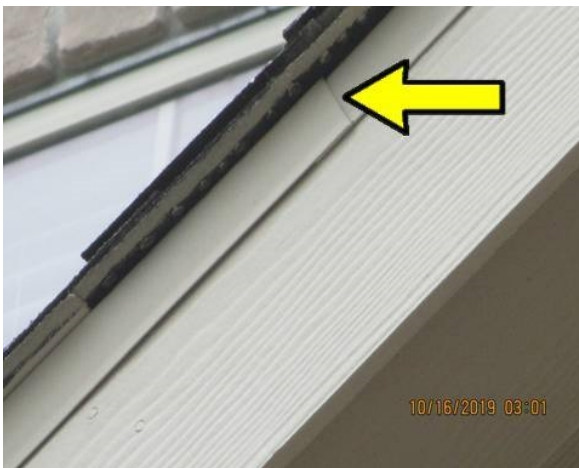
Drip edge is not properly installed
