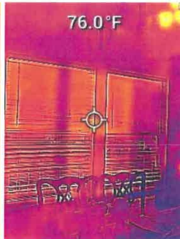
Some conditioned air loss from the windows
