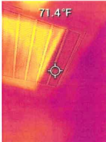
Temperature differential between registers and returns are within range
