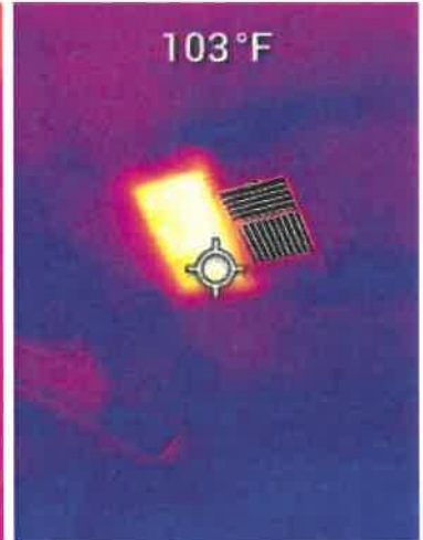
Temperature differential between registers and returns are within range
