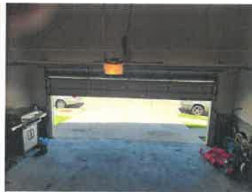
Garage door operating
