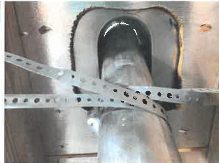
The water heater
