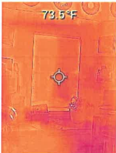
Some conditioned air loss from the windows
