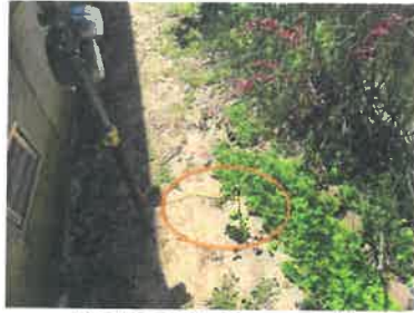
Bonding wire disconnected
