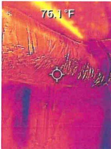
The ducting appears not to be leaking at the time of the inspection
