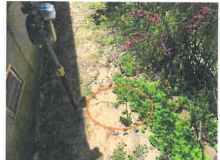
Bonding wire disconnected
