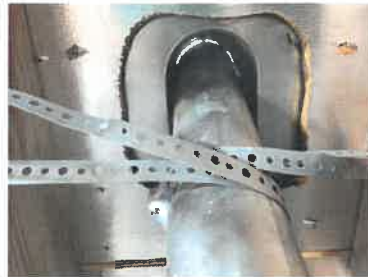
The water heater
