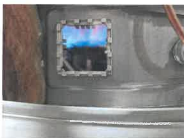
The blue flame of the burners indicates proper combustion.
