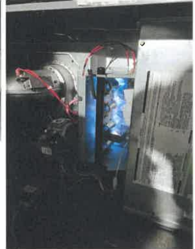
The blue flame of the burners indicates proper combustion.
