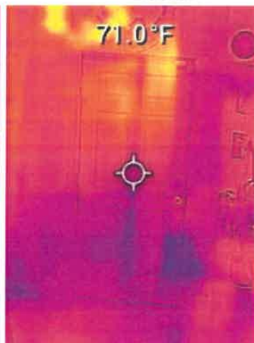
Some conditioned air loss from the front door
