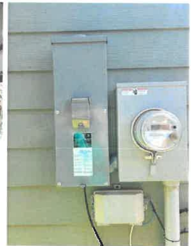
Main panel disconnect
