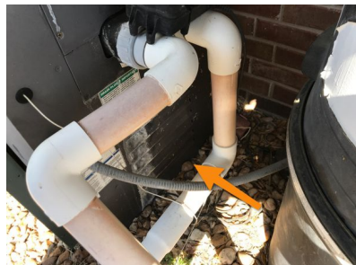
Heater is not connected to bonding
