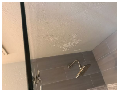
2nd Floor Bathroom Multiple Locations
