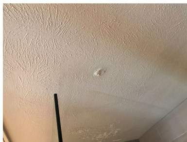
2nd Floor Bathroom Multiple Locations
