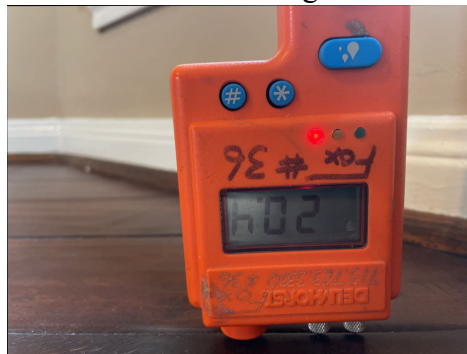
Wet floor in primary bedroom.
