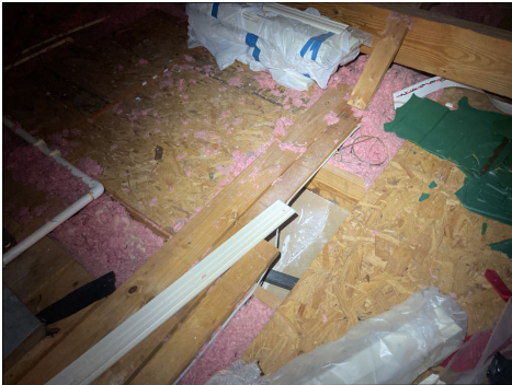
Decking incomplete/ missing insulation.
