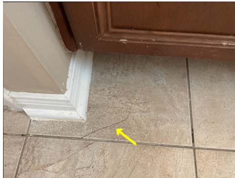
Cracked floor tile; Hall bath.
