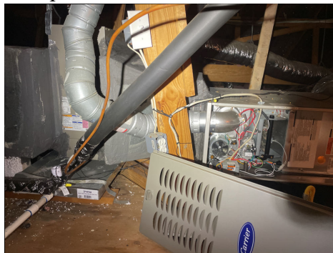
Improper slope of vent.
