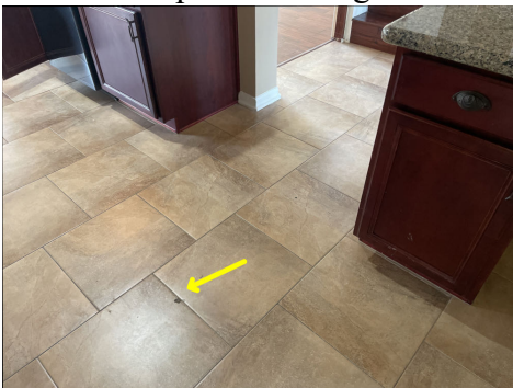
Damaged tile in Kitchen.
