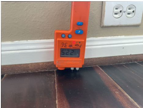
Wet floor in living room.
