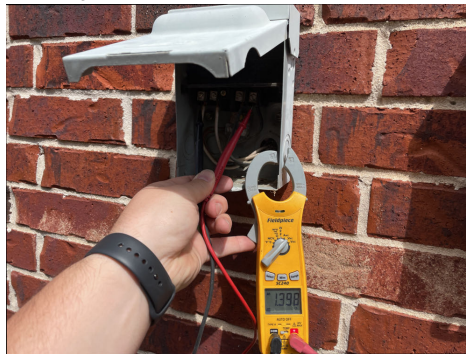
No power to disconnect, breaker tripped.
