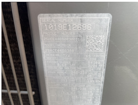
Upstairs Condenser. 2019 Carrier 4 Ton R410a.
