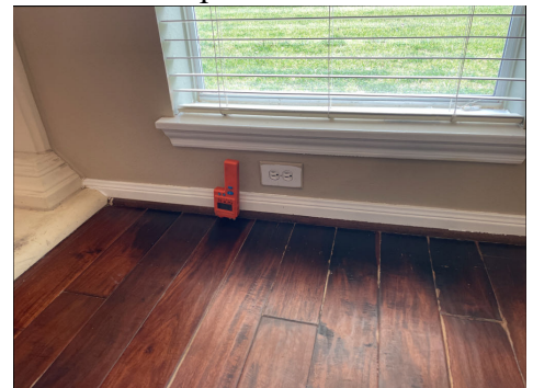
Wet floor in living room.
