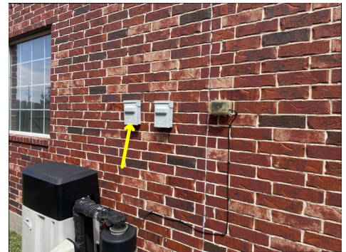
No power to disconnect, breaker tripped.
