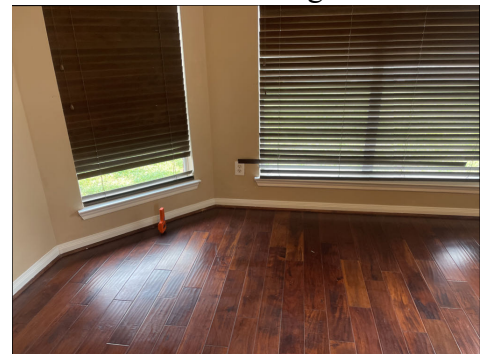
Wet floor in primary bedroom.
