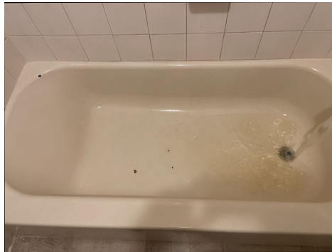
Porcelain damaged/chipped on steel tub; Jack and Jill.
