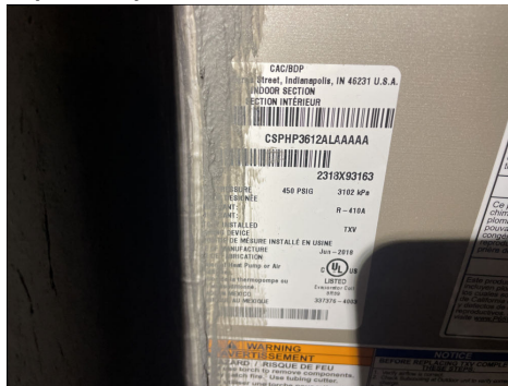
Downstairs Evaporator Coil. 2019 Carrier 3 Ton R410a.
