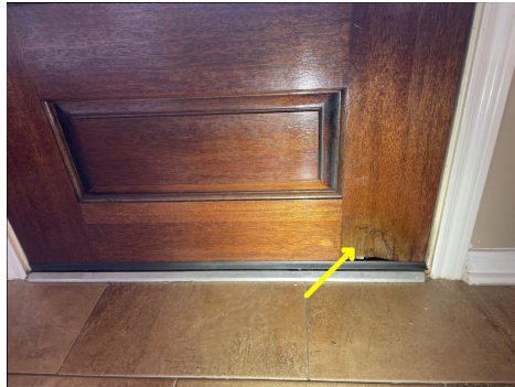
Front door is damaged.
