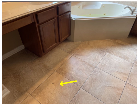
Damaged tile in Primary bath.
