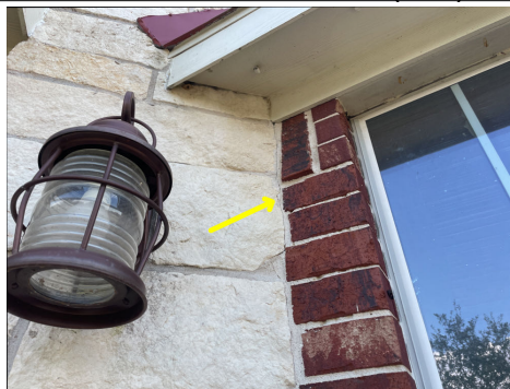
Crack in brick/stone joint.
