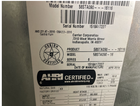
Upstairs Heater. 2019 Carrier.
