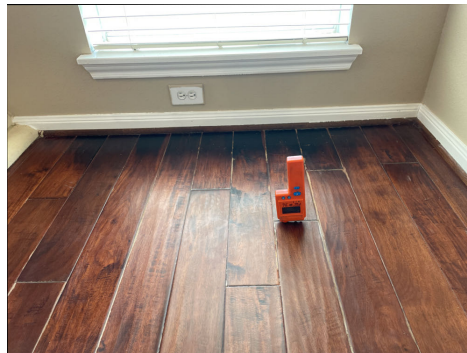
Wet floor in living room.
