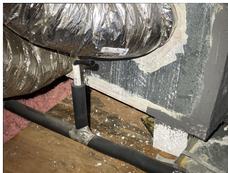
Downstairs Unit appears to have sweated at some point.
