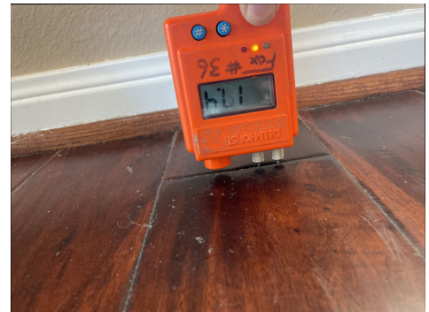
Wet floor in living room.
