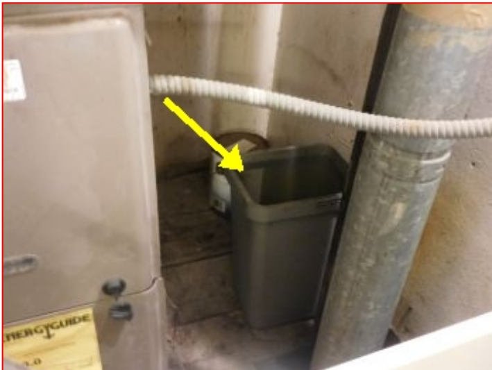
Trash can is full of dripping condensation from pipes above it?
