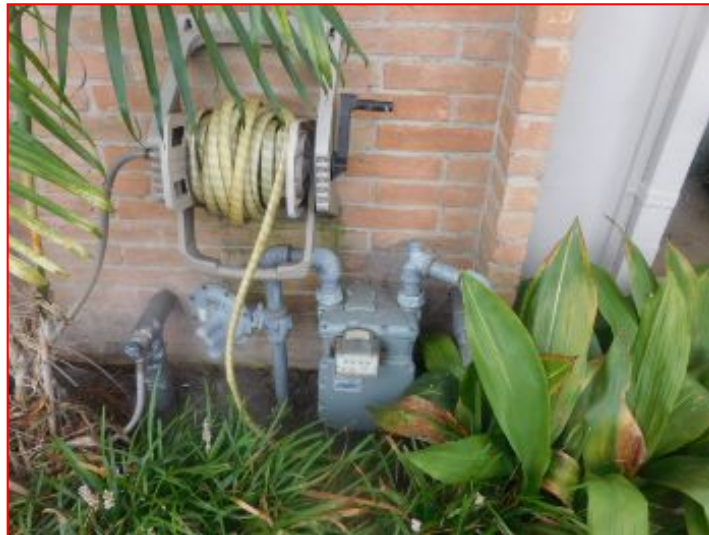
Gas meter in front.
