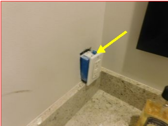
A plug is loose on the bathroom wall.
