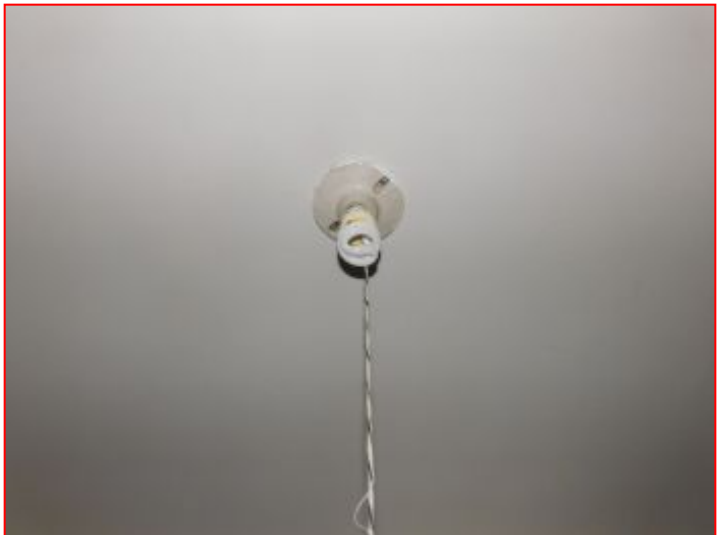
Open light bulbs in the closets are considered unsafe.
