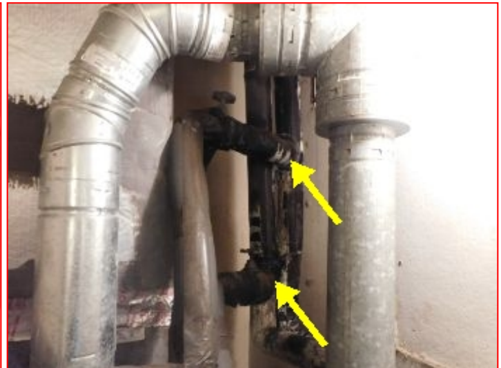
Dripping pipes above trash can
