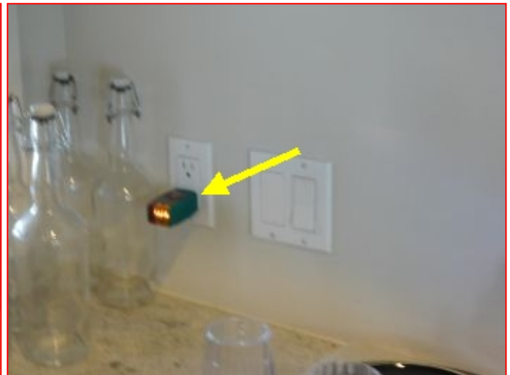
It is recommended that the left side kitchen sink plug be equipped with ground fault circuit interrupter (GFCI).
