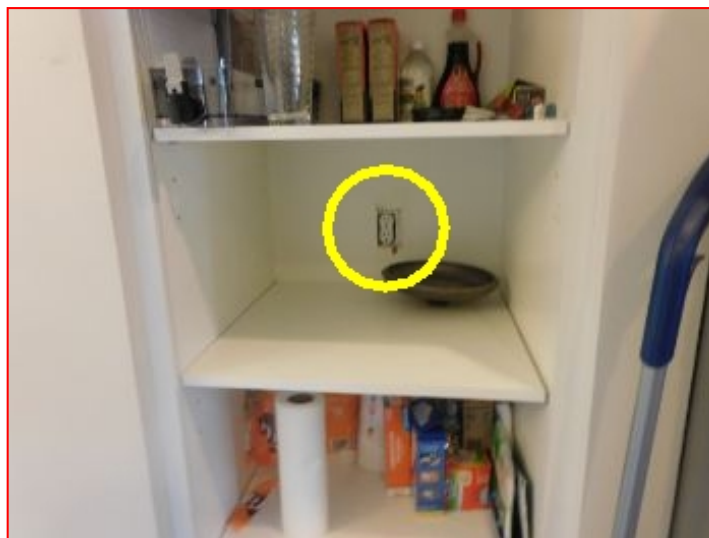
Missing cover plate
