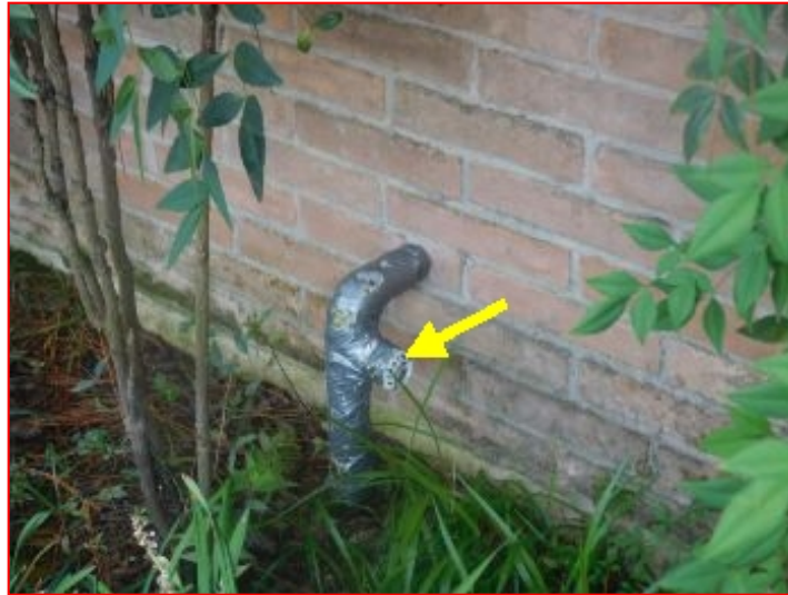
Main water shut off valve
