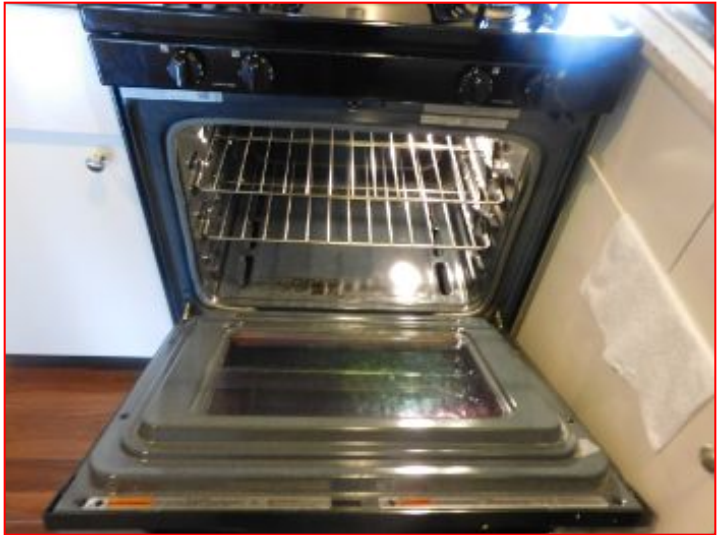
Temperature was 450. Oven requires calibration.
