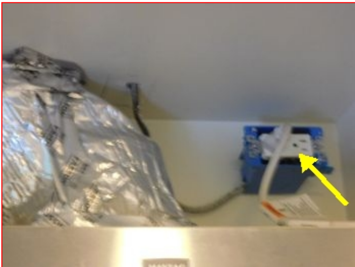
Missing cover plate above microwave
