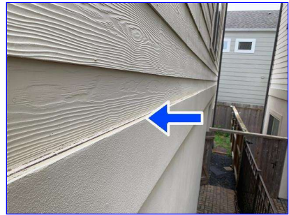
E. Missing Flashing
