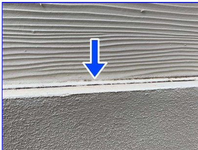
E. Missing Flashing
