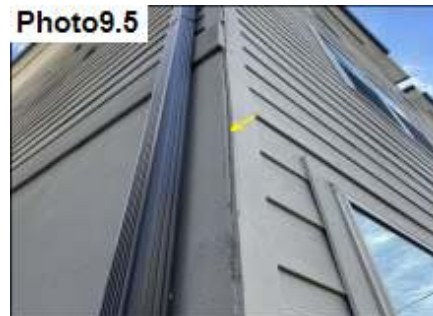
Sealant separation noted at siding transitions.
