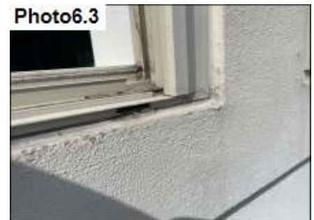
Sealant separation noted around window frames.
