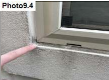
Sealant separation noted around window frames.
