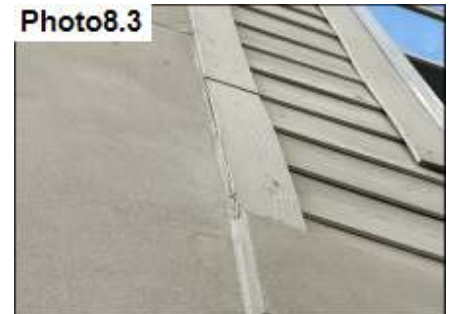
Sealant separation noted at siding transitions.
