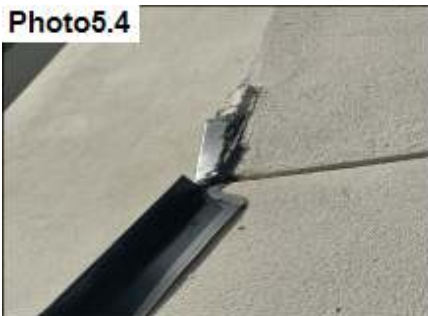
It is suggested to reseal metal cap terminations.
