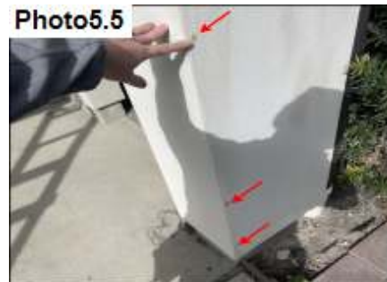
Glue / adhesive noted in stucco.
