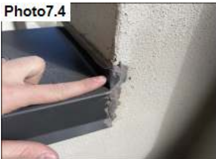
Photo7.4 It is suggested to reseal all metal cap terminations.
