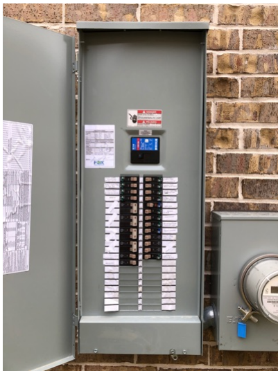
150 Amp Square D service panel
