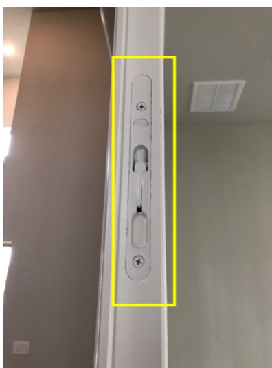
Door latch not functional
