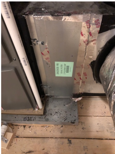
Media filter located at base of furnace
