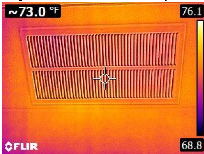
Thermal image of return air grille
