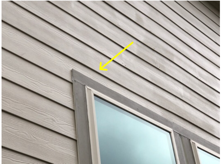
No flashing installed above windows
