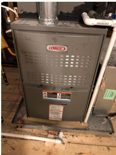
Lennox gas furnace
