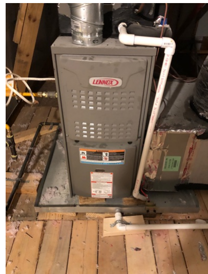
Lennox gas furnace
