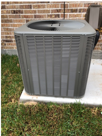
Unit # 1: Downstairs 2019 model Lennox 4 ton condenser
