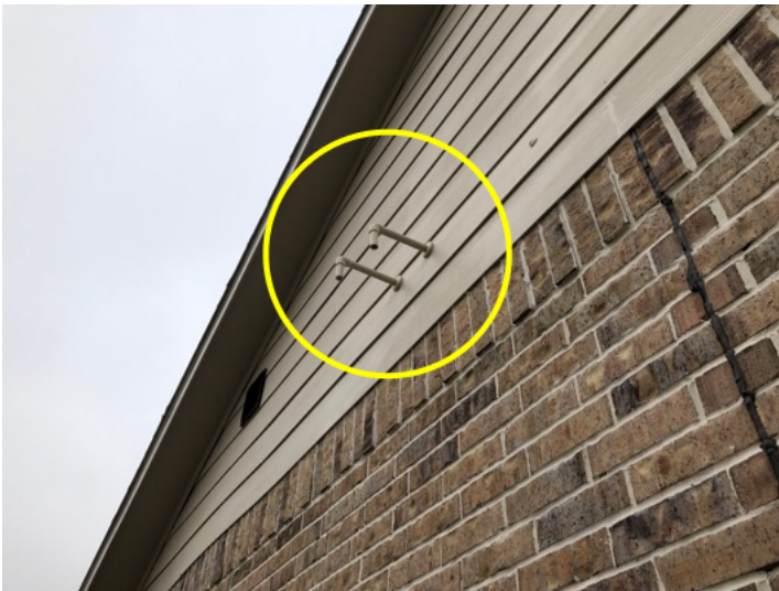
Secondary drain lines
