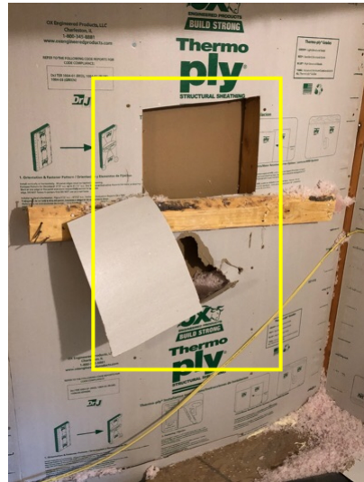
Sheathing damaged / removed
