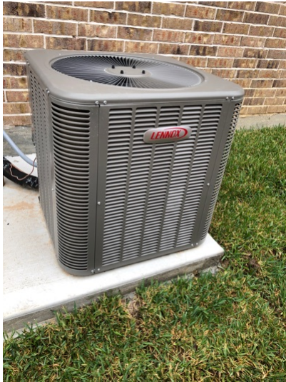
Unit # 2: Upstairs 2019 model Lennox 2 ton condenser
