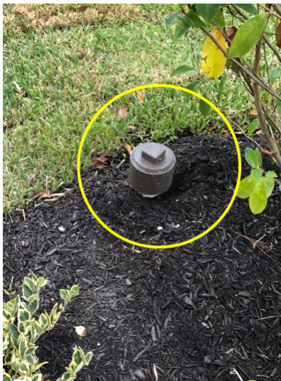
Waste plumbing cleanout located in front flowerbed
