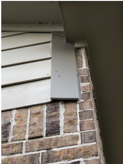
Trim at right rear corner not flush with wall and not properly caulked.
