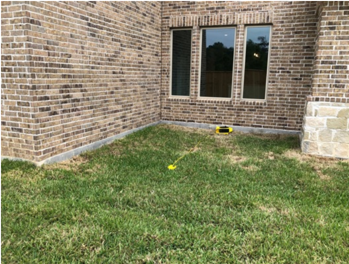
Insufficient grading at back yard
