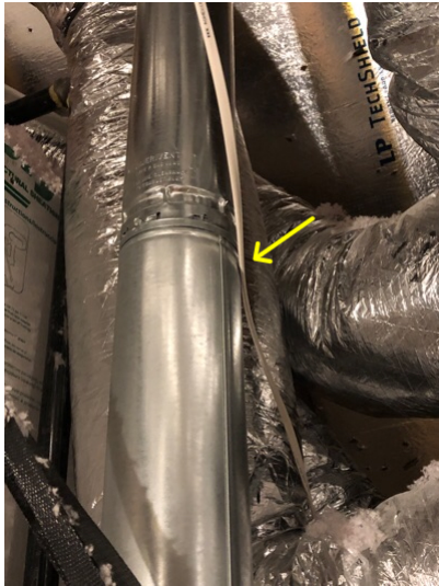
Circuit in contact with flue pipe
