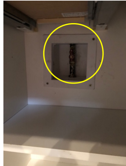
Gas shut off valve for cooktop
