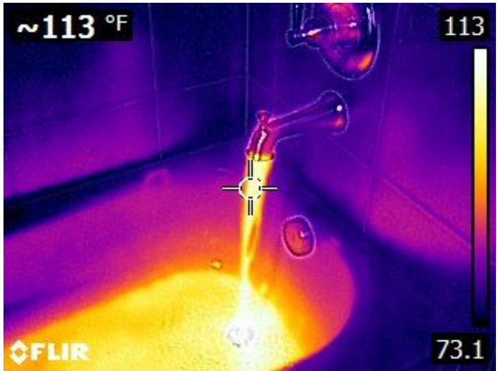
Hot water was verified at all interior fixtures and showers. Hot water temperature measured: 113F
