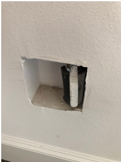
Main water supply valve
