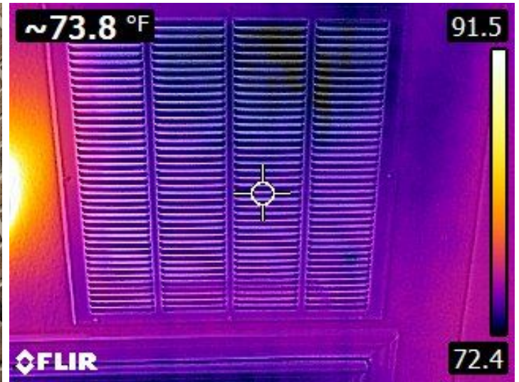
Thermal image of return air grille
