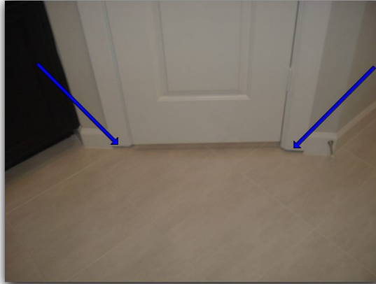
The pantry door trim was short cut.
