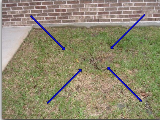
Erosion was observed at the rear yard area of the house.
