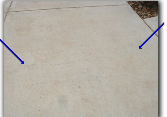
The driveway has visible cracks.
