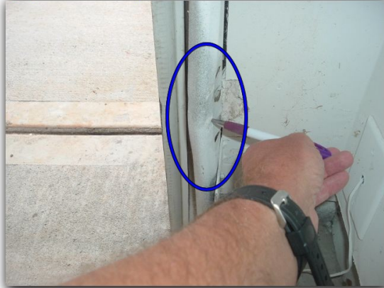
The garage door track has damage.
