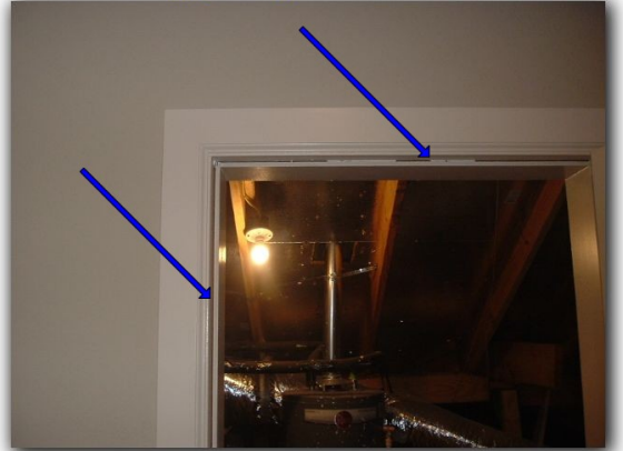
The attic door weather stripping is missing.
