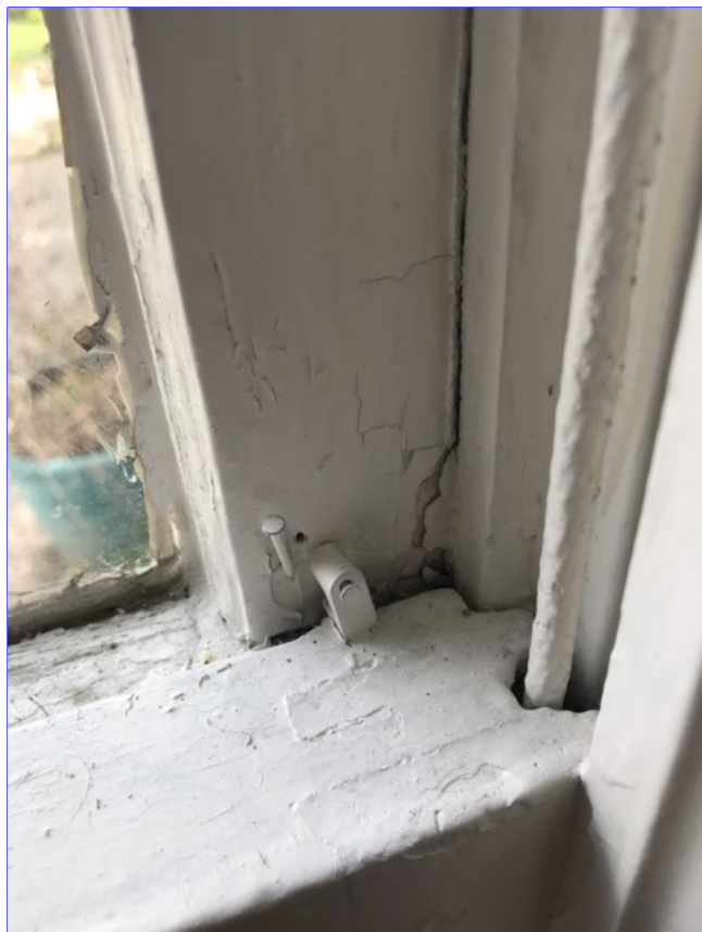
(7) Living room windows are painted shut.
