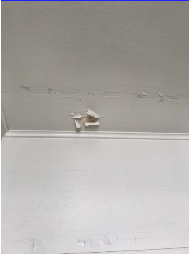
(4) Evidence of water intrusion in the second floor rear hallway.
