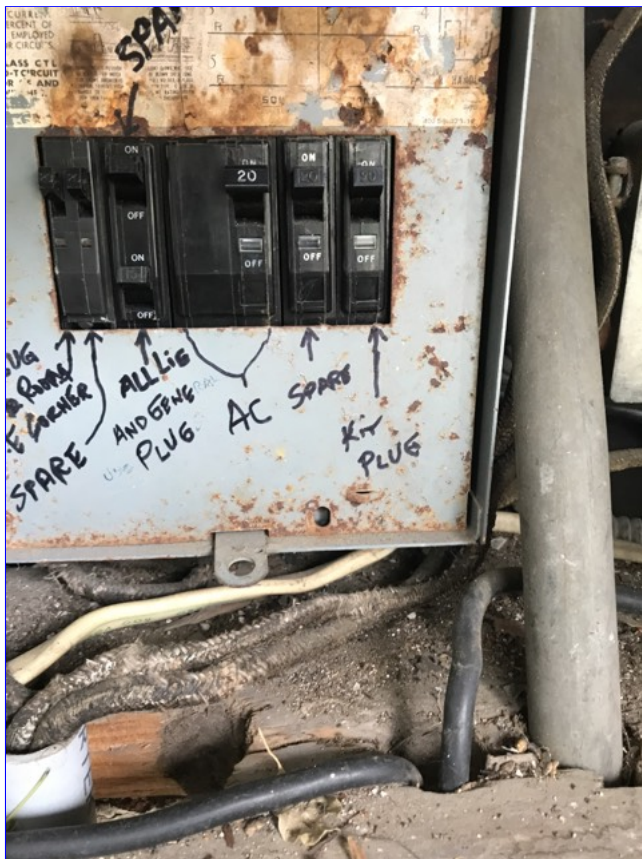
(3) Electrical distribution panel is severely corroded.
