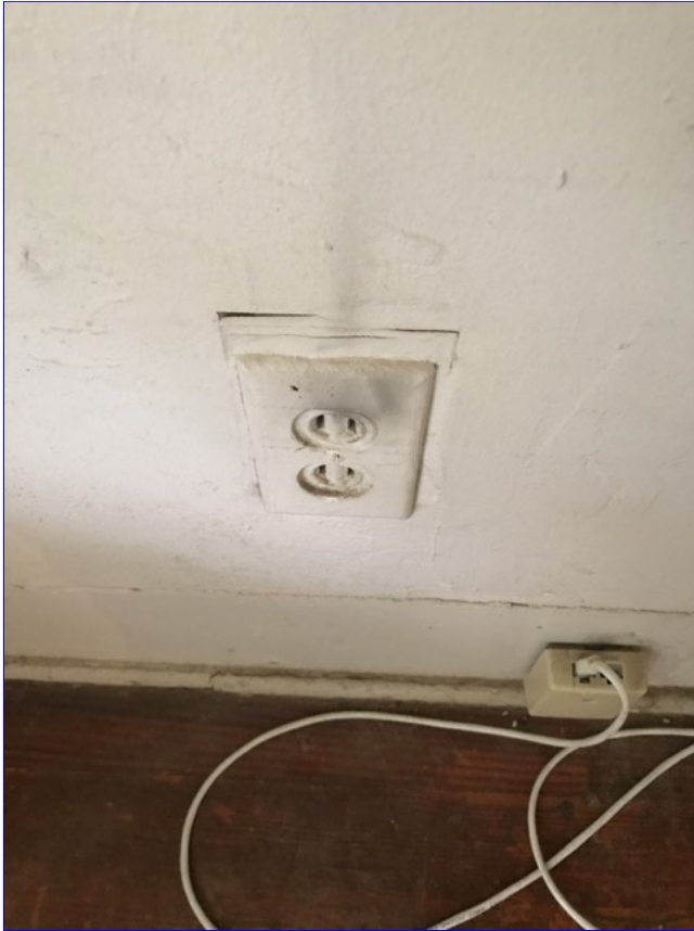
(18) Second floor rear hallway lights do not function.
