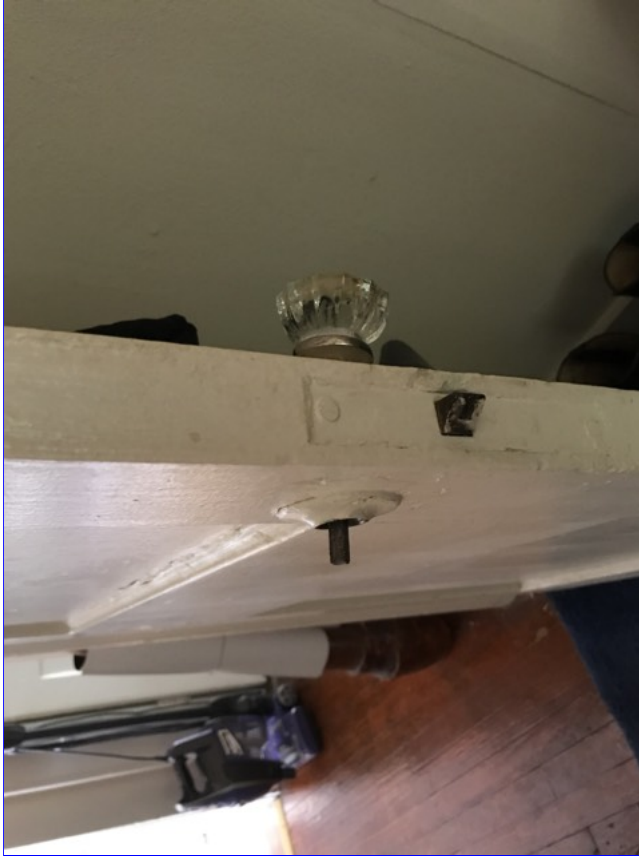
(2) Rear entry door has loose hardware.
