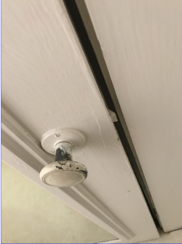
(7) Bathroom door hardware is loose and damaged.
