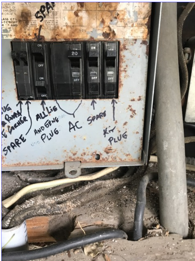
(3) Electrical distribution panel is severely corroded.
