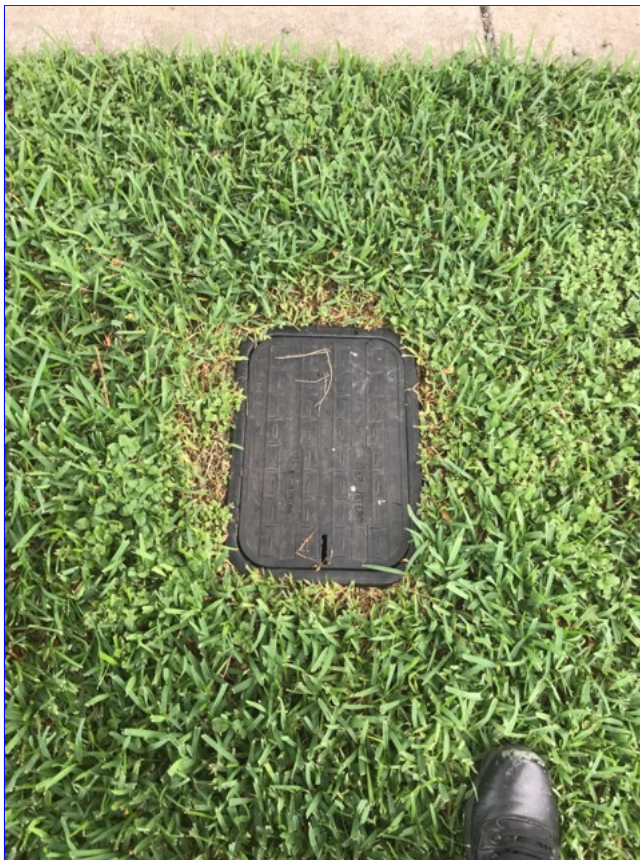
(4) Hot water bath tub supply valve leaks at the stand.
