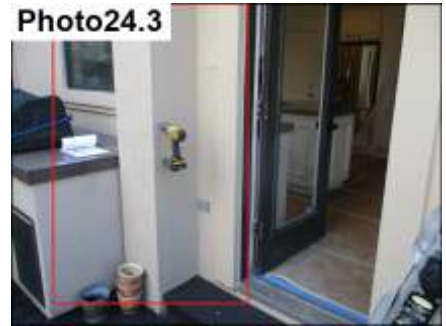
Substrate Damage / Repair
