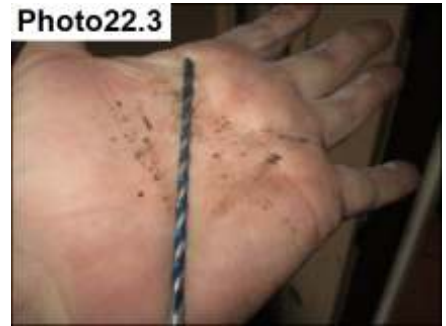
Substrate Damage / Repair
