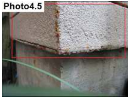
Rusted Casing Bead/ Repair As
