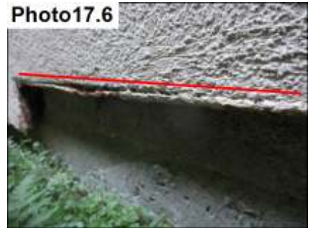
Rusted Pilaster Stop / Repair As Needed
