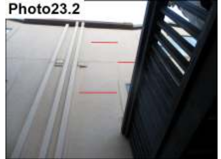
Cracks / Assess & Seal As Needed
