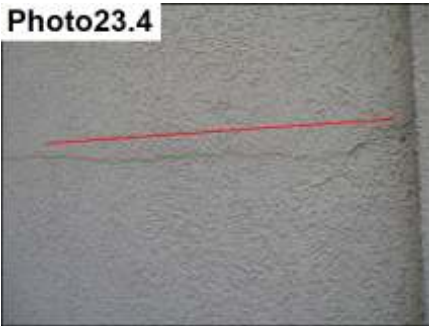
Cracks / Assess & Seal As Needed
