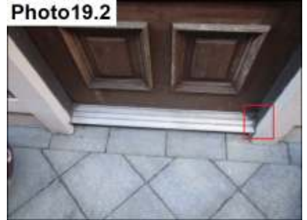
Wood Rot / Repair
