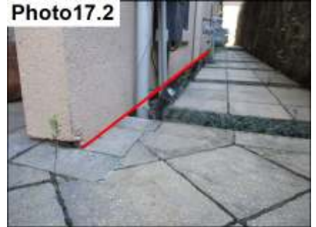
Rusted Pilaster Stop / Repair As Needed
