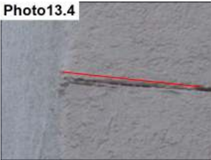
Crack Noted / Seal Or Repair As Needed
