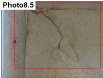
Cracks /Further Assess And Repair As Needed
