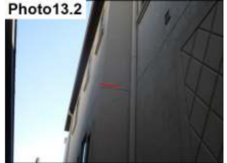
Crack Noted / Seal Or Repair As Needed
