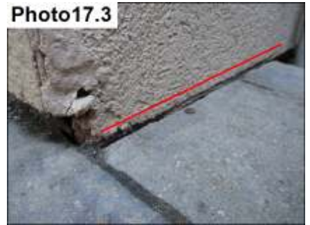
Rusted Pilaster Stop / Repair As Needed
