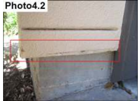
Rusted Casing Bead/ Repair As
