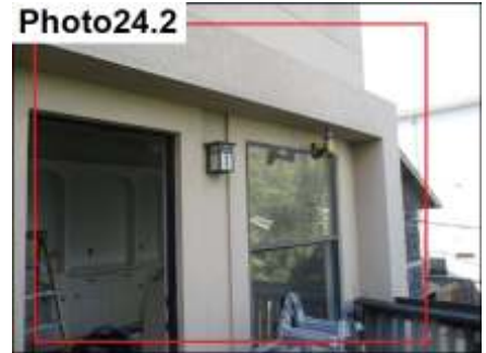
Substrate Damage / Repair
