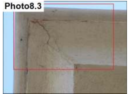
Cracks /Further Assess And Repair As Needed
