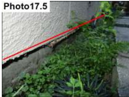
Rusted Pilaster Stop / Repair As Needed
