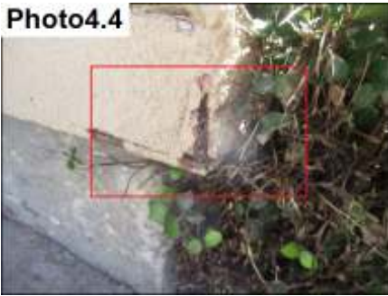
Rusted Casing Bead/ Repair As
