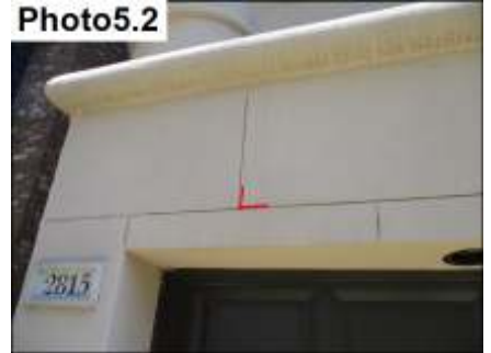
Minor Cracks / Seal
