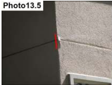
Crack Noted / Seal Or Repair As Needed
