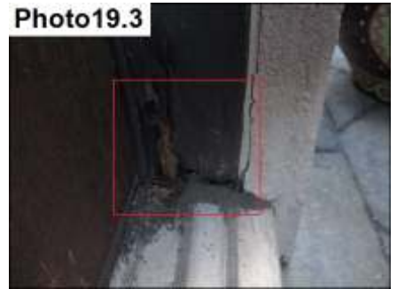
Wood Rot / Repair
