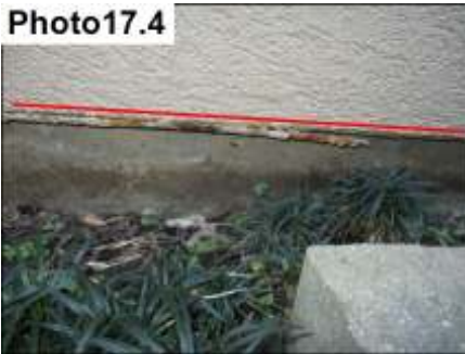
Rusted Pilaster Stop / Repair As Needed
