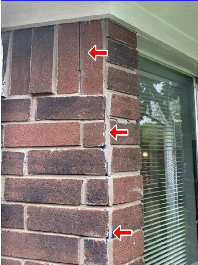
E. Item 7(Picture) Brick veneer mortar cracks were observed.
