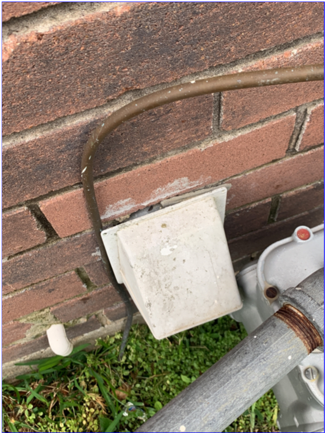
H. Item 1(Picture) The dryer exhaust vent should be caulked to the wall.
