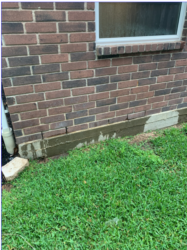
B. Item 1(Picture) Moisture was observed coming from the outside wall at the master bath.
