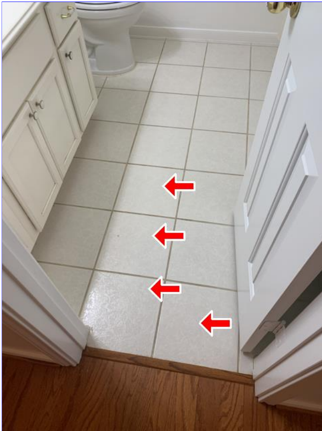
F. Item 3(Picture) Some floor tiles are not fully set to slab.
