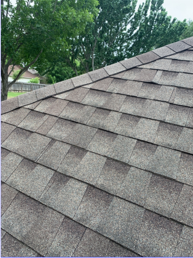
C. Item 3(Picture) The roof covering, is not new and shows signs of wear consistent with its age.
