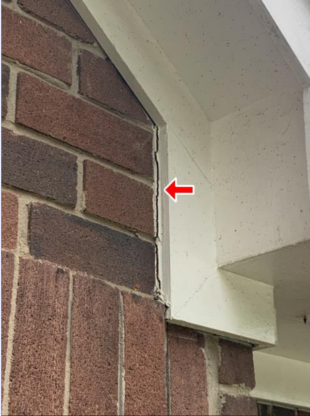
E. Item 2(Picture) Areas around the home where are the brick, trim, and siding meet, need to be caulked and sealed.
