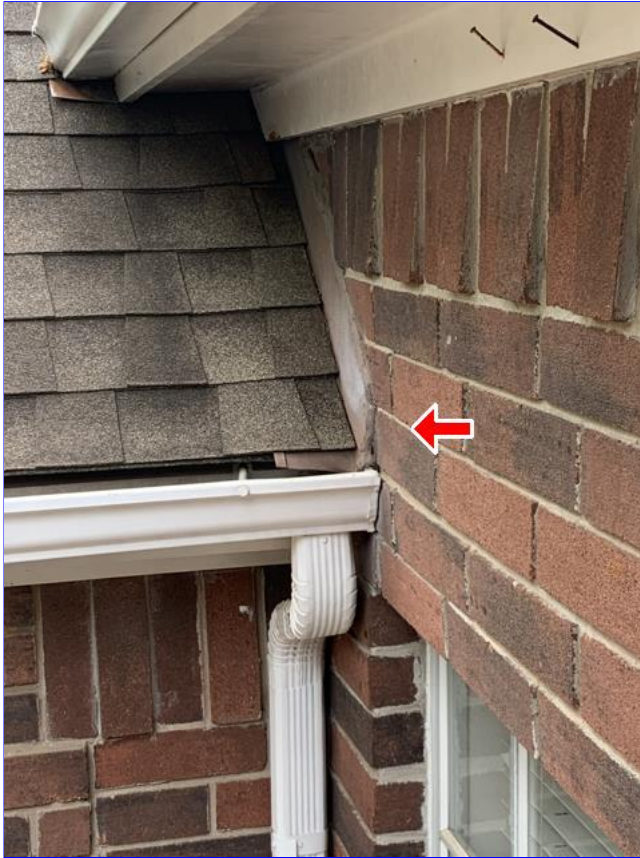
B. Item 5(Picture) No kick out flashings are observed at gutters where roof line and vertical wall flashings meet gutters.
