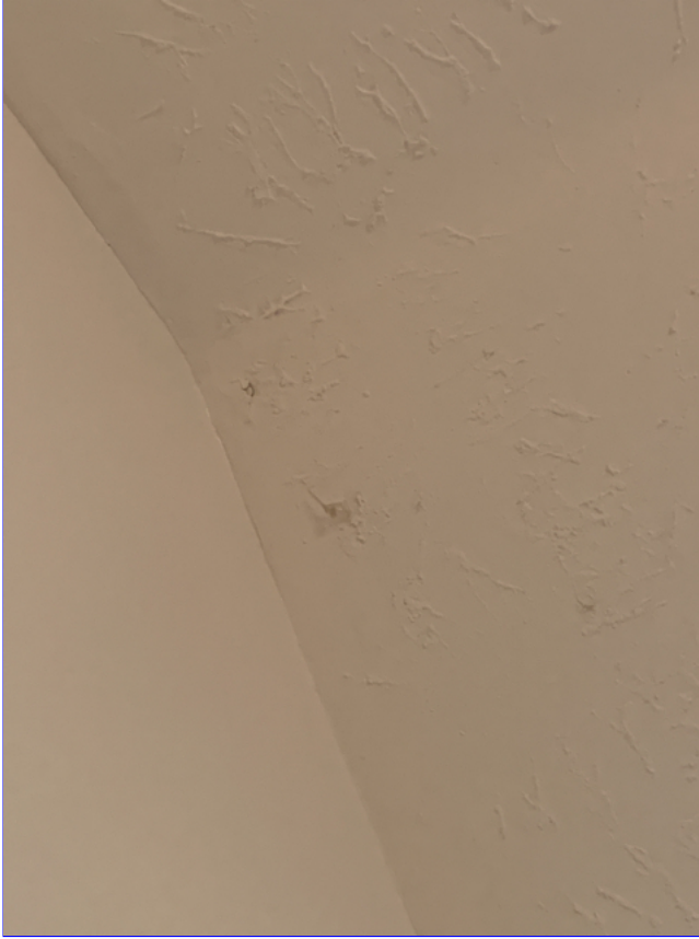
F. Item 1(Picture) Drywall tape joint cracks and/or nail pops were observed around the home.
