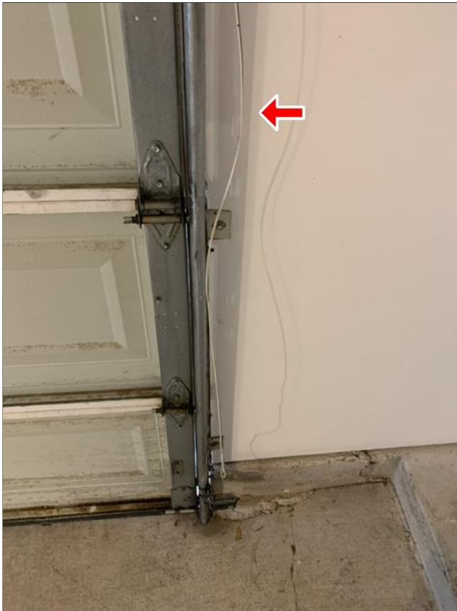
G. Item 2(Picture) The wires for the garage door sensors or not secure.
