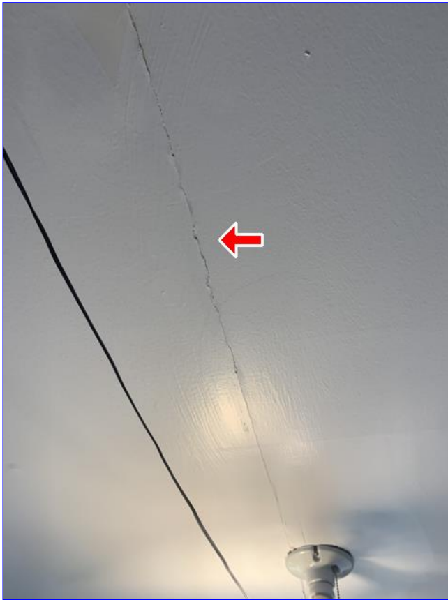
F. Item 4(Picture) Drywall tape joint crack observed in the garage.
