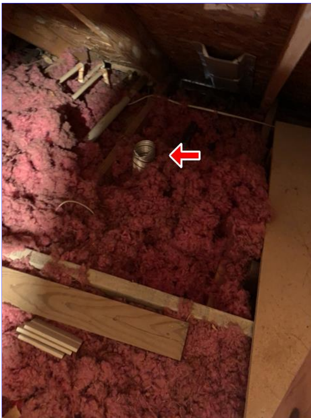
F. Item 1(Picture) Exhaust fans terminating into attic space.
