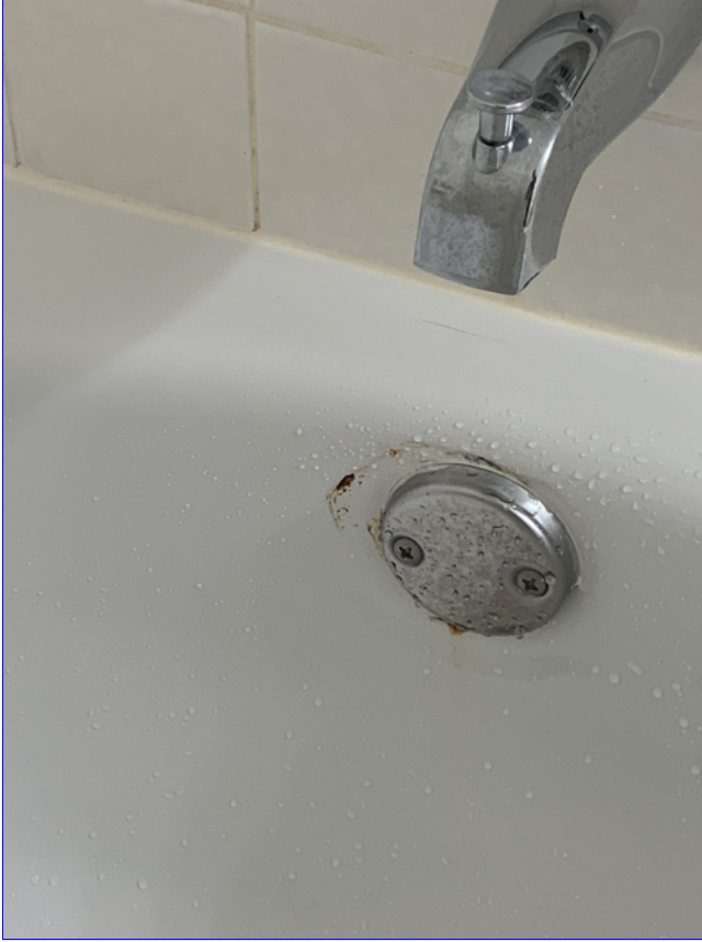
A. Item 1(Picture) Rust and chipped areas were observed on the tub in the guest bathroom.
