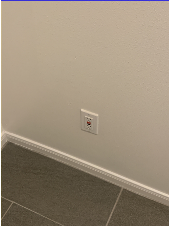
B. Item 1(Picture) GFCI outlet in bathroom closet does not reset.
