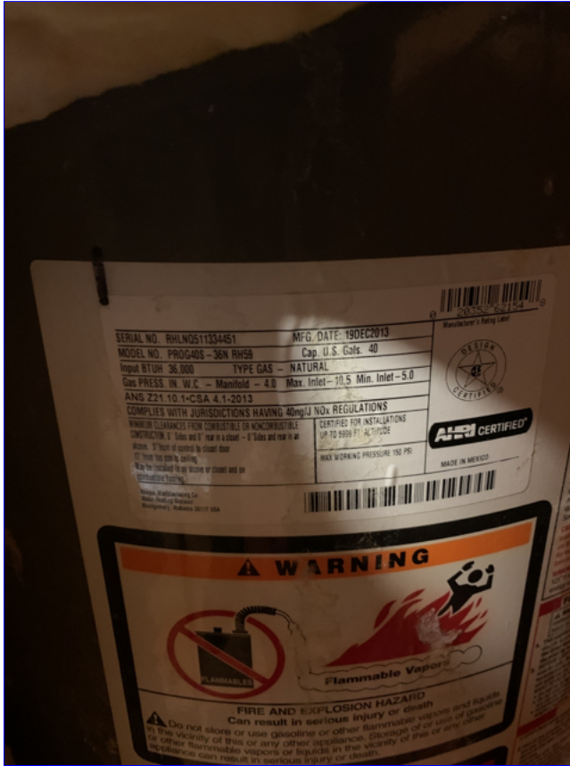
C. Item 1(Picture) Water heater service tag. Manufacture date 2013.
