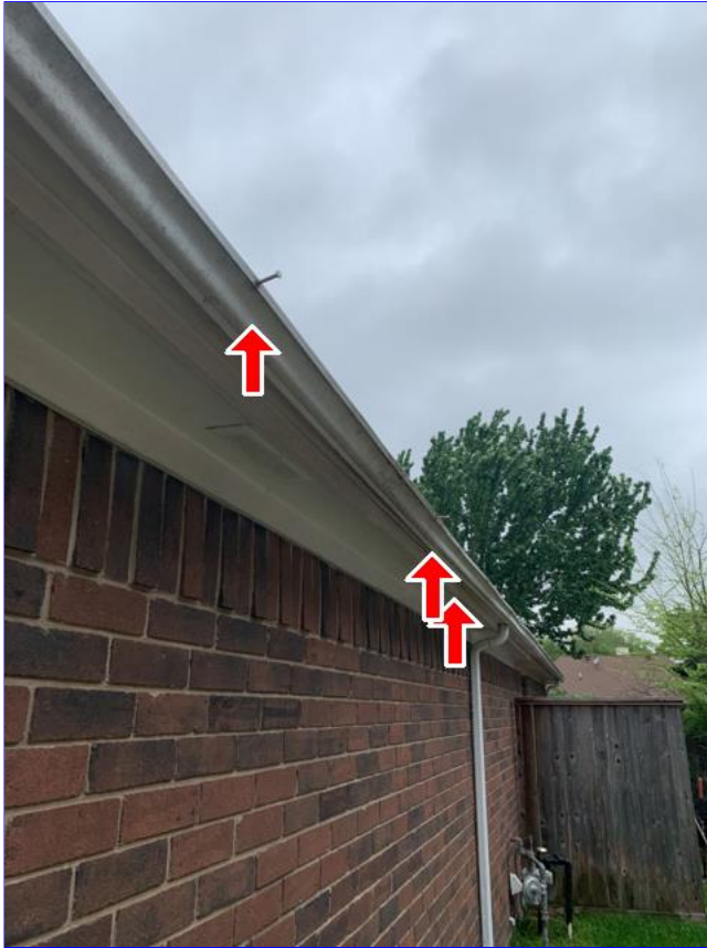
B. Item 2(Picture) The gutters hold water, sag, leak and are in a general state of disrepair. Recommend remove or replace as needed.
