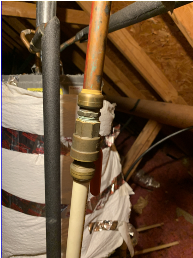
A. Item 4(Picture) Shark bite plumbing fittings where observed.
