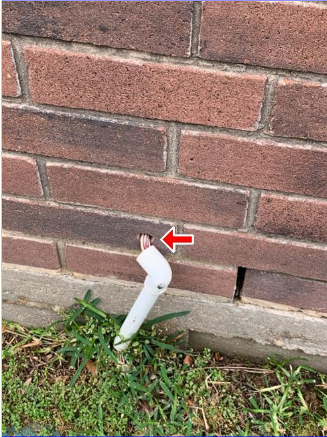
E. Item 8(Picture) Penetrations for sprinkler wiring into the wall should be sealed.
