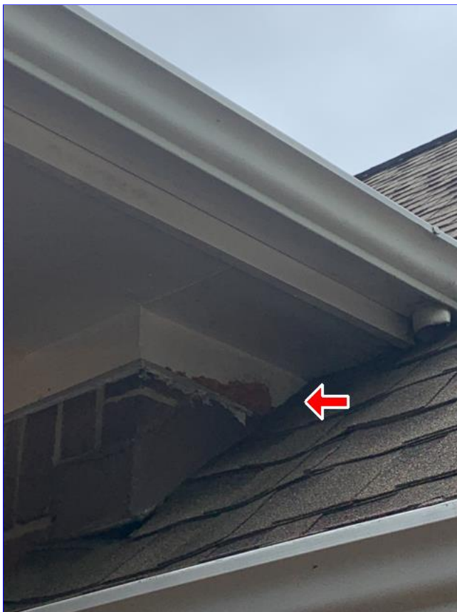
C. Item 1(Picture) Pest chewing on wood exterior of home observed.
