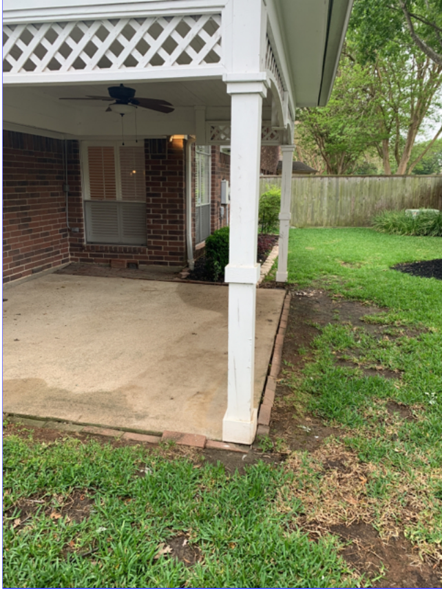
K. Item 1(Picture) Impossible to know whether the proper footers were used under the post or if the patio cover was attached to the home properly.
