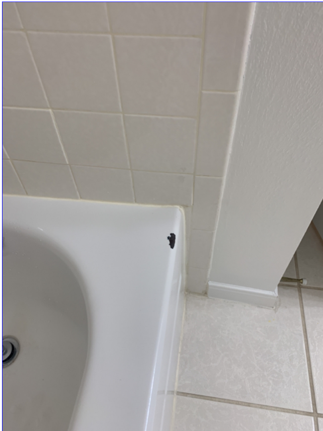
A. Item 2(Picture) Rust and chipped areas were observed on the tub in the guest bathroom.
