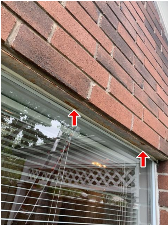
E. Item 10(Picture) Steel lintils above windows have rust and need to be painted.
