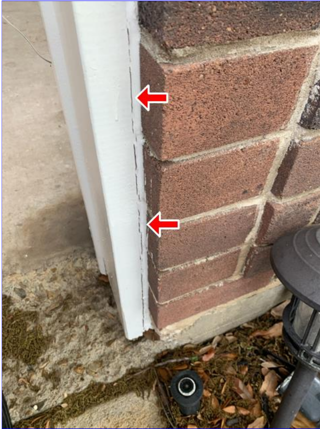
E. Item 1(Picture) Areas around the home where are the brick, trim, and siding meet, need to be caulked and sealed.
