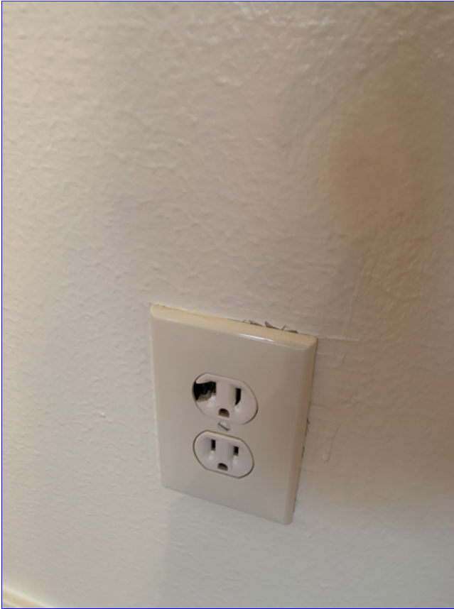
B. Item 3(Picture) Outlet is damaged in the master bedroom. Recommend replacement.
