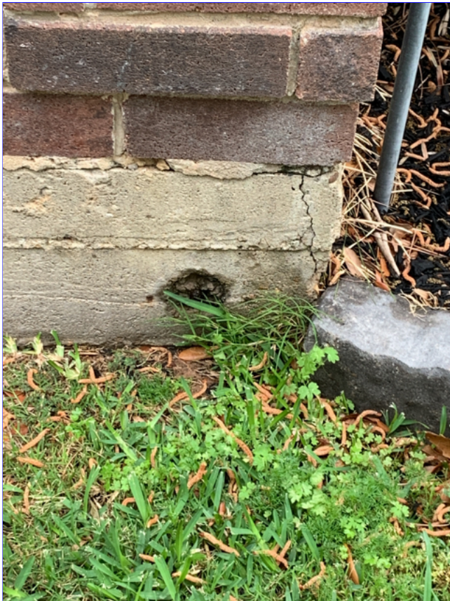
A. Item 4(Picture) Exposed post tension cable ends were observed.
