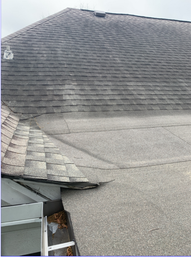
C. Item 4(Picture) The roof covering, is not new and shows signs of wear consistent with its age.
