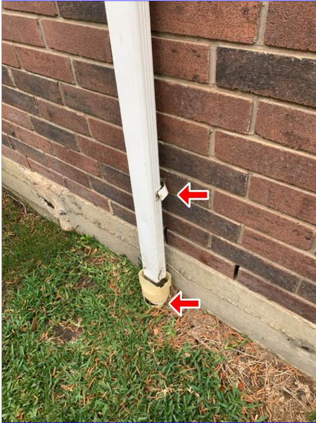
B. Item 3(Picture) The gutters hold water, sag, leak and are in a general state of disrepair. Recommend remove or replace as needed.
