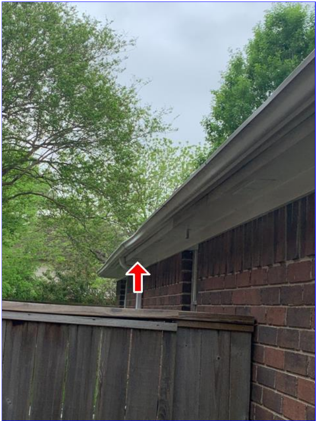
B. Item 4(Picture) The gutters hold water, sag, leak and are in a general state of disrepair. Recommend remove or replace as needed.
