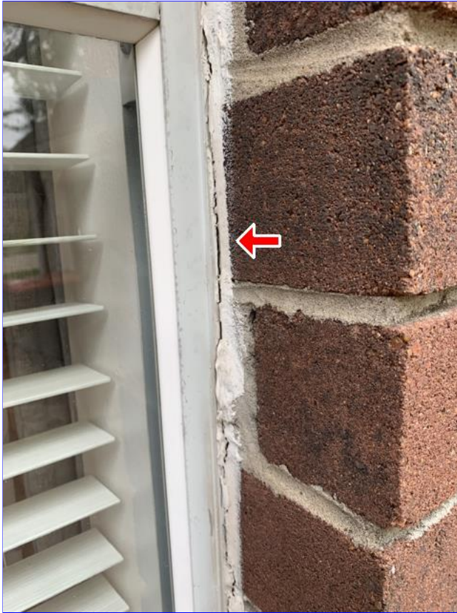
H. Item 1(Picture) The perimeter sealant, has failed on some windows.
