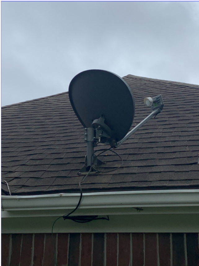
C. Item 7(Picture) The satellite dish was observed mounted on the roof covering.
