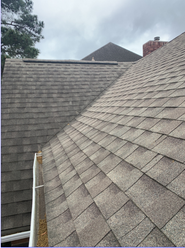
C. Item 2(Picture) The roof covering, is not new and shows signs of wear consistent with its age.
