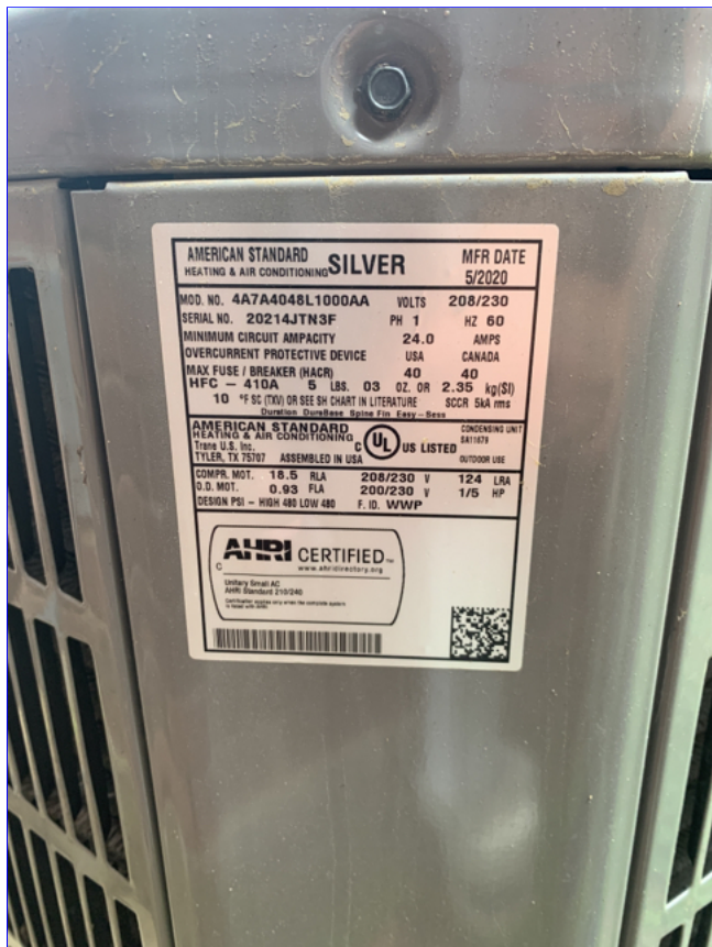
B. Item 1(Picture) AC service tag
