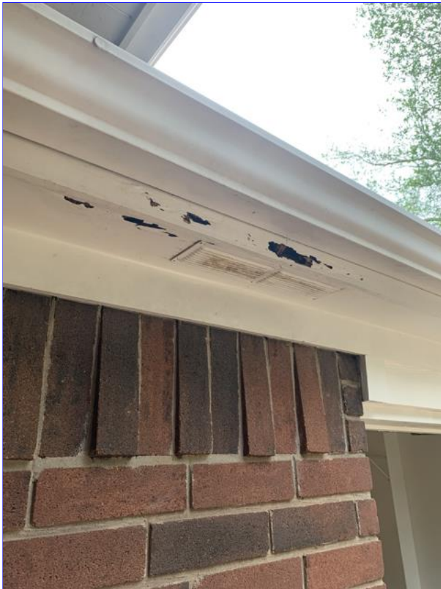
D. Item 1(Picture) Wood rot was observed on the soffit and fascia by the front door.
