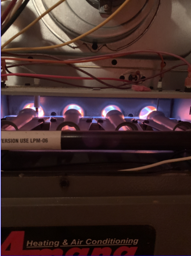
A. Item 1(Picture) Furnace burners
