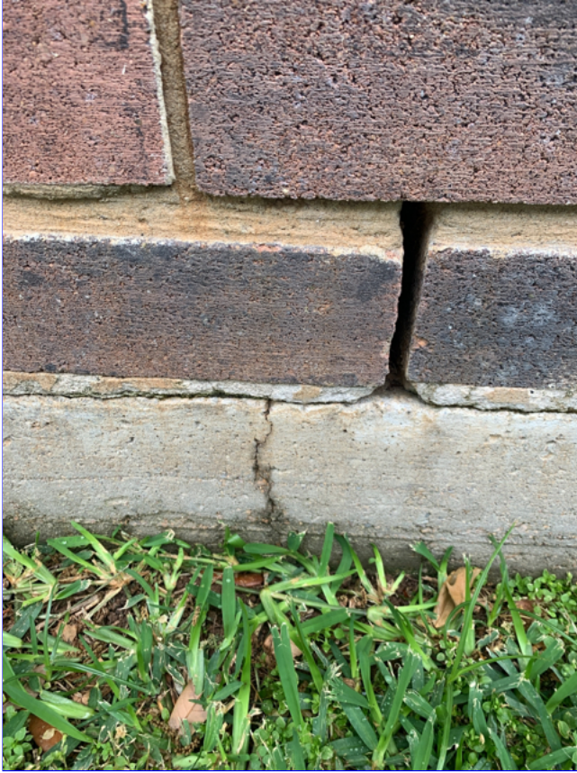
A. Item 2(Picture) There is some slab edge cracking.
