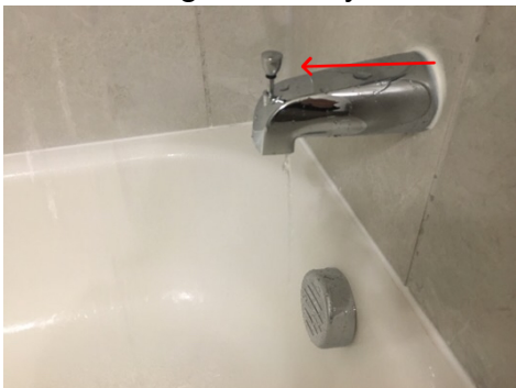
Bathroom 1: diverter not ok
