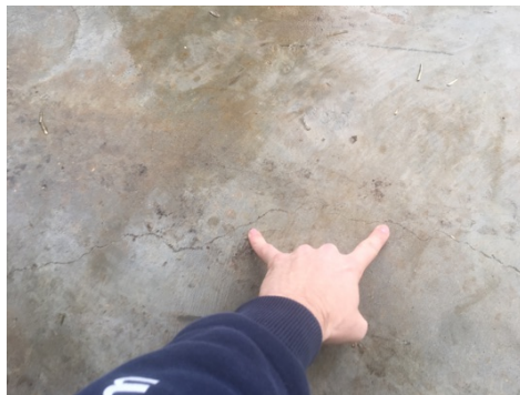
Back porch: hairline crack
