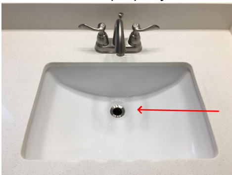
Bathroom 2: missing stopper at right lavatory
