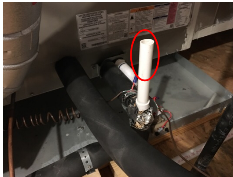
Cap missing on primary condensate drain line cleanout
