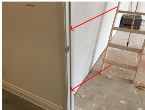
Garage man door: missing weatherstripping
