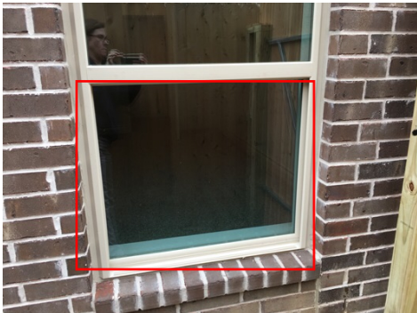
Around the house: missing screens
