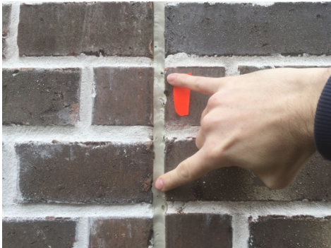
Left: incomplete caulk at expansion joint
