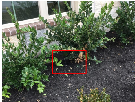
FYI: Main Cleanout located on the front
