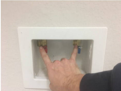
Laundry room: washing machine connections improperly oriented
