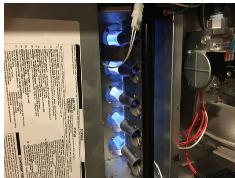
Furnace fired up
