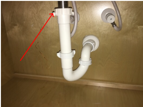
Bathroom 3: leak at drain connection
