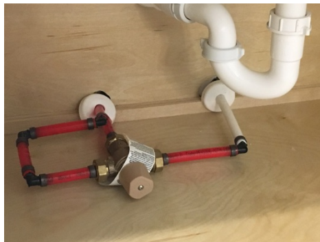
Bathroom 2: loose supply line
