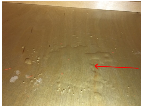
Bathroom 3: water on cabinet floor from leak at drain
