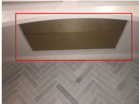
Range hood not installed
