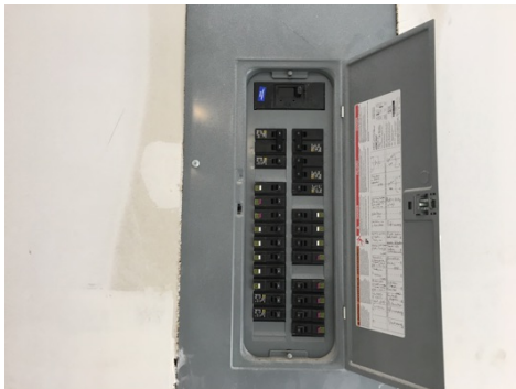
Garage: service panel
