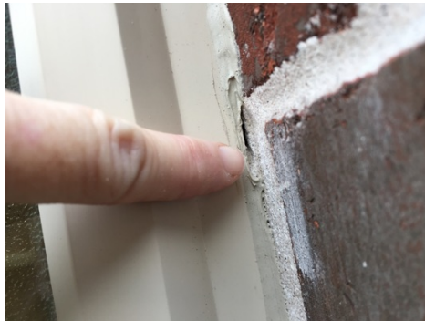
Around the house: additional caulk needed
