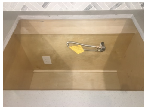
Cooktop not installed
