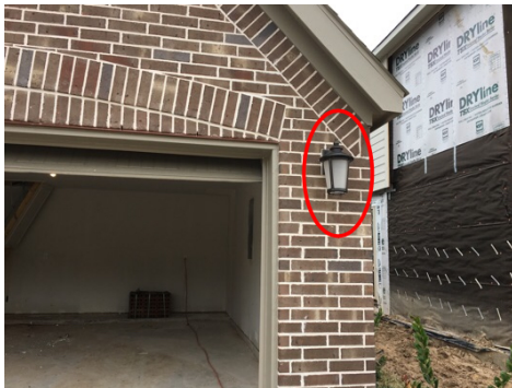
Front right: inoperative fixture
