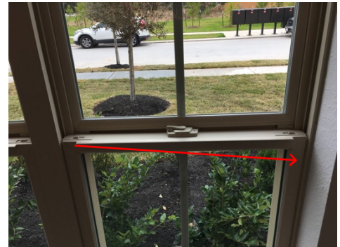
Office 1: window out of square
