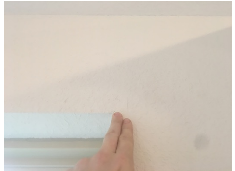
Breakfast nook: hairline crack
