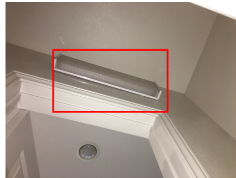
Pantry: inoperative fixture
