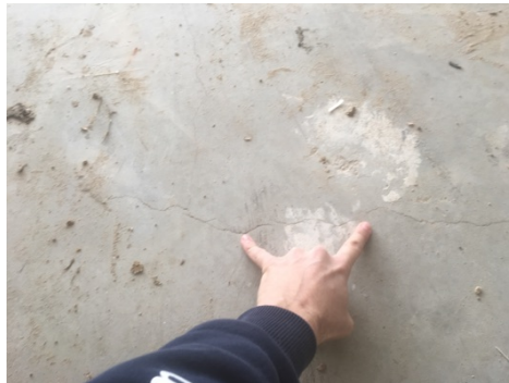
Garage: RTS hairline crack
