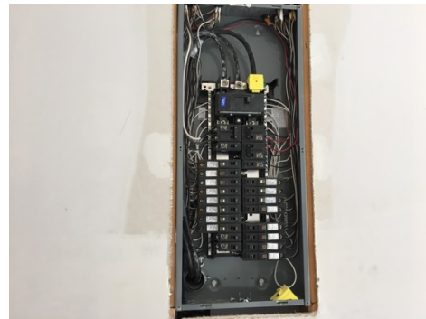
Service panel with deadfront removed
