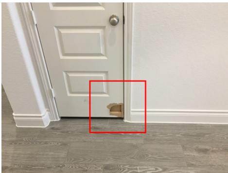
Foyer/hallway: damaged door
