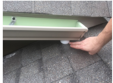
Downspout extension missing, discharge on roof
