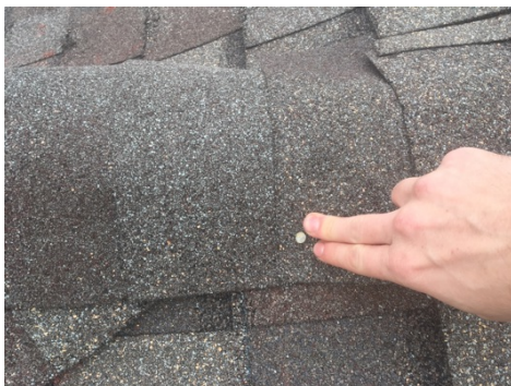
Exposed nail heads
