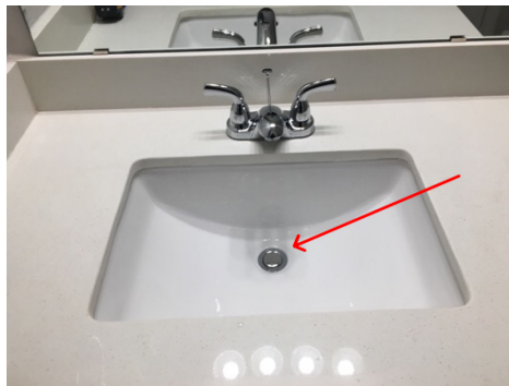
Bathroom 3: inoperable stopper
