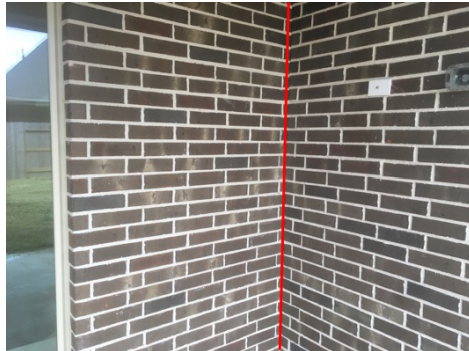
Rear: missing caulk at expansion joint
