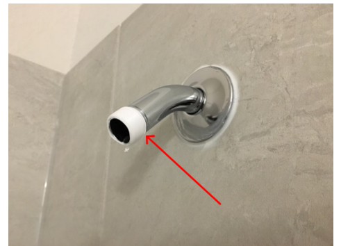
Bathroom 1: missing hardware
