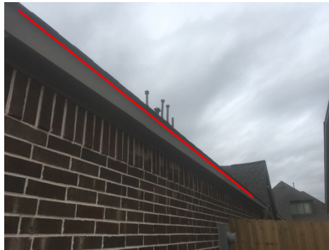
Incomplete gutter system
