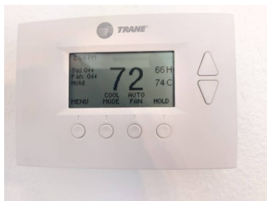
General Infrared Photos of HVAC Equipment:
