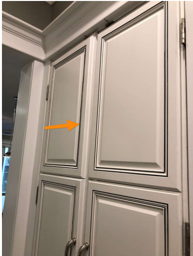
Doors hardware needs an adjustment.
