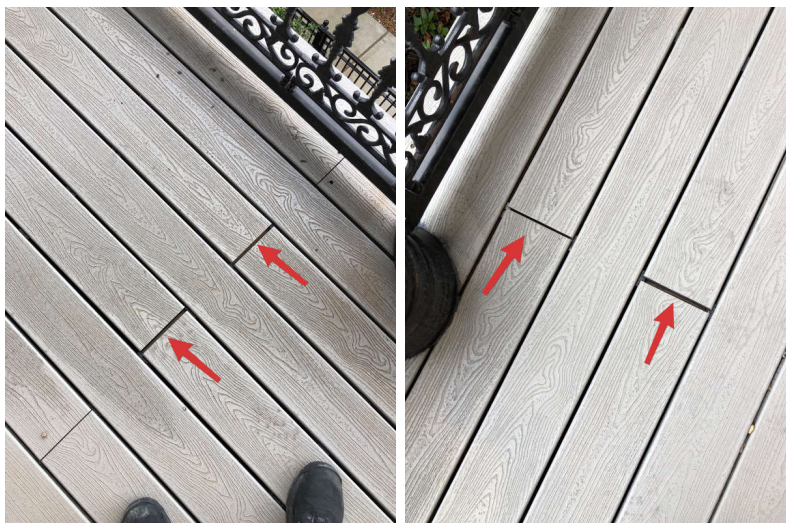
Fasteners are missing.
