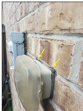
Right side, needs caulking improvements
