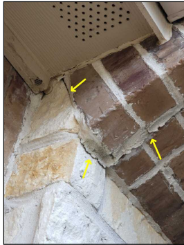
Front, needs mortar pointing
