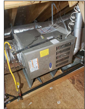
Furnace unit, gas shutoff valve, sediment trap and vent
