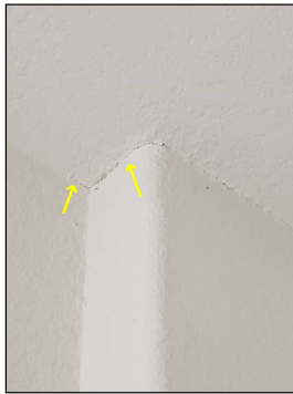
Hall bathroom, sheetrock cracks noted
