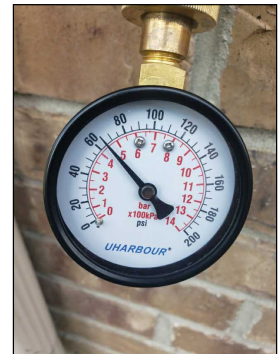
Static water pressure is approximately 65 psi
