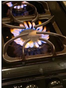
Orange flame on all burners noted and is the result of incomplete combustion and generation of carbon monoxide. Recommend further review by a appliance technician
