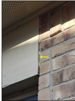
Right side, needs caulking improvements
