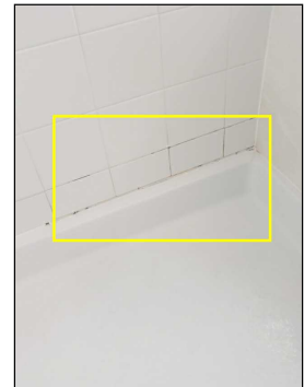
Primary bathroom shower, damaged grout noted
