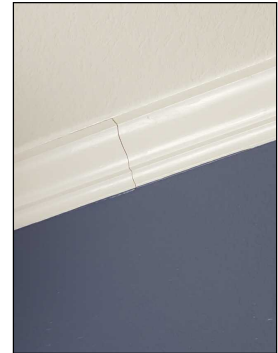
Primary bedroom, caulking cracks noted
