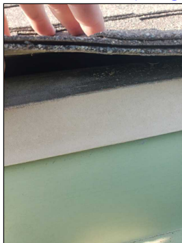
Underlayment not properly installed over drip edge
