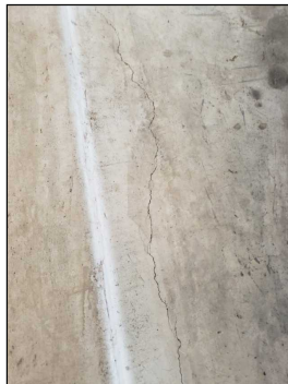
Minor cracks in garage floor noted
