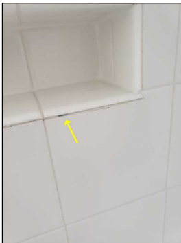
Hall bathroom, cracked or missing grout noted
