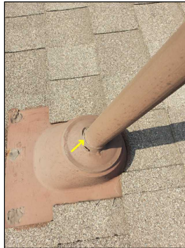
Recommend adding sealant to all plumbing vents at the boot/pipe interface
