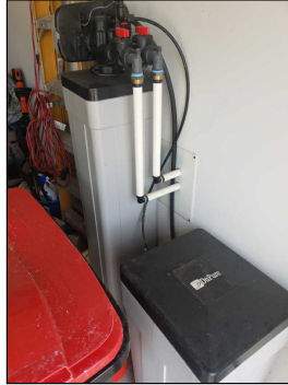
DuPure water softener. We do not inspect this item
