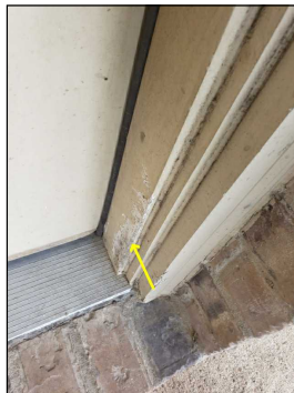
Back side, pet damage noted and needs paint
