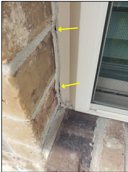
Back side, needs caulking improvements
