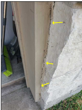
Front, needs caulking improvements REI 7-5 (05/4/2015)
