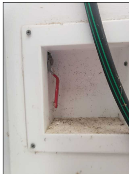
Garage, water supply shutoff valve
