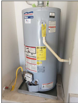
American 40 gallon gas water heater manufactured in 2015. TPR valve/drain , gas shutoff valve, sediment trap, heat controls, pan and pan drain
