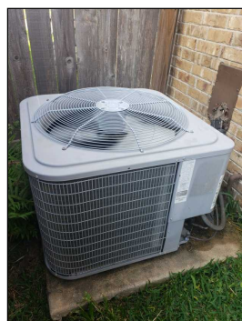
Carrier 3 ton condenser unit manufactured in 2015
