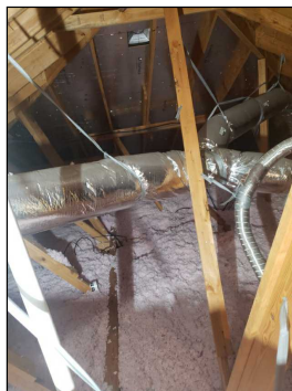
Ductwork was properly hung from roof structure and not touching each other
