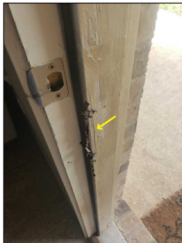
Back door, damaged weather stripping noted
