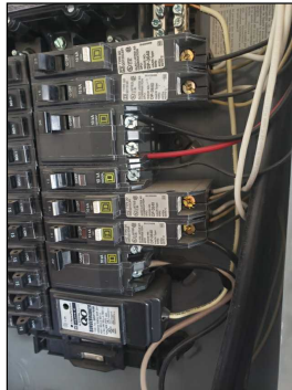
Right side breakers
