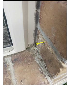
Right side, needs caulking improvements
