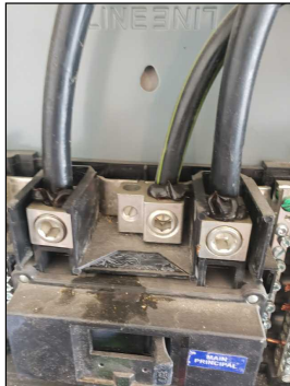
Aluminium service entrance conductors with anti-oxident grease
