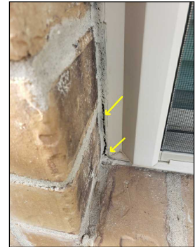
Back side, needs caulking improvements
