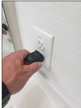
Primary bathroom, outlet is loose in wall and should be corrected
