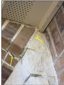
Front, needs mortar pointing
