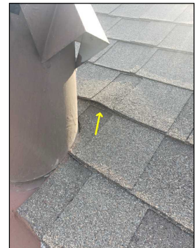
Nail pop noted
