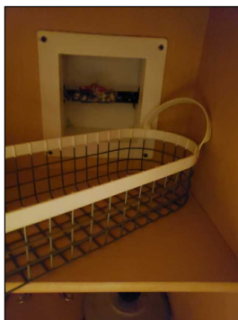
Gas shutoff valve in bottom left cabinet
