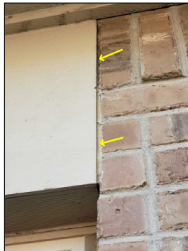
Left side, needs caulking improvements
