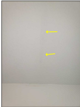
Primary bathroom, possible water stain noted
