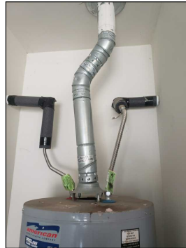
Water supply lines and vent
