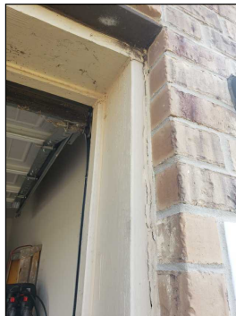
Front, needs caulking improvements
