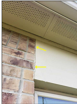
Back side, needs caulking improvements
