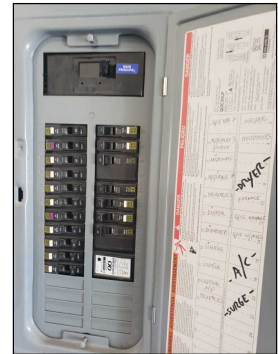
Square D 150 Amp service entrance panel, properly labeled
