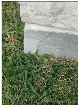
Front right, corner pop noted
