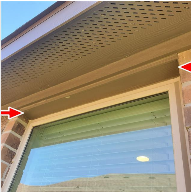
E. Item 2(Picture) This is a different window showing what is missing.
