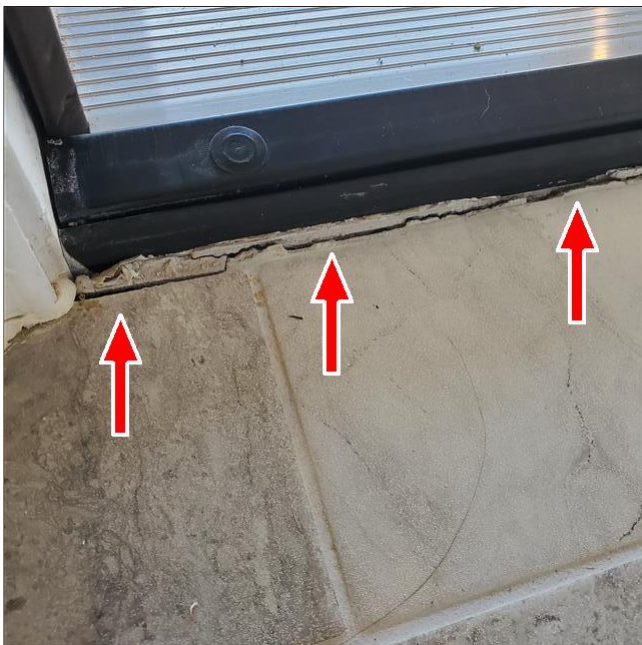
F. Item 1(Picture) Damage to flooring/grout at entry to garage.
