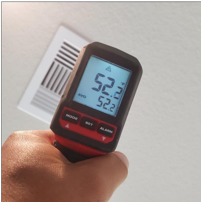
B. Item 2(Picture) 52 degree supply air.
