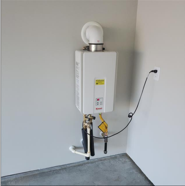
C. Item 1(Picture) Overview of water heater.
