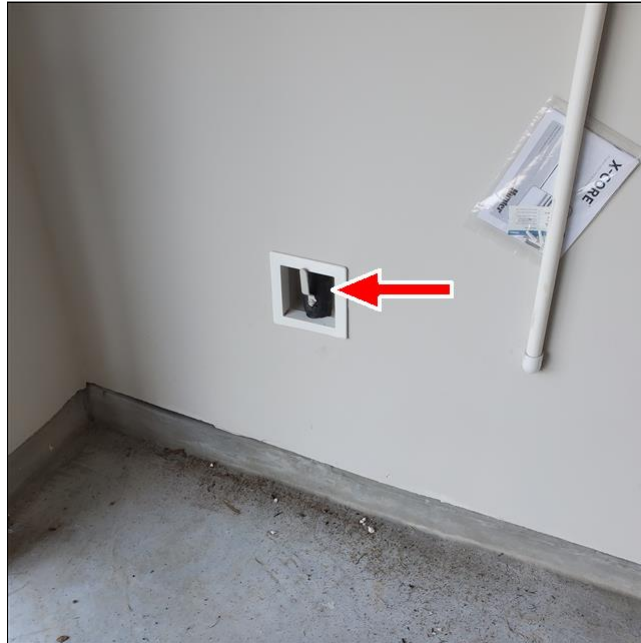
Main water valve in the garage.
