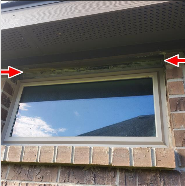
E. Item 1(Picture) Missing wood header here.
