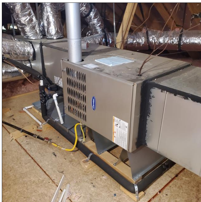
A. Item 1(Picture) Overview of heating system.
